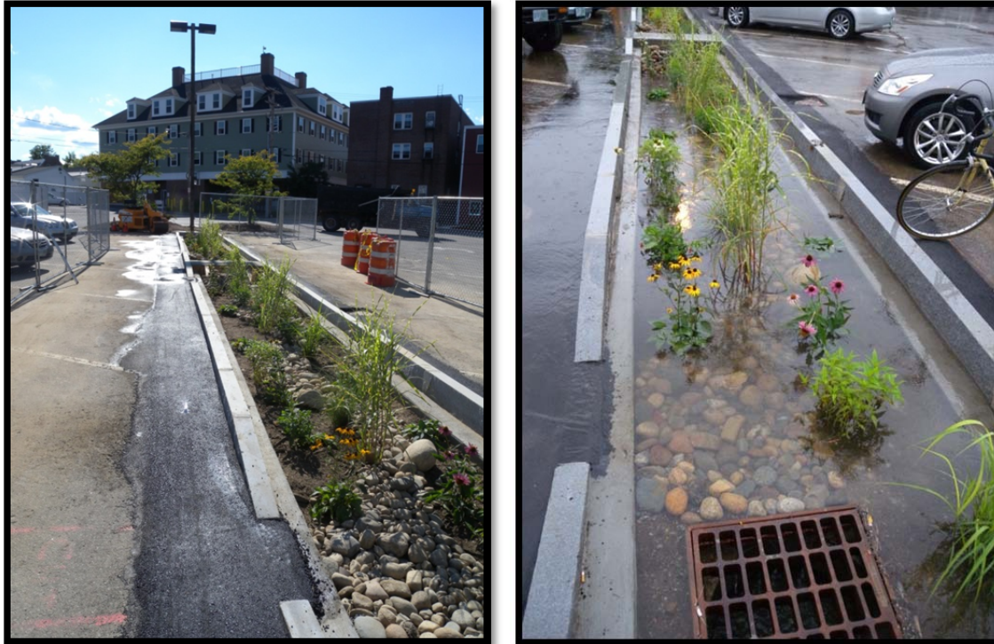
(a) (b) Figure 29. Bio-5 in Durham, NH immediately after completion (a) and during the first storm (b), Cell 2 in the foreground in each. Photos by Viktor Hlas.
