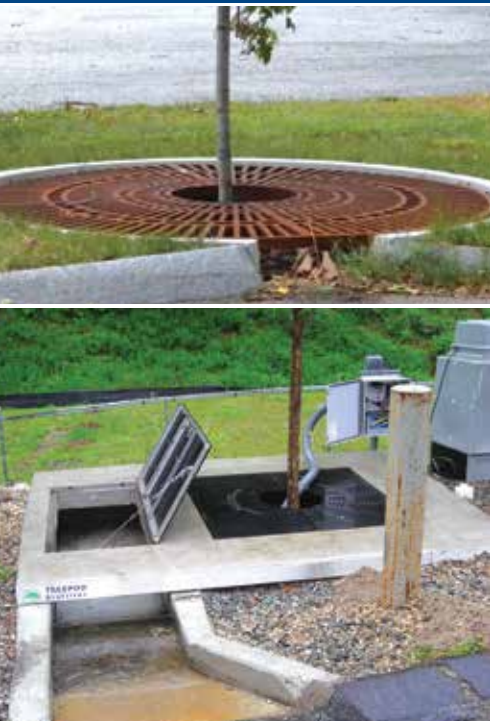
Though small, tree filters can manage runoff from the numerous lighter rain events that make up the majority of the annual rainfall in most regions. This makes them valuable assets in treating areas with large amounts of impervious cover.
