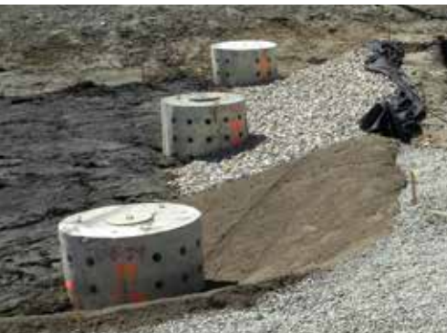
Subsurface gravel wetlands have demonstrated exceptional water quality treatment in a range of land uses, including commuter parking, high-density commercial development, and along major transportation corridors.
