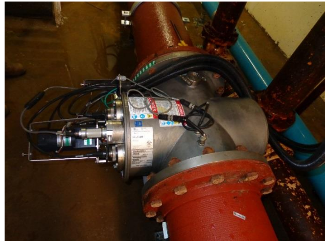
Figure 1a: This is a photo of the pilot UV disinfection system placed in Bethlehem. There are four UV lamps shown with black tops sticking out of the left side of the reactor. There are two UV wavelength sensors shown with longer gray columns connected to the black tops.
