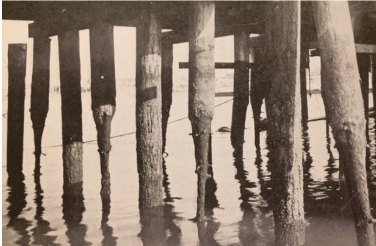
Figure 29: “Hourglass” Piles. The San Francisco Marine Piling Committee of the American Wood-Preservers’ Association, Inc. Final Report of the San Francisco Bay Marine Piling Committee , 27. Used with permission of the American Wood-Preservers Association.
