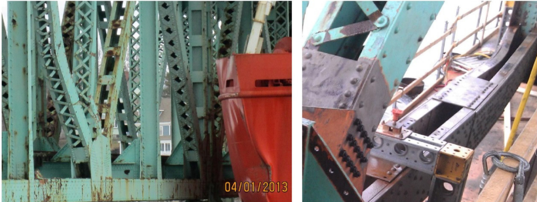
Figure 2 – Vertical Member Damage (left) and Lower Chord Damage (right)
