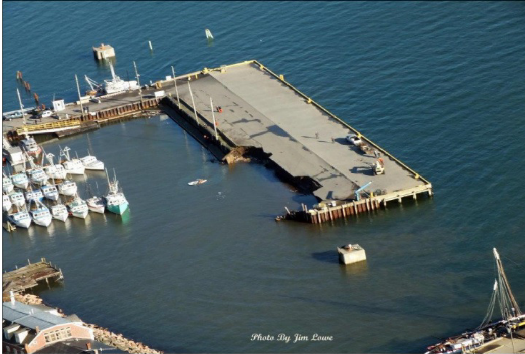
Figure 31 - Overview of Collapsed Eastport Breakwater
