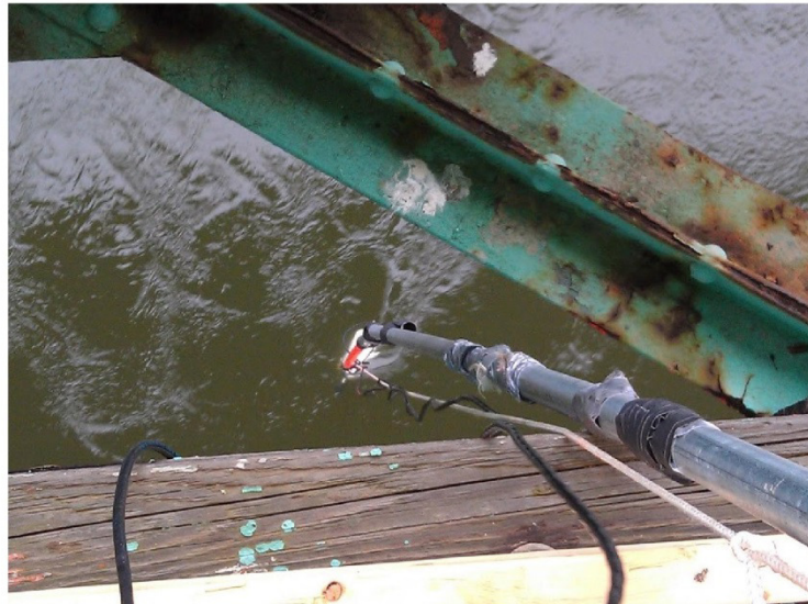
Figure 5 - Conduit Secured to Catwalk
