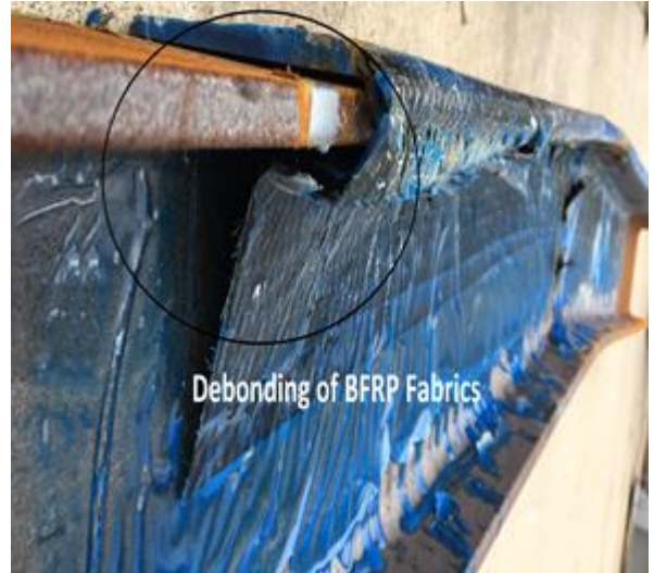
Figure 2.18: Photo showing the debonding for thick repairs
