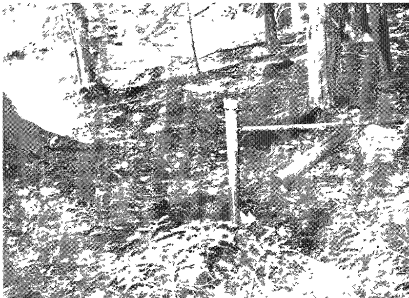
Figure 12: Example monitoring well installation. Well g4-1 installed immediately downstream of the catchment outlet at s4 approximately 5-m from Lamprey River (at left). Well extends 51.51-cm above grade and extends to 137-cm below grade.
