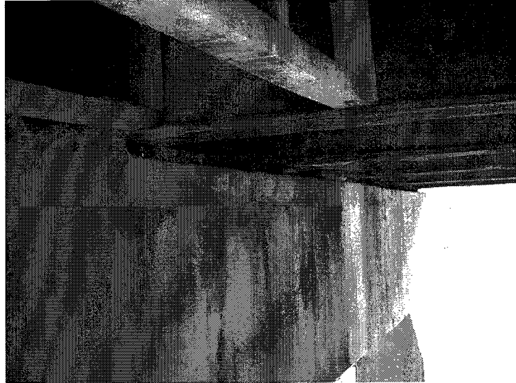
Photo 17: Pier Cap #1, south face; Rust stains exist below horizontal cracks.
