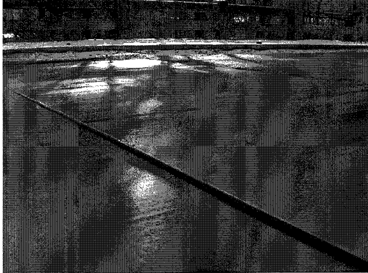
Photo 1: Connection welds are broken between steel plates. Plate #2 sags, creating a 1" lip between Plates #1 & #2.
