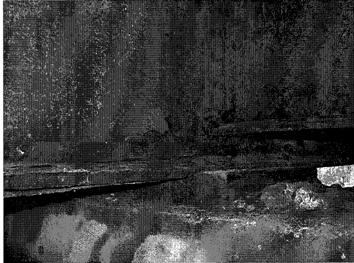
Photo 13: Span 1, Typical heavy corrosion of beam & bearing above Pier #1.
