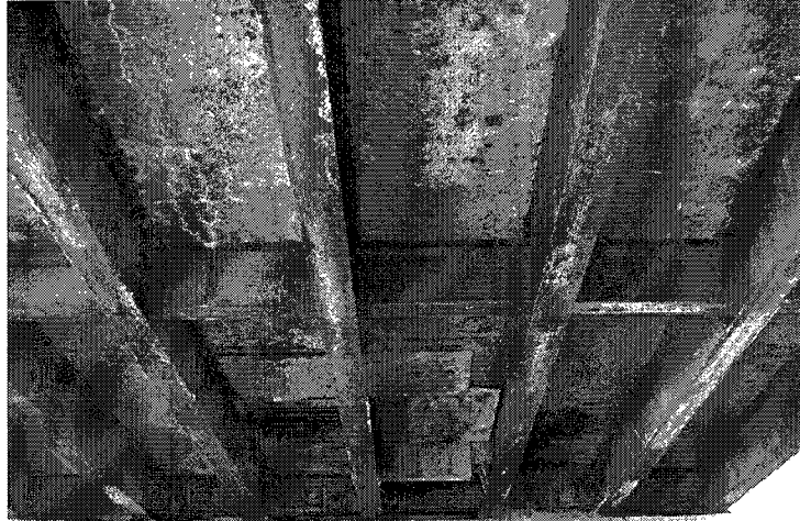
Photo 5: Span 2, looking south; Note the heavy cracking with efflorescence & severe spalls, some with timber repair forms.
