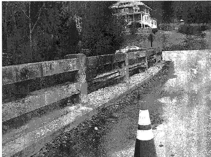
Photo 12: Heavy deterioration of concrete horizontals is typical for approximately 25% of the bridge rail system.
