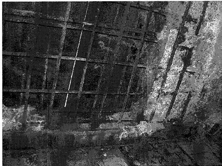
Photo 6: Span 2, Close-up of typical full depth spall adjacent to Pier #1.
