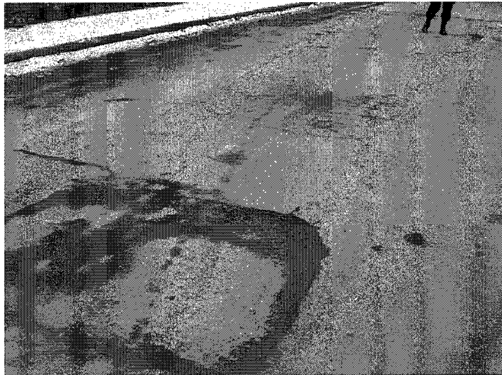
Photo 4: Wearing surface above Span 3 has areas of full depth repairs; Other areas are heavily cracked.
