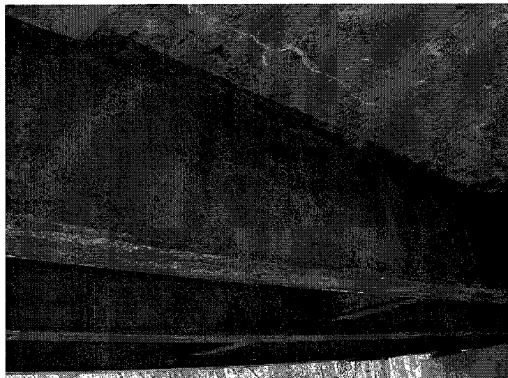
Photo 14: Span 2; Typical corrosion of beams.
