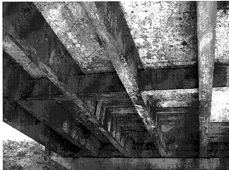
Photo 8: Span 3; Timber repair forms remain in place at north end of Bays #3, #4, & #5.
