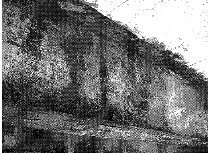
Photo 15: Span 3, Beam #4 near mid-span. Upper & lower flanges have layered rust with measurable section loss. Web has flaking rust.
