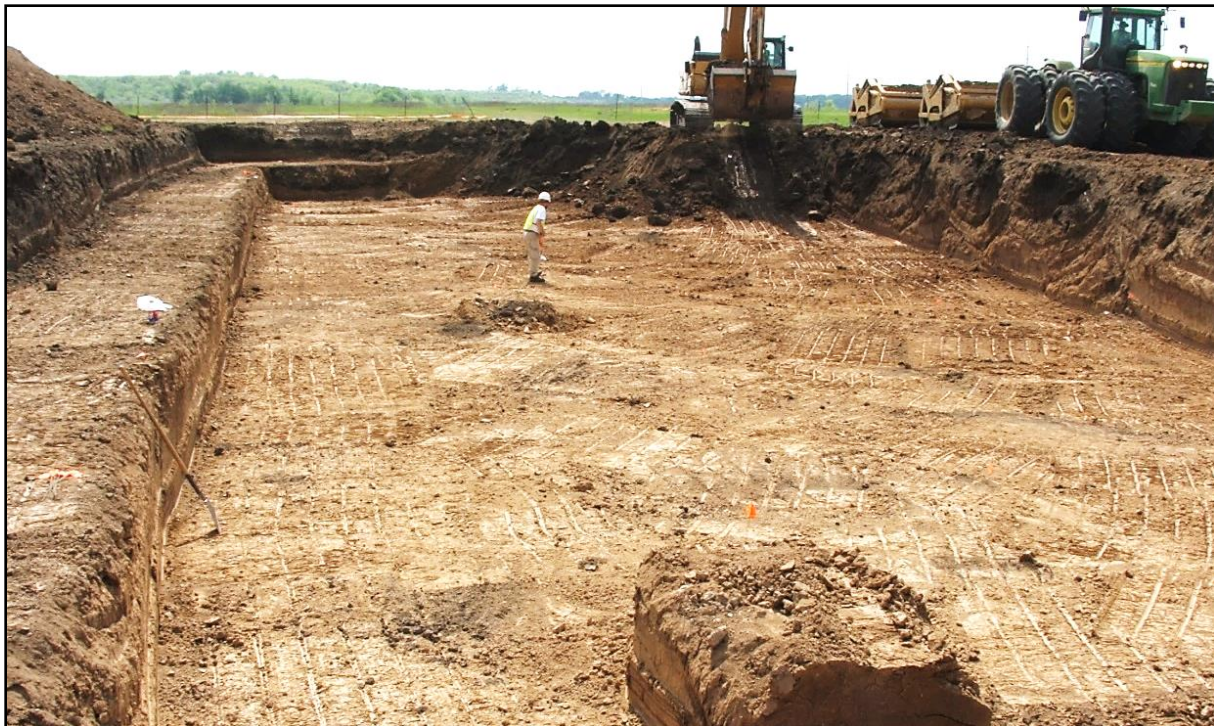
Figure 5-1. Southern view across mechanically stripped excavation block with track hoe and other earth removal equipment in background. Note safety bench on left side and pedestalled burned rock feature in foreground.
