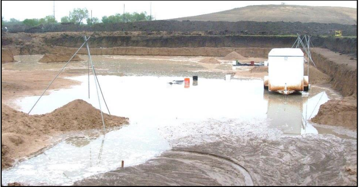
Figure 5-9. Northern view of flooded excavation area.
