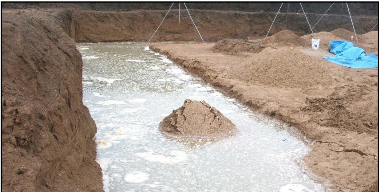
Figure 5-10. Western view of water filled trench along southern margin of excavation block.
