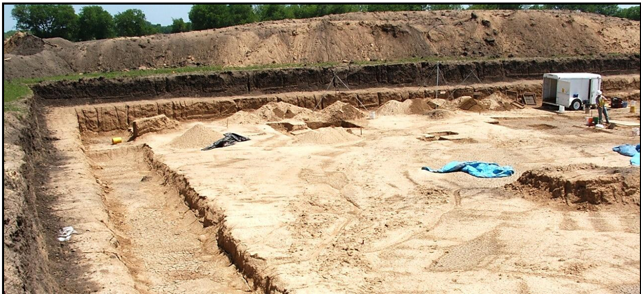
Figure 5-3. Northern end of excavation block showing safety bench and water collection trench. Note Block A is on far side and Block D on right.
