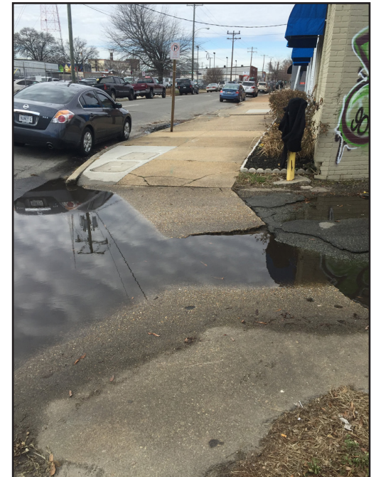
Figure 19: Poor Sidewalk Condition
