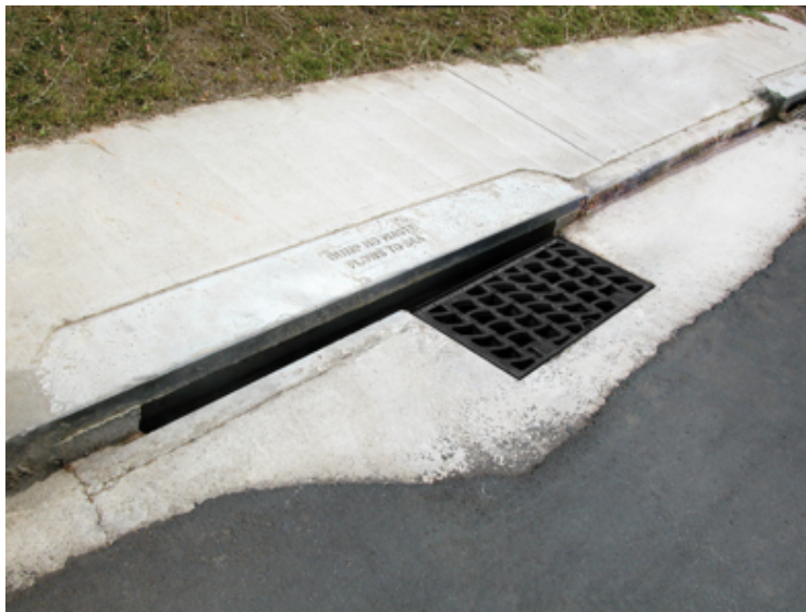
Image 15: Water Catchment in New Zealand (Source: http://www.hynds.co.nz/product-category/stormwater/stormwater-pits-kerb-blocks/ )
