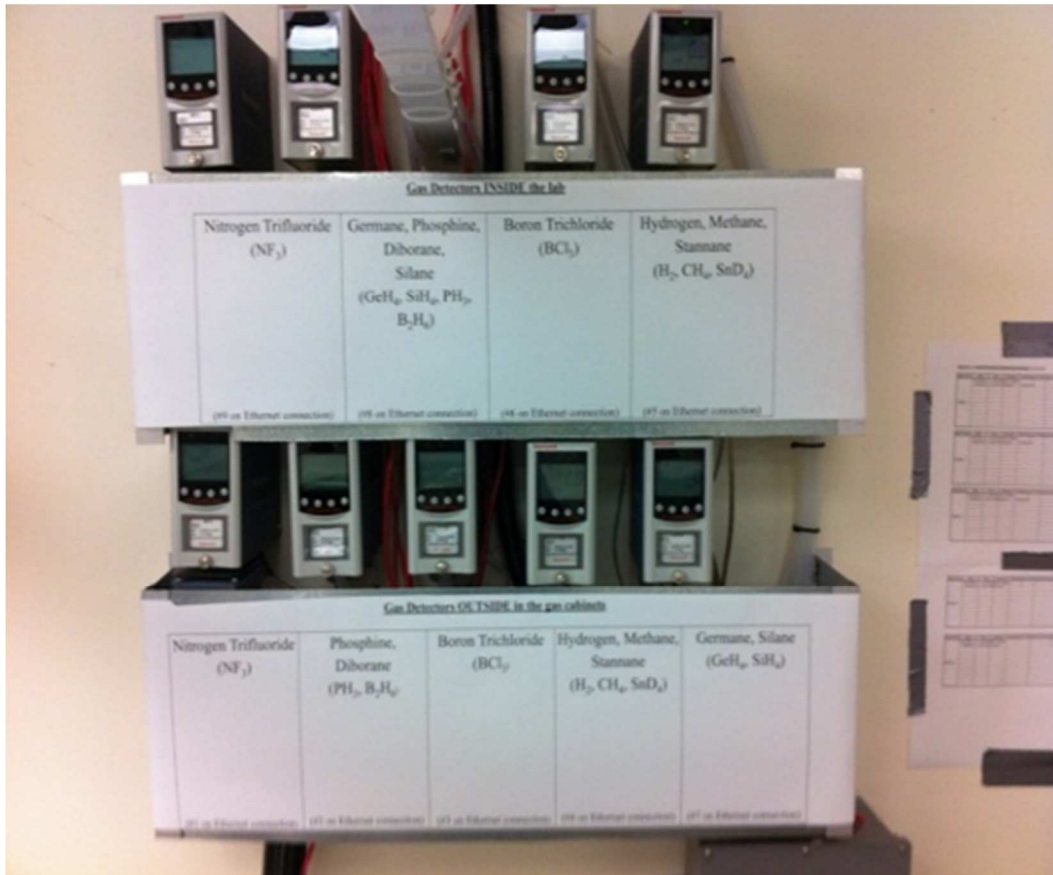
Figure 2.4: Image of toxic gas detection monitors installed in UHV-CVD lab.
