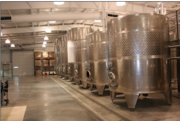
Figure 4. Modern wineries ferment in stainless steel tanks that are jacketed so that glycol circulation can be used to control temperature. (Photo courtesy of Prospero Equipment Corp.)
