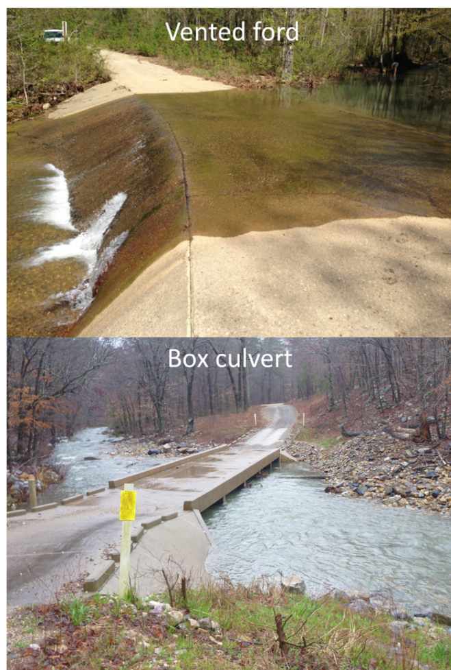
Figure 2. Water moves from right to left in both photographs of the 2 culverted streams. At the clogged vented ford on intermittent Bear Creek, water pooled upstream and flowed over the concrete slab. The turbulent water in the left foreground indicates the 2 culvert outlets. At the box culvert on perennial Long Creek, water flowed easily through the road crossing, even during summer low-flow conditions.
