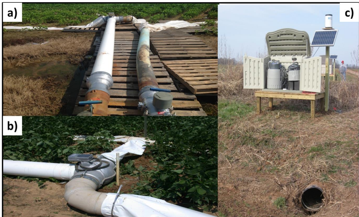
Fig. 2. Irrigation flow meters (a), surge (b) and automated runoff monitoring station utilized to measure irrigation flow, automatic distribution of flow and tail water loss from irrigation.
