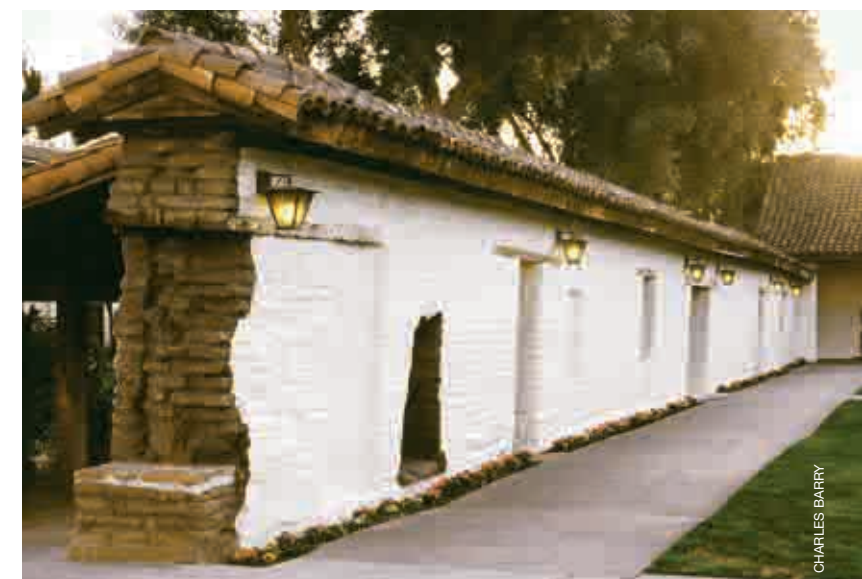
Brick and mortar: and a place some pause and pray—the Adobe Wall
