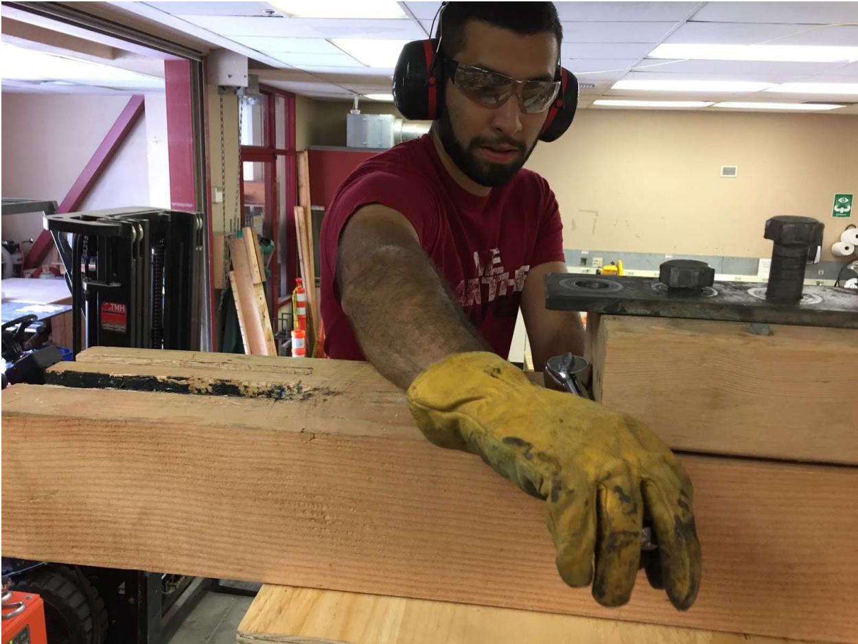
Installation of Nut + Washer for Bond Beam to Top Course connection at Top of Wall 2.
