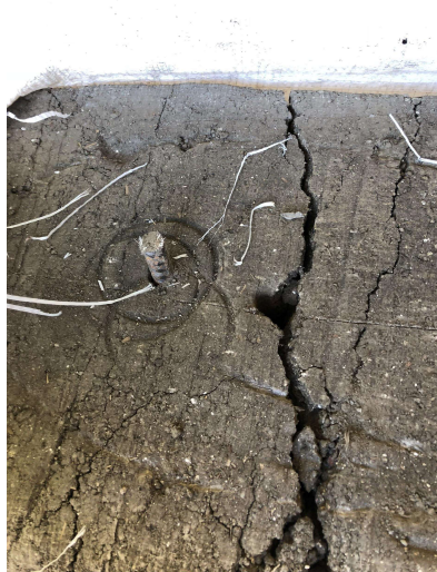
Figure 21: State of soil around rebar lap splice, Wall 1.
