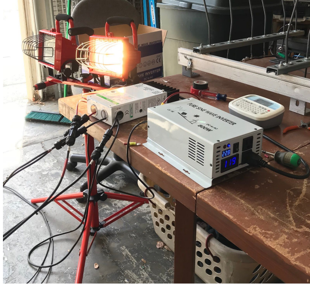
Figure 9: Overall setup with the 24V 800W inverter, powering a flood light
