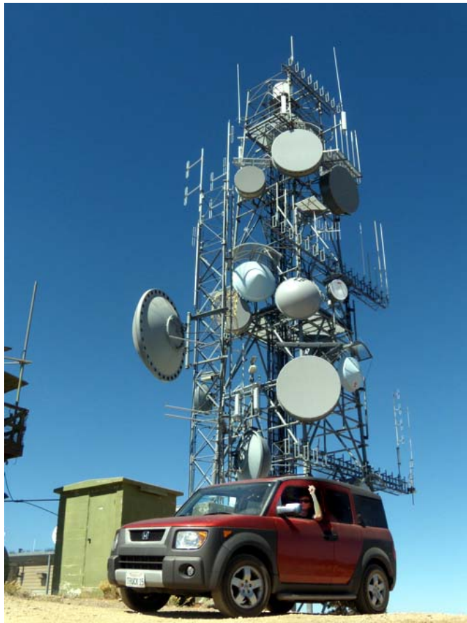
Fig. 1. Tower with several microwave antennas. 1
