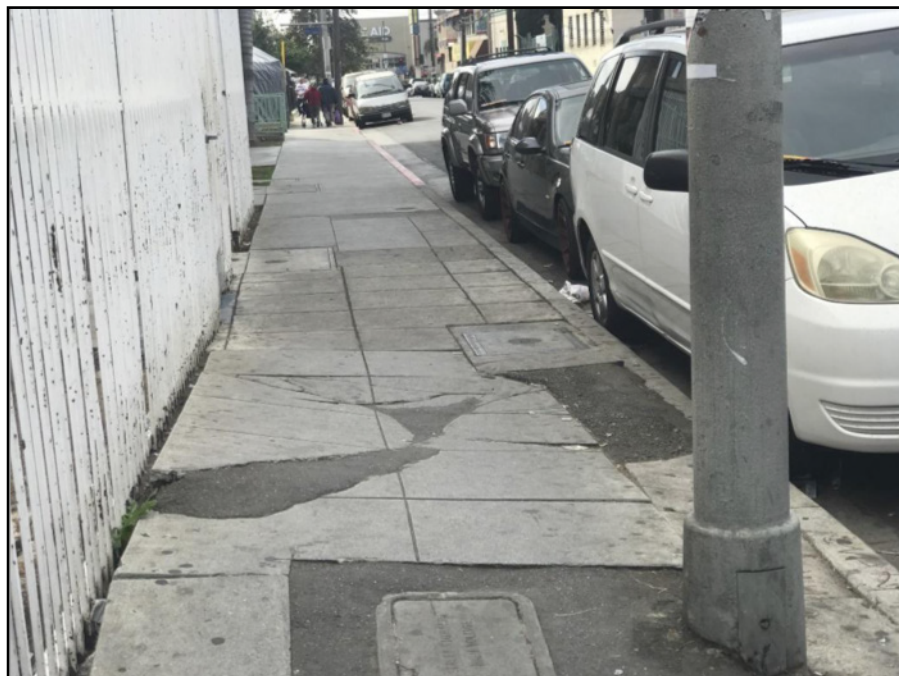
Figure 27. Cracks and Uneven Pavement on Walking Route
