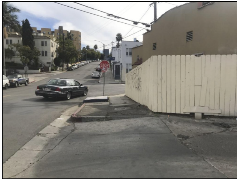
Figure 26. Cracks and Uneven Pavement
