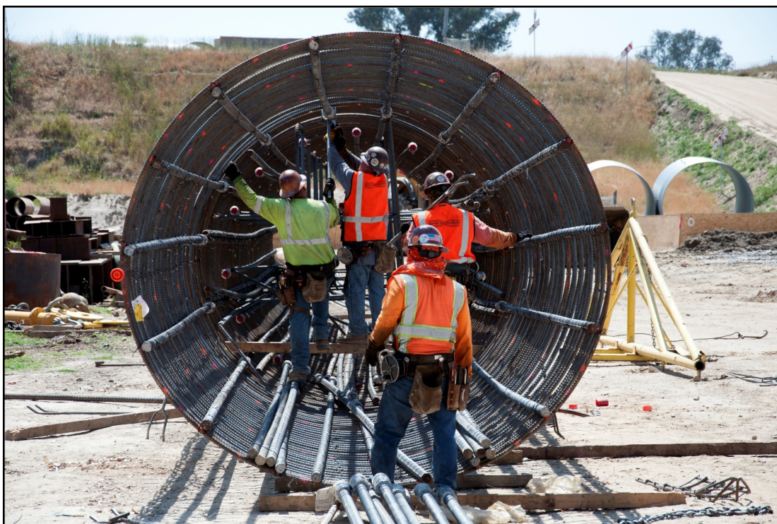
Figure 18. Steel Frame That Will be Part of a Poured Concrete Pillar for the San Joaquin River Viaduct
