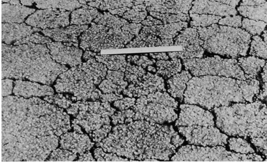
Figure 5 AC Bottom-Up Cracking taken from (ASTM-D6433-07)
