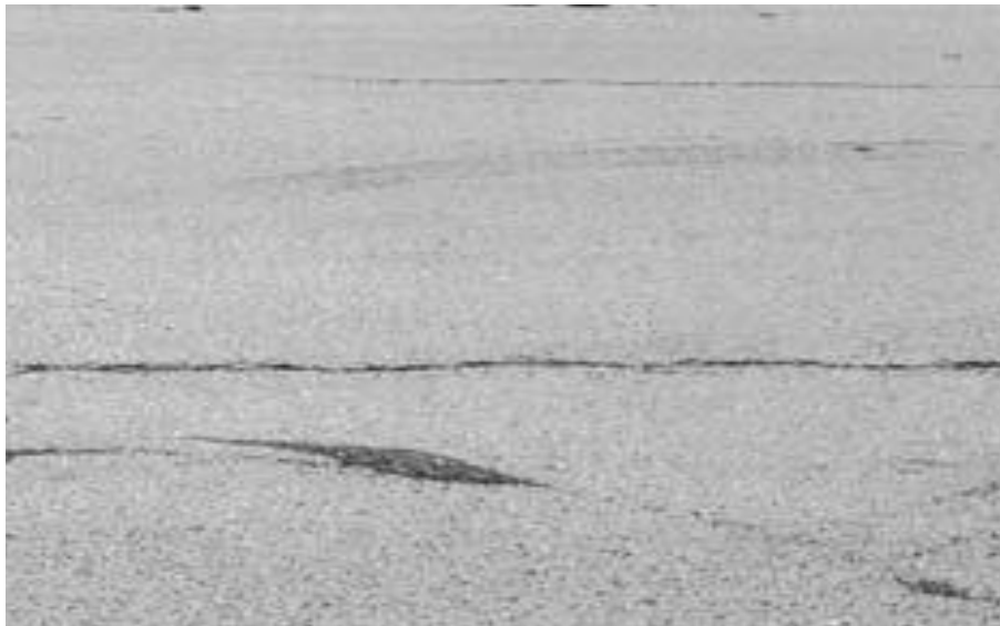
Figure 7 AC Top-Down Fatigue Cracking taken from (ASTM-D6433-07)
