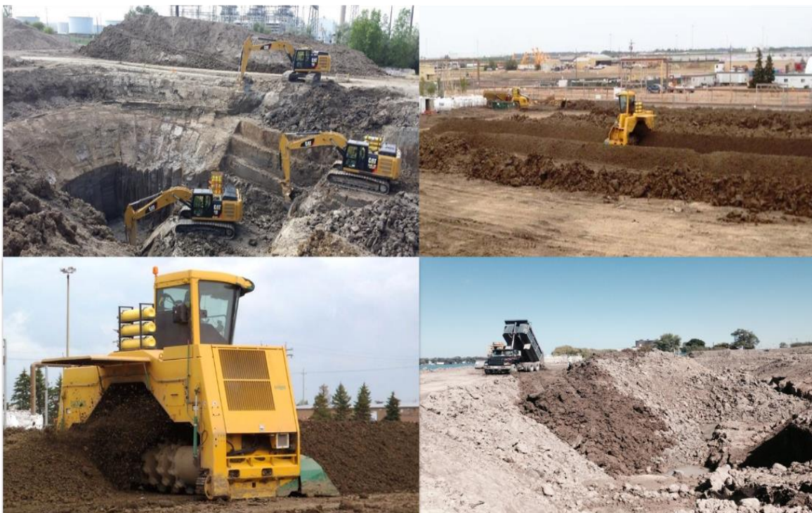
Figure 3.2 Pictures of the of the remediation process used to treat chlorinated solvent impacted soil ex-situ. The impacted soil is excavated (top left), then the amendment is mixed into the soil (top right and bottom left) before being backfilled to its original location (bottom right).
