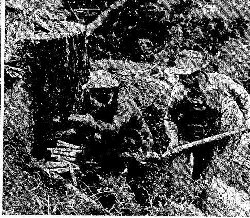
IMPROVING SKI BOWL: The Milwaukee Road is busy making improvements at its Ski Bowl. Above, Peter Birchall, section foreman, in charge of blasting, and Arthur Raymond (with shovel) place dynamite to blast a stump. Most stumps need 15 sticks of dynamite, but larger ones require a double dose. Small stumps are scooped out by a bulldozer without blasting.
