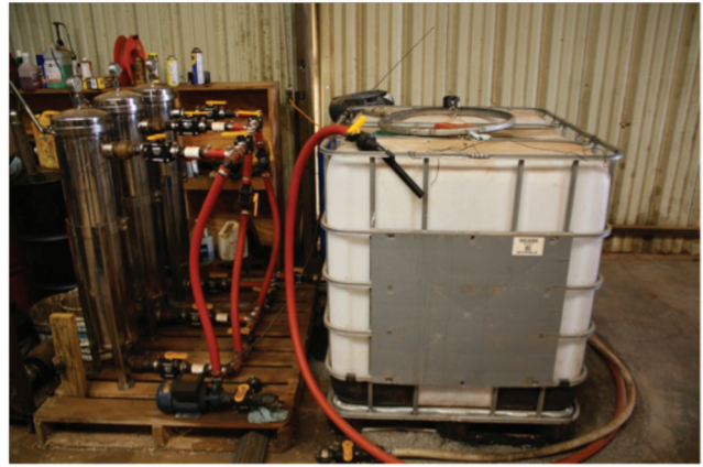
Figure 2: On-farm biodiesel filtration system.
