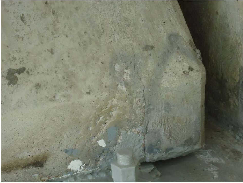
Figure 184. Crack at girder and diaphragm intersection (1S-W)
