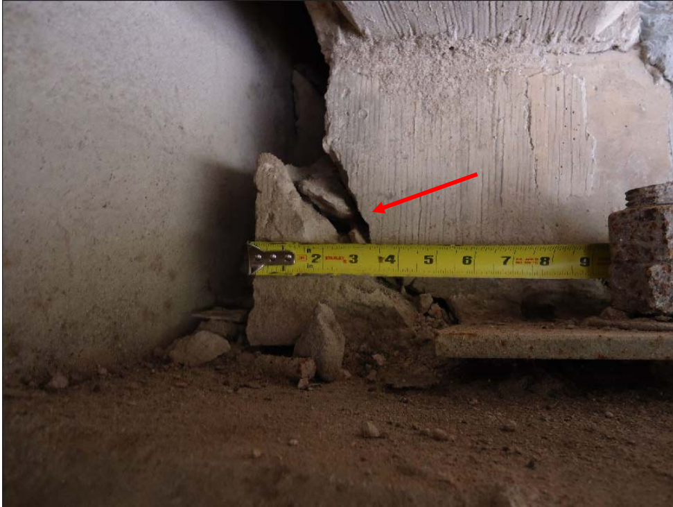
Figure 96. Example of back diagonal cracking
