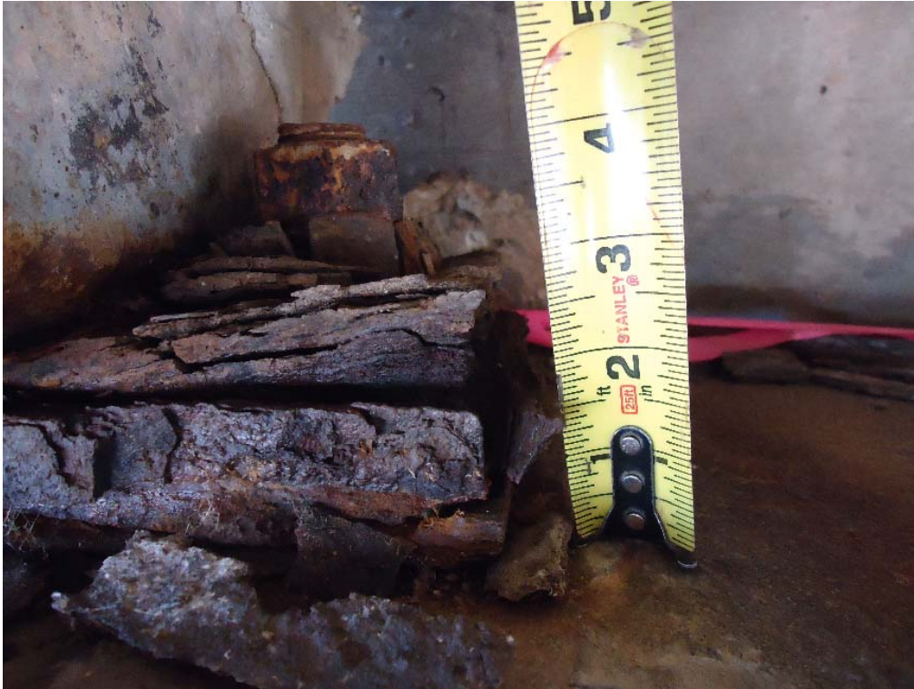
Figure 172. Corroded, flaky bearing plate
