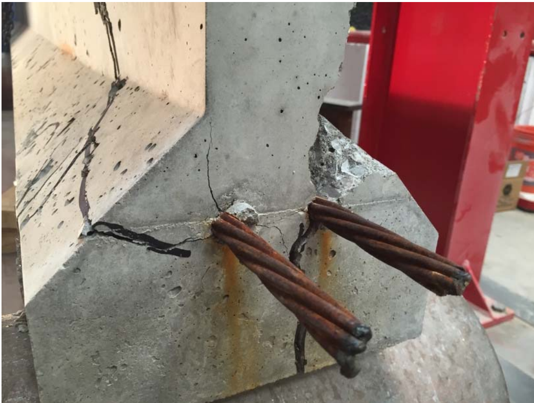
Figure 78. Cracking near prestressing strands
