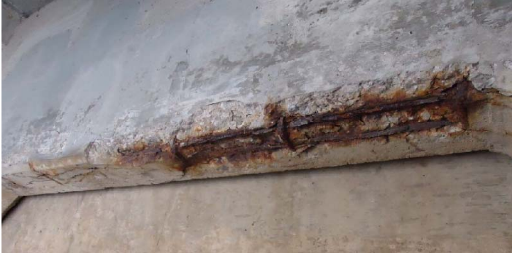
Figure 102. Example of Diaphragm deterioration
