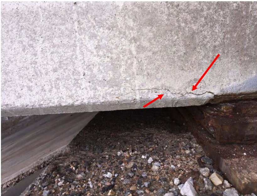
Figure 138. Cracking from corroded bearing plate into bottom flange (10S-W)
