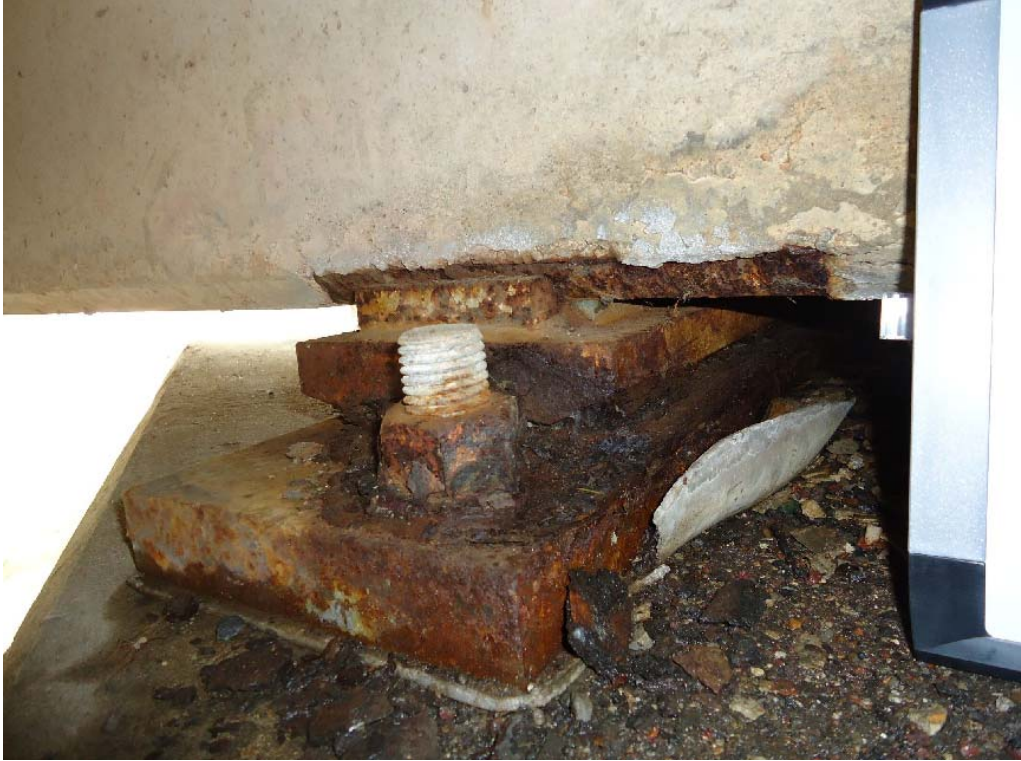
Figure 131. Corroded bearing plate (1E-S)
