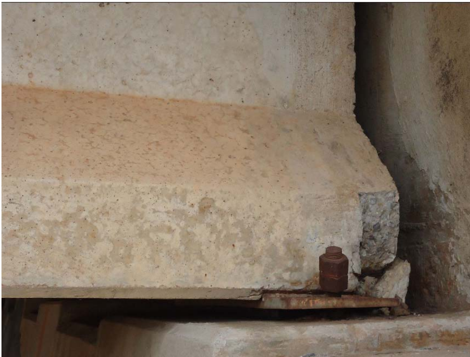
Figure 159. Back corner spalling of girder (9E-S)
