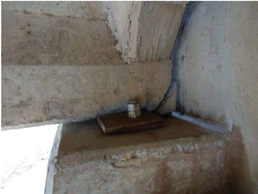
Figure 160. Back corner diagonal cracking of exterior beam (1E-S)
