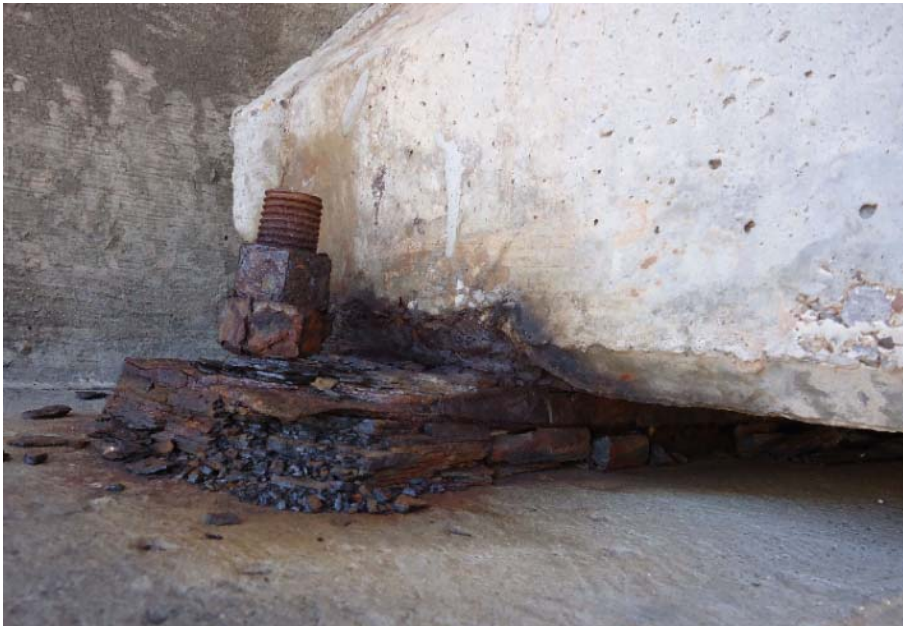
Figure 169. Corroded bearing plate, bolt, and nut along with spalling above the support of an exposed, exterior girder (1E-N)
