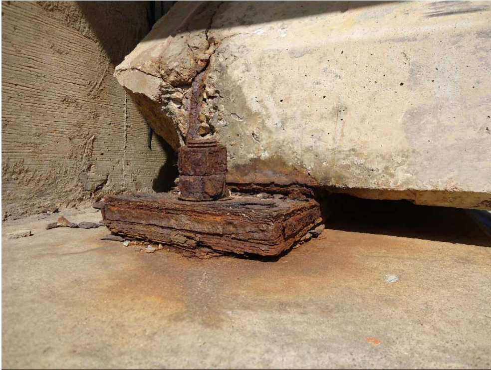
Figure 178. Corroded bearing plate, exposed rebar, and spalled back corner of girder (5W-S)
