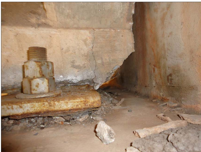
Figure 161. Similar back corner cracking (deformation) (2E-S)
