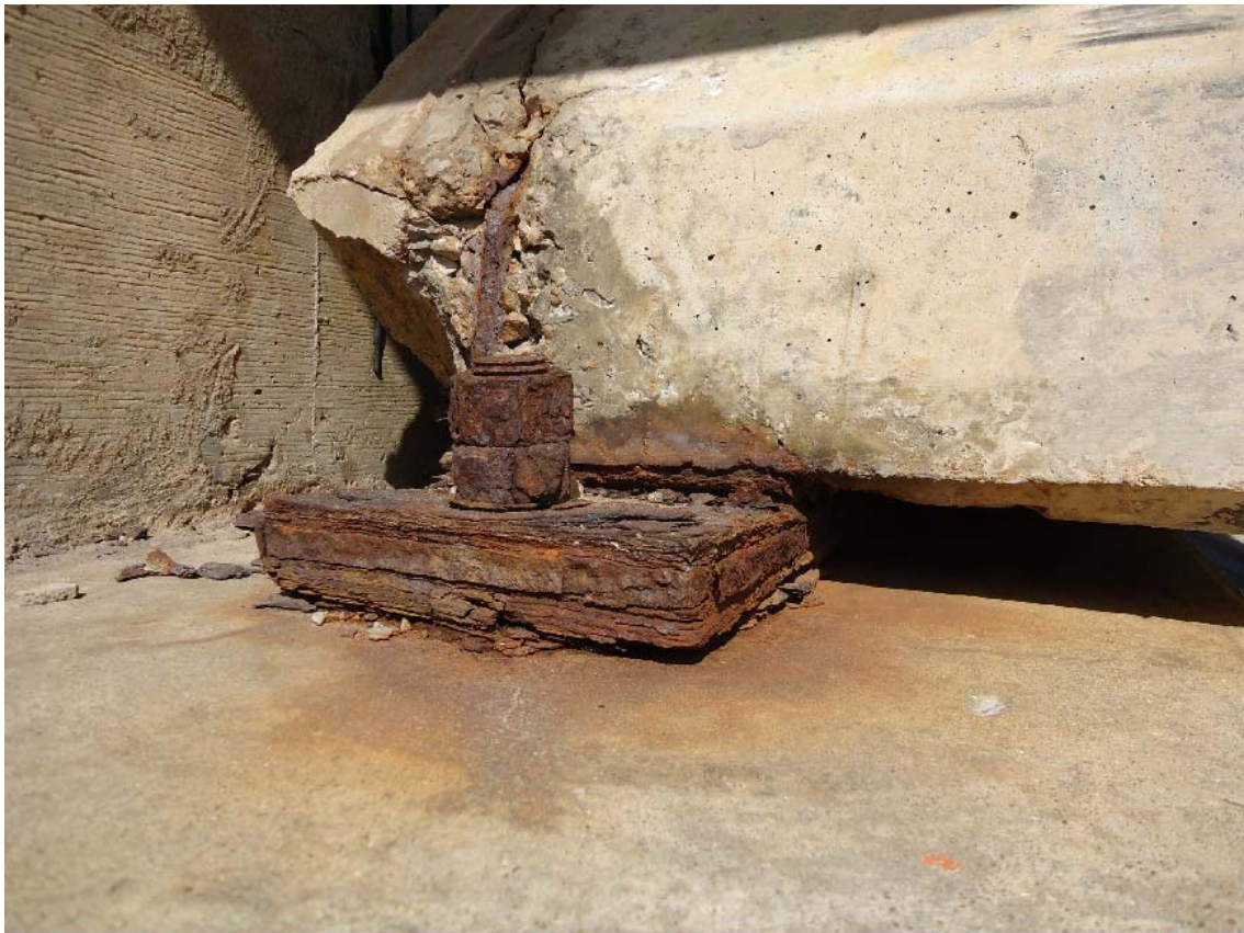
Figure 88. Example of corroded bearing plate
