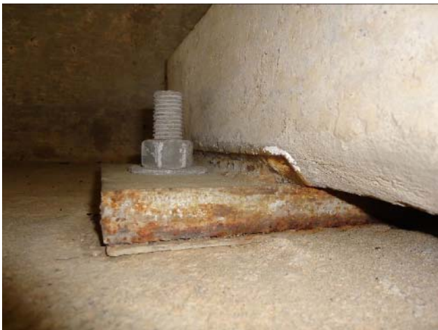
Figure 109. Another example of a corroding bearing plate (3W-S)
