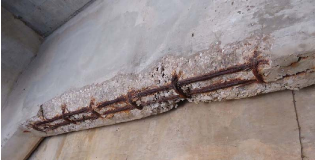
Figure 194. Similar corrosive underside of diaphragm, with exposed rebar cage
