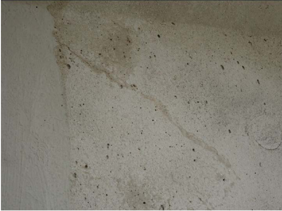
Figure 152. Diagonal crack in web from top flange towards bottom of beam (1N-W)
