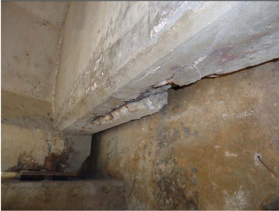
Figure 124. Deterioration of an interior diaphragm (6W-N); the diaphragm connects two interior beam ends
