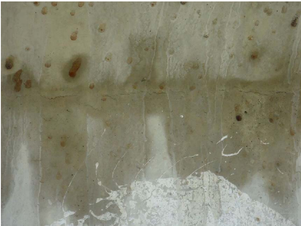
Figure 181. Horizontal crack at top flange and web interface for about one foot into the beam (5S-E)
