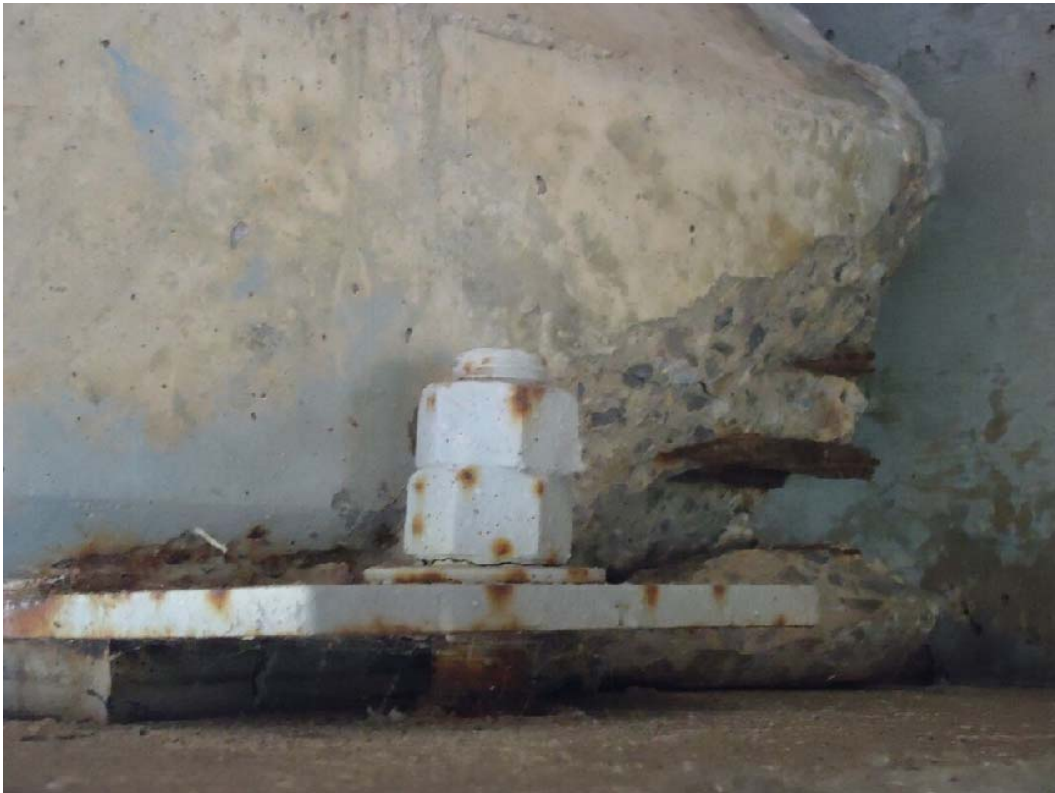
Figure 146. Exposed prestressing strands (10W-N)
