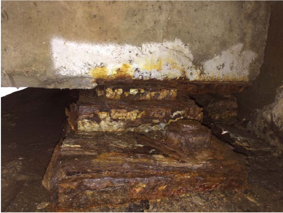
Figure 137. Corroded, and deteriorated bearing plate (8N-E)
