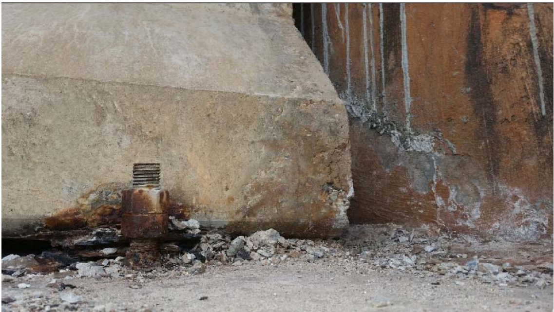
Figure 142. Corroded anchor bolt and spalling along bottom of girder and girder end (5N-E)
