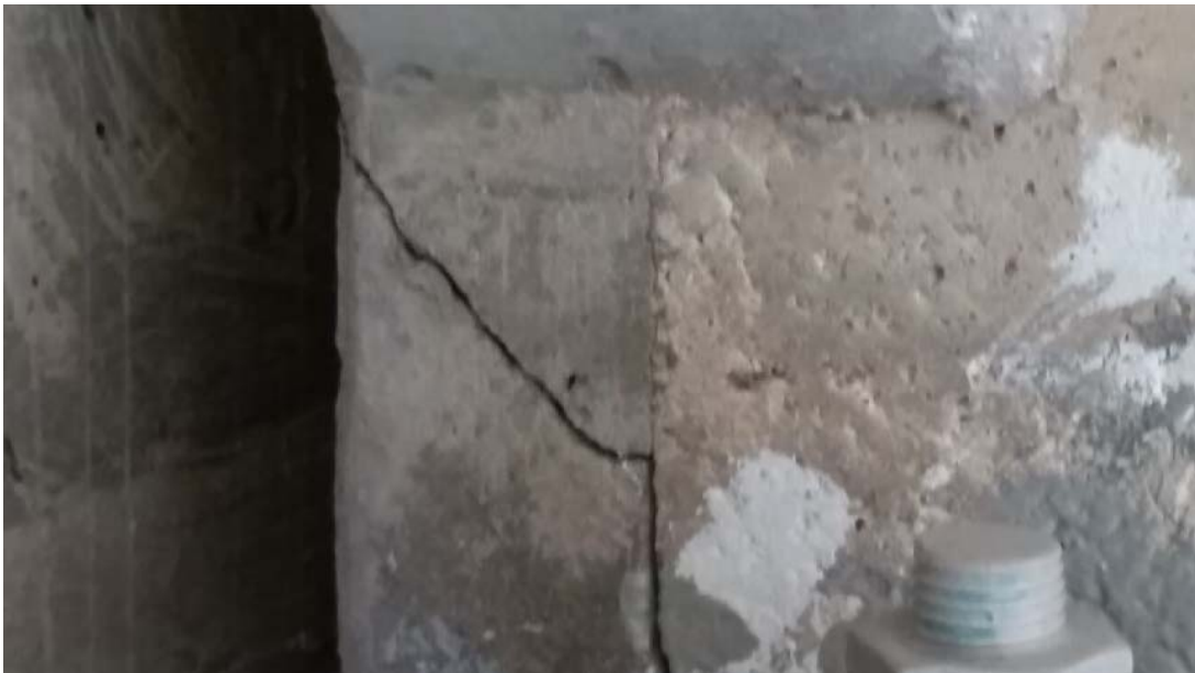
Figure 185. Back diagonal and vertical crack in girder end (2N-W)
