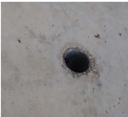
Figure 125. Spalling around pipe interface with exterior of concrete girder (3E-N)
