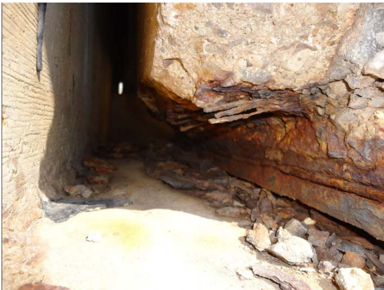
Figure 177. Diagonal back corner spalling and exposed prestressing strands (5W-S)
