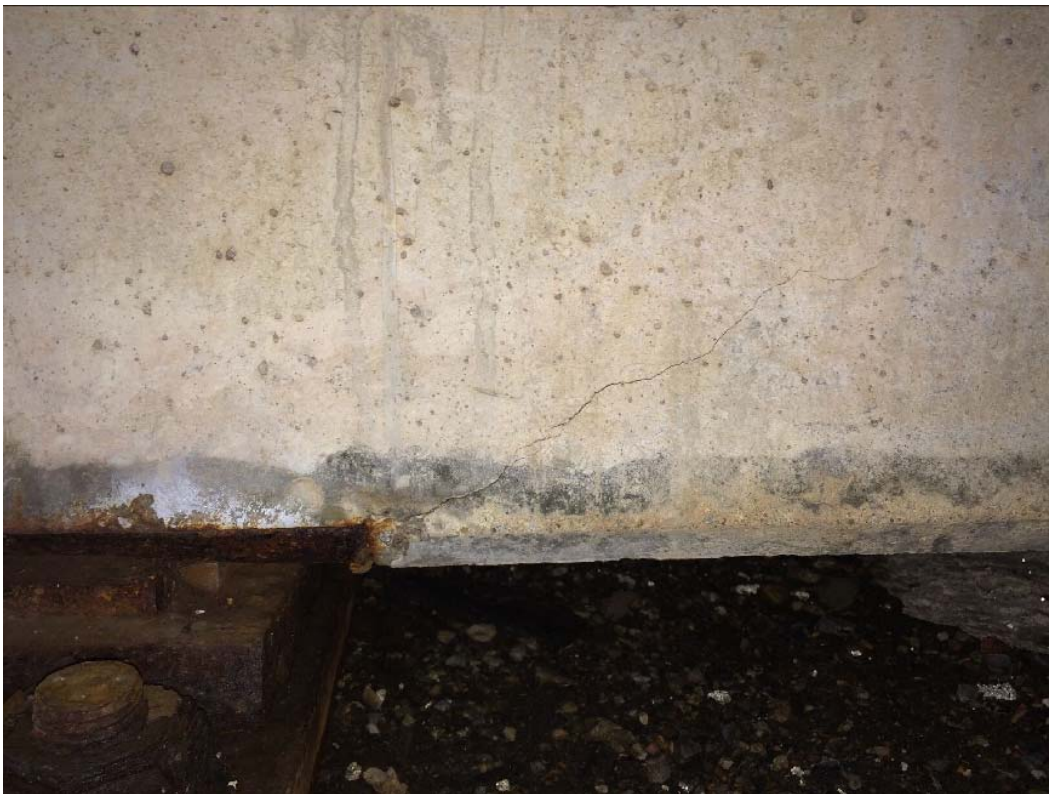
Figure 132. Diagonal crack in bottom flange of beam from corroding support (10W-N)
