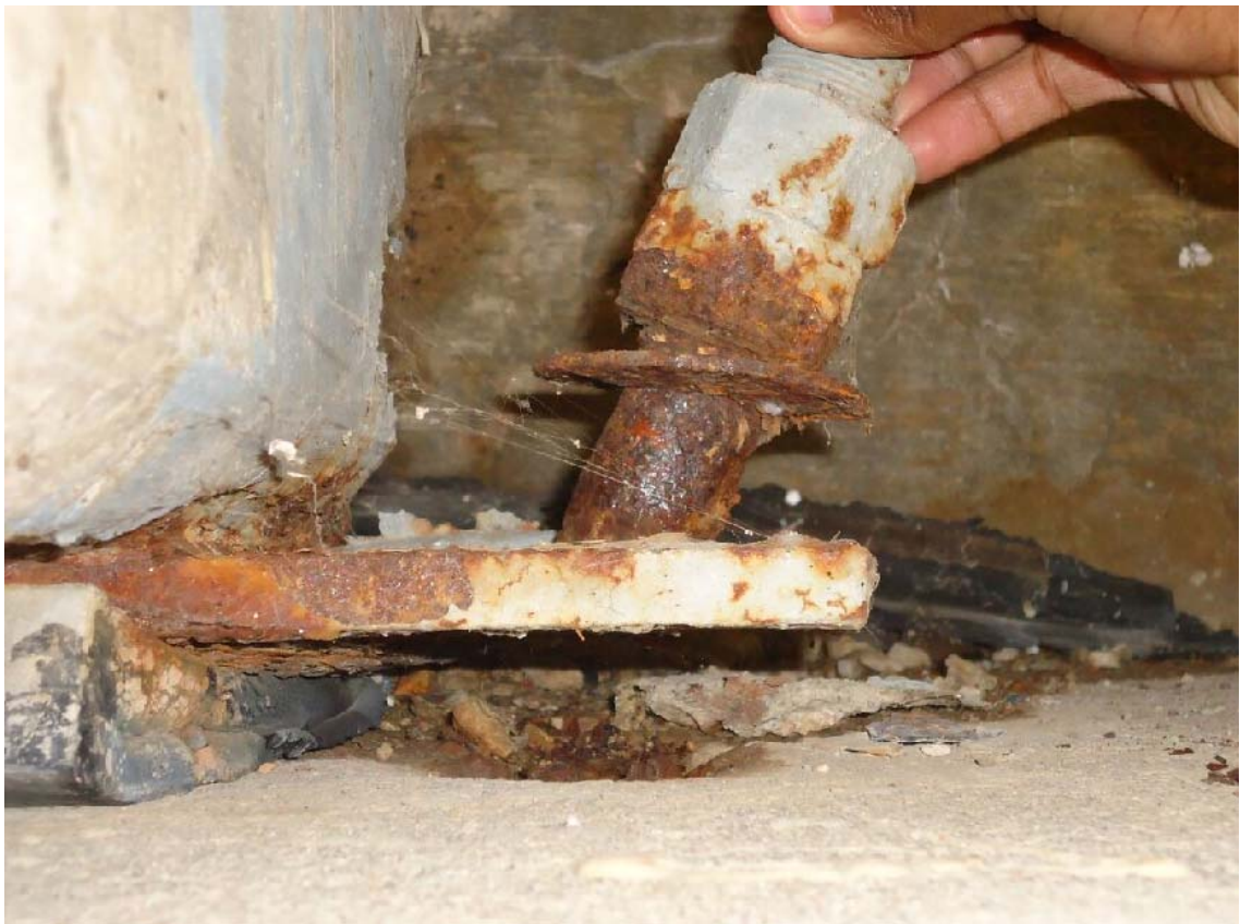
Figure 89. Example of corroded anchor bolt
