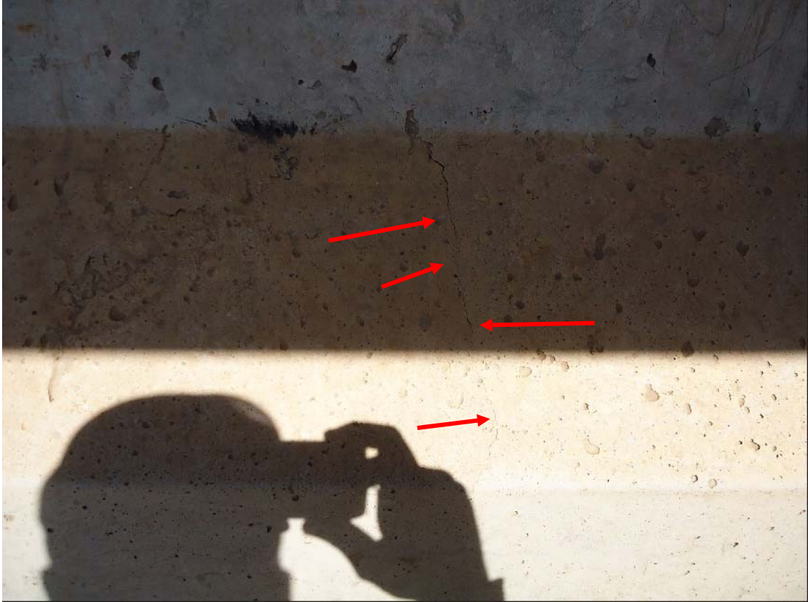
Figure 176. Crack along the web of girder (5E-S)
