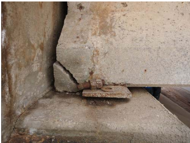
Figure 157. Back corner diagonal crack of exposed, exterior beam (1E-N)
