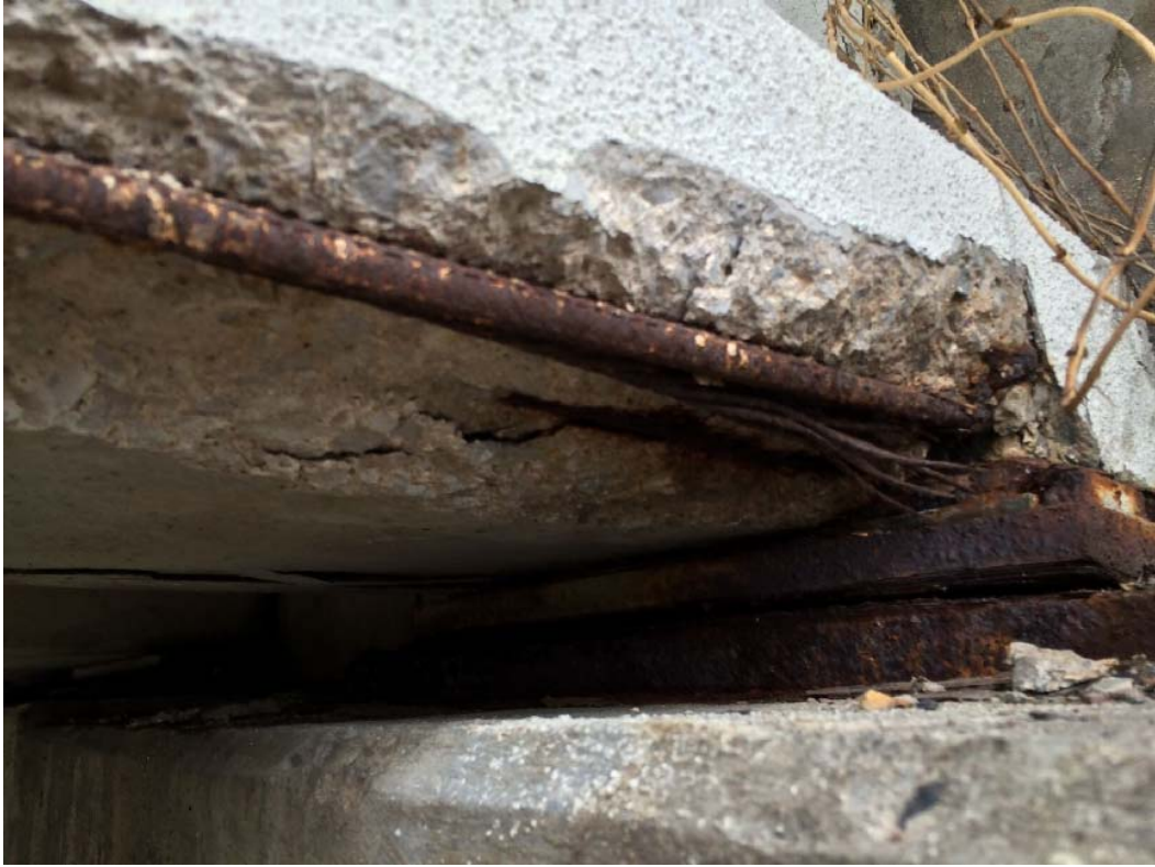
Figure 93. Example of exposed steel
