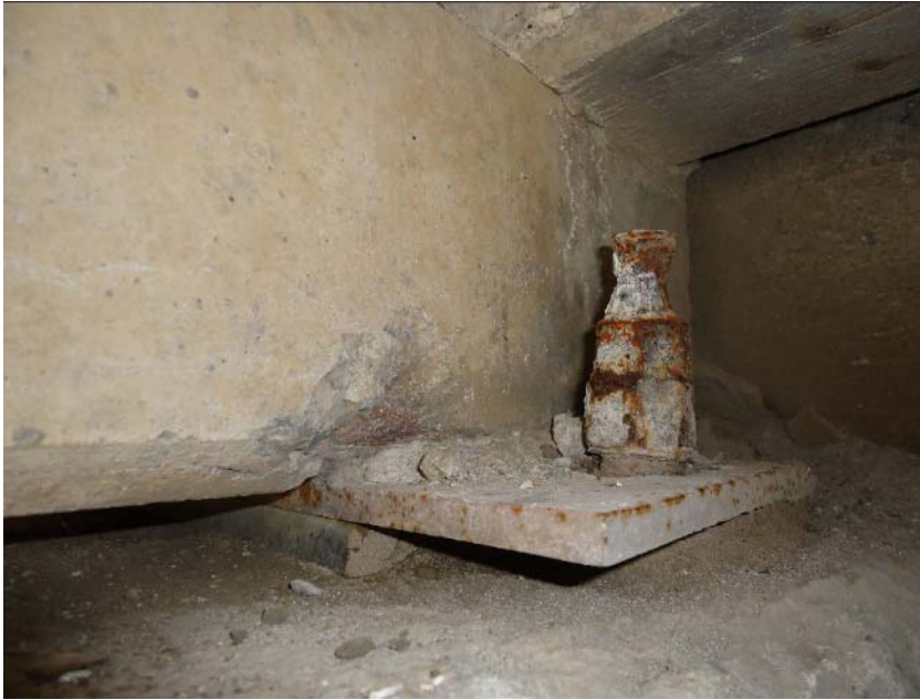
Figure 126. Anchor bolt with extreme deterioration, with necking of the anchor bolt at the top (4E-S)
