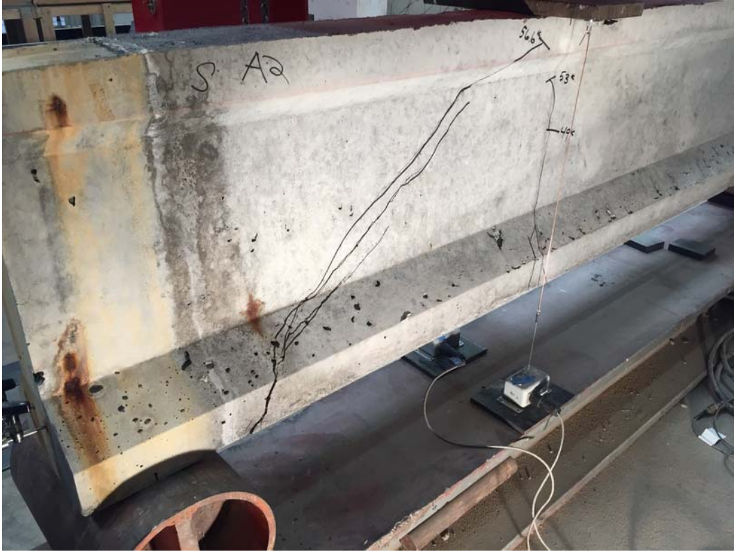
Figure 71. Visual map of cracking of A2SC
