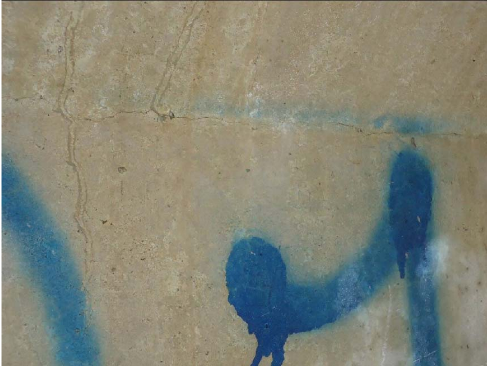
Figure 180. Horizontal crack at top flange and web interface for about one foot into the beam (1S-E)
