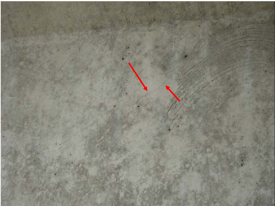
Figure 116. Diagonal cracking on the web of the beam, heading towards the bottom flange (1S-W)
