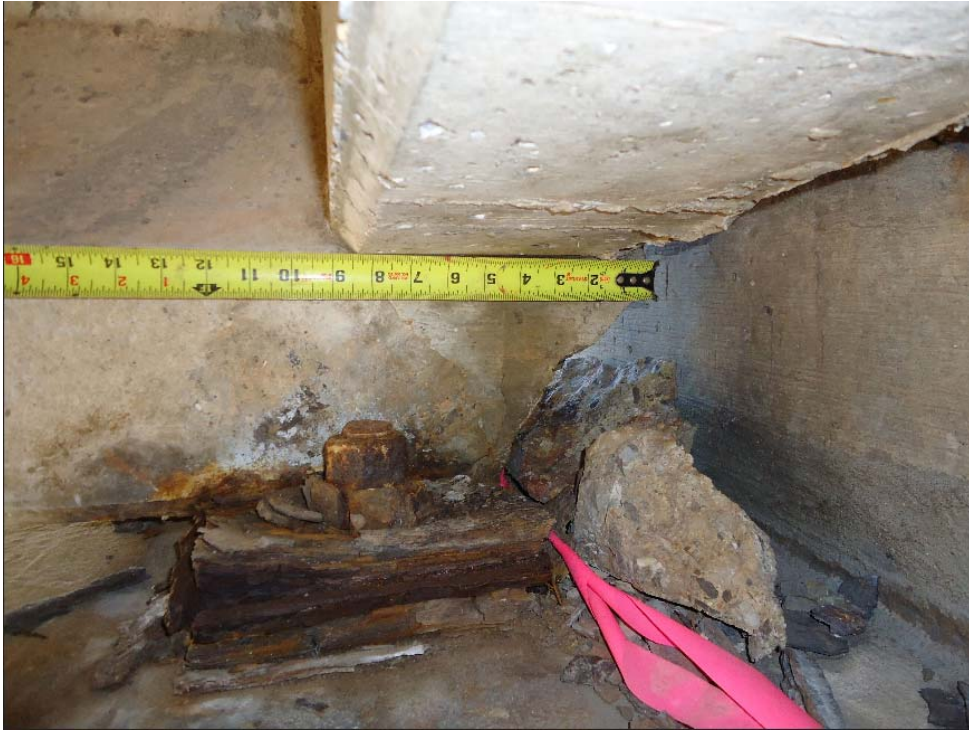
Figure 170. Corroded bearing plate and diagonal back corner crack with a maximum width of approx. four inches
