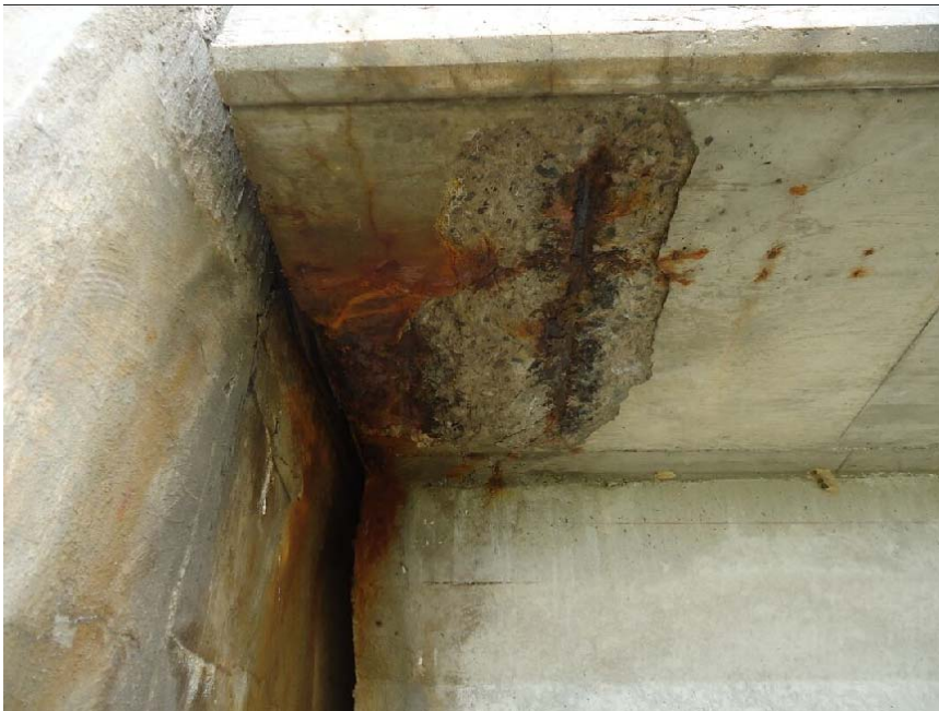
Figure 113. Exposed rebar, showing insufficient concrete cover at end of bridge deck (IN-W)
