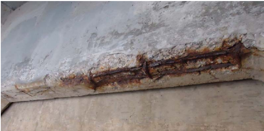
Figure 193. Corrosion and deterioration of underside of diaphragm
