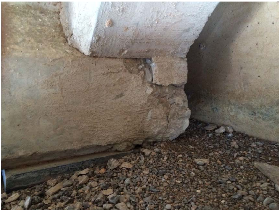
Figure 168. Spalling at diaphragm and girder interface (3W-N)
