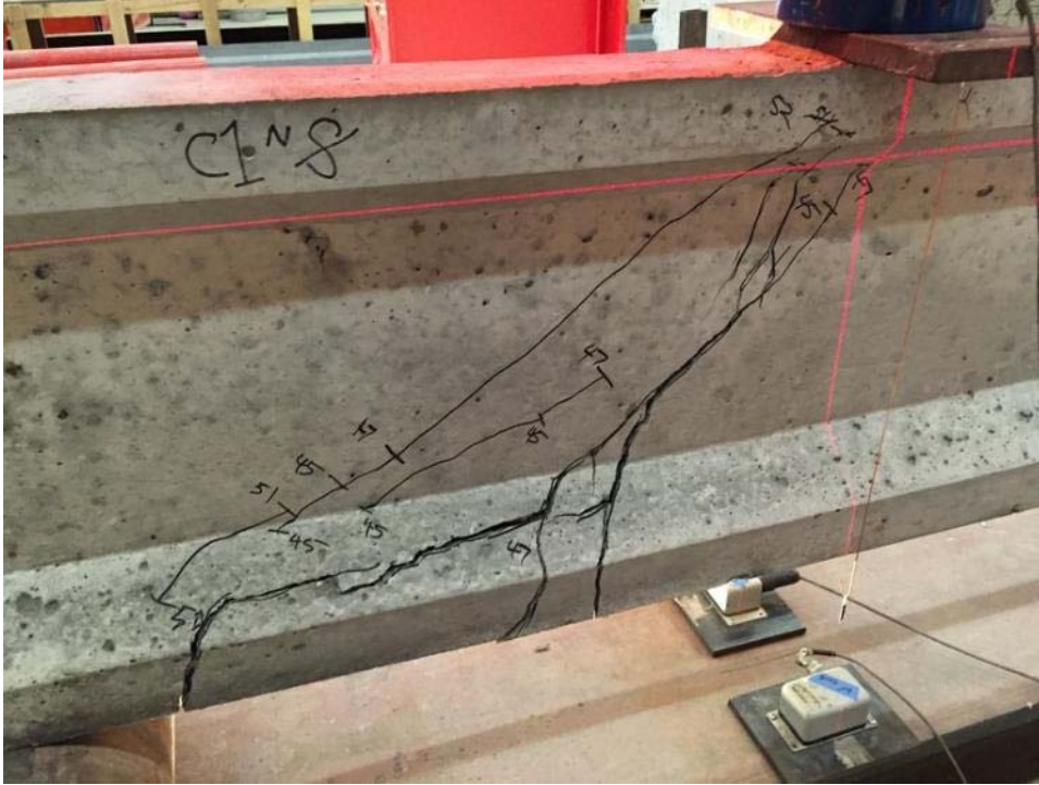
Figure 31. Visual Map of Cracking for Shear Test on C1NC
