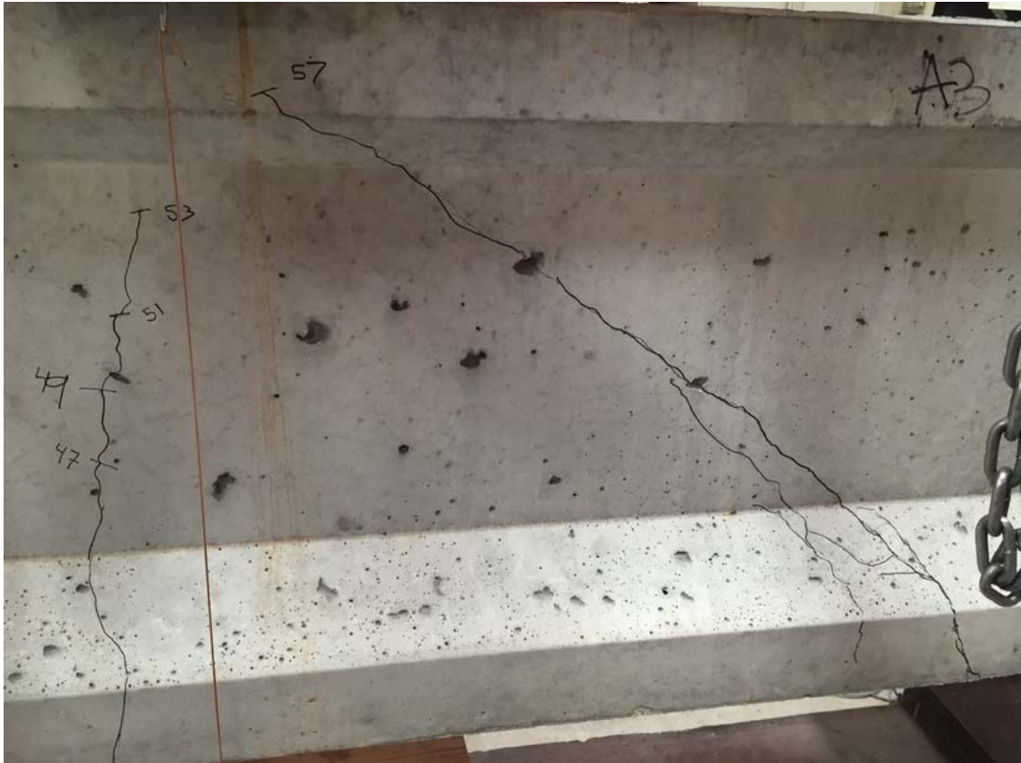
Figure 42. Web shear and flexural cracks of Girder A3SC
