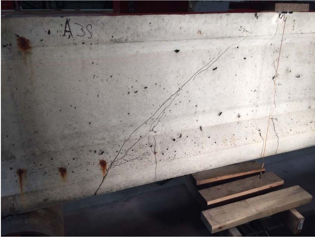
Figure 40. Web-shear crack on A3SC
