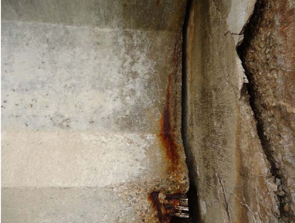
Figure 144. Vertical cracking with visible corrosion on exterior, exposed girder (12E-S)
