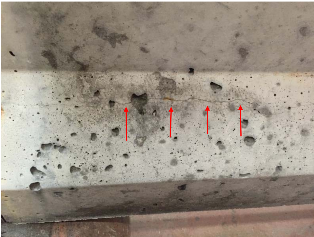
Figure 47. Horizontal crack below the web/flange interface of C2NC
