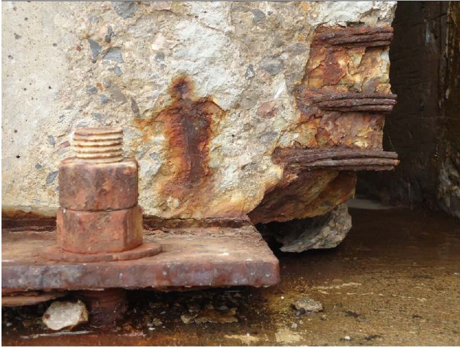
Figure 145. Exposed prestressing strands of an exposed, exterior girder (1W-N)
