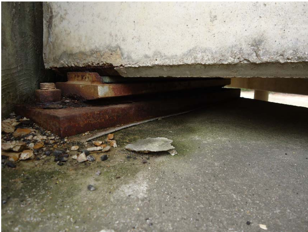
Figure 130. Spalling above corroded support of exposed, exterior girder (1E-N)
