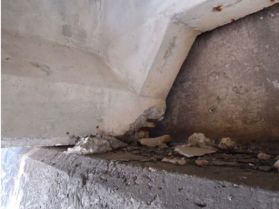
Figure 197. Diagonal back corner spalling of diaphragm and exposed prestressing strands (5S-W)
