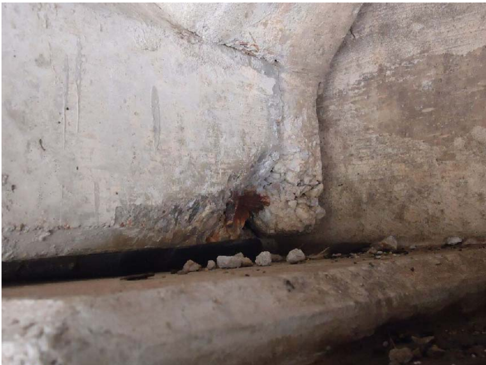
Figure 190. Exposed rebar, back corner spalled (2S-W)
