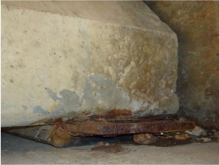
Figure 149. Spalling above corroded bearing plate, missing anchor bolt (10E-S)
