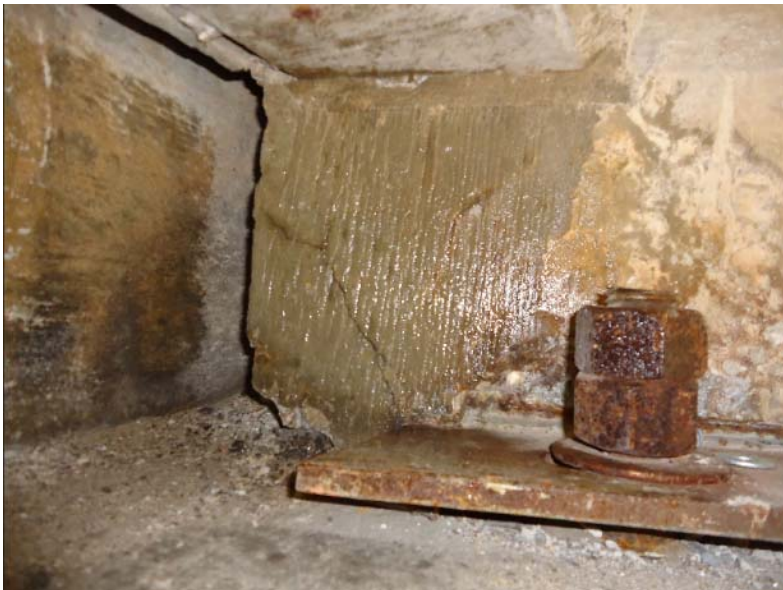
Figure 129. Back corner diagonal cracking of beam end (5W-S)
