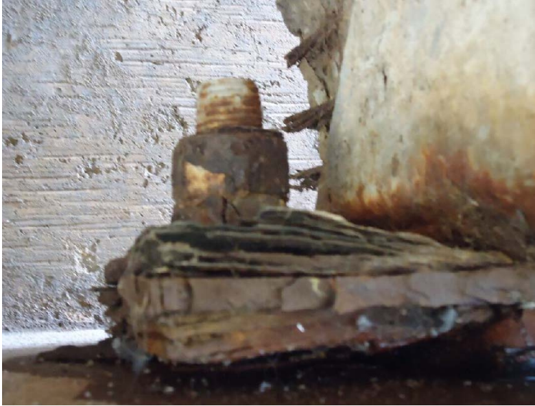
Figure 147. Corroded and flaky bearing plate, not providing much functionality as original designed (1W-S)
