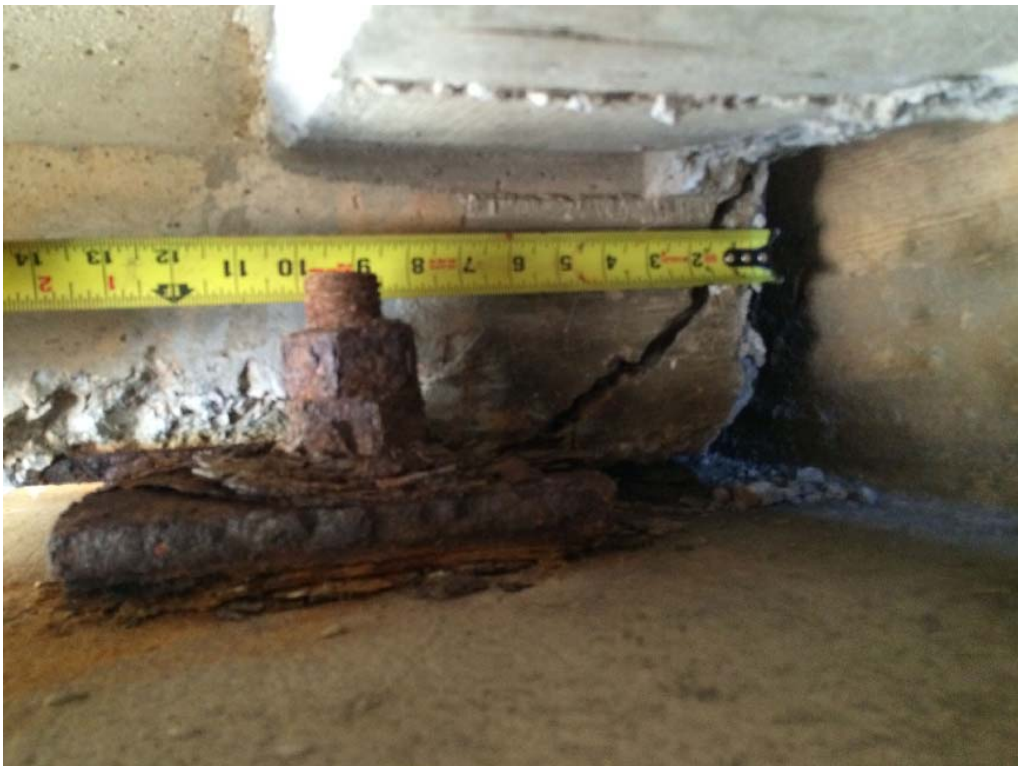
Figure 171. Corroded bearing plate and diagonal back corner crack with a maximum width of approx. five inches (2W-N)
