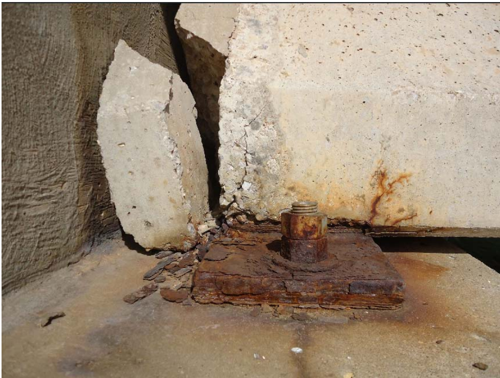
Figure 165. Spalling girder end and corroded bearing plate (5W-S)
