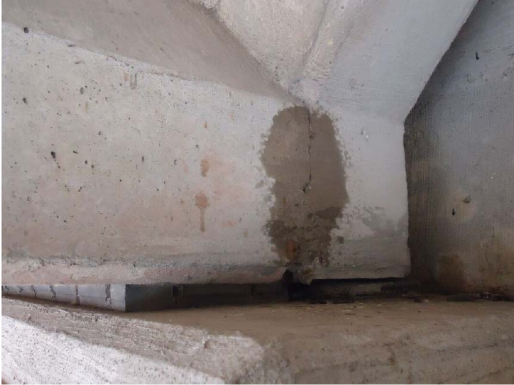
Figure 189. Vertical crack at bottom flange and diaphragm interface (3N-E)
