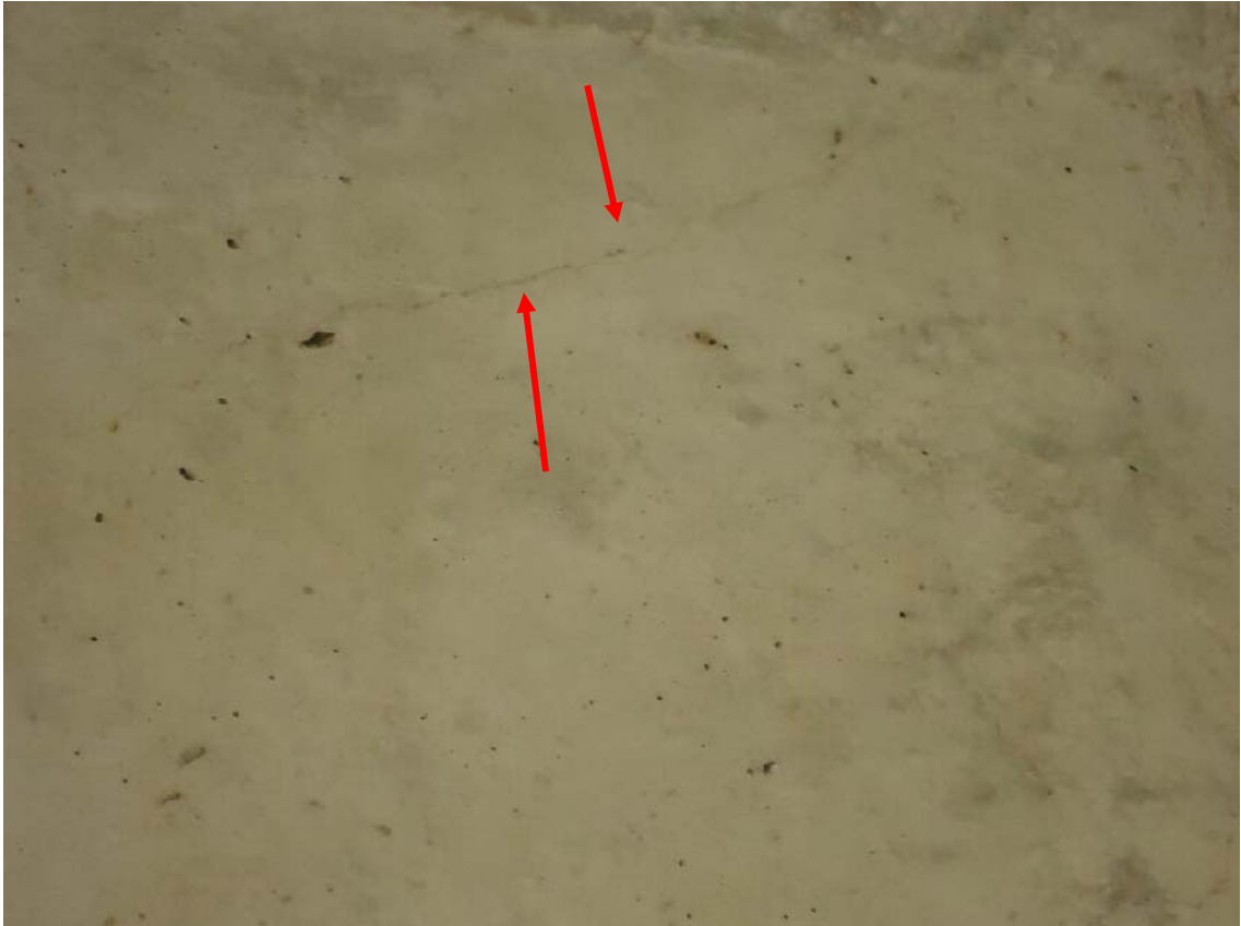
Figure 191. Diagonal crack from top flange and web interface (2S-W)
