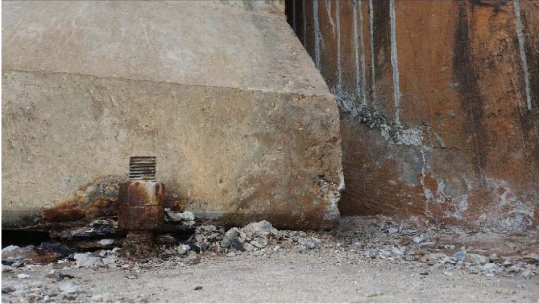
Figure 91. Example of spalling above bearing support
