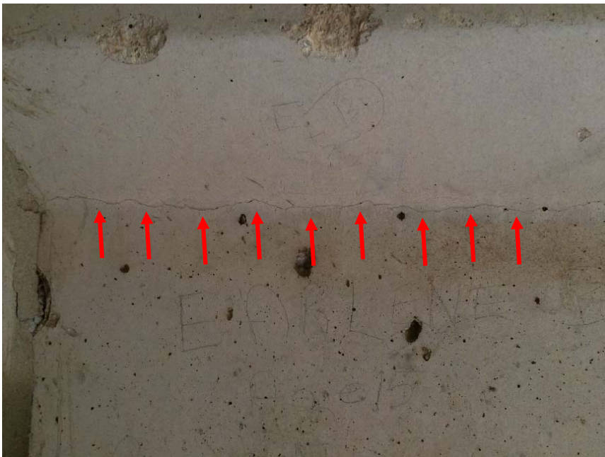
Figure 136. Crack along intersection of the top flange and web
