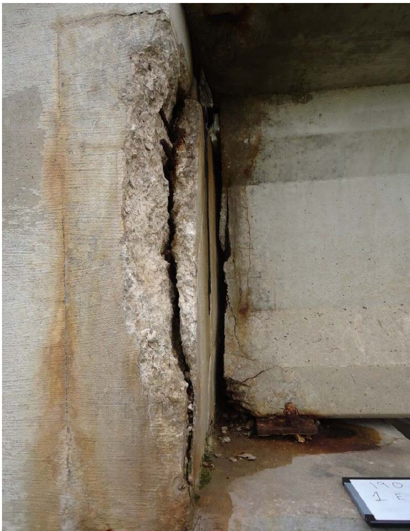
Figure 143. Extreme deterioration of back wall and girder end due to moisture/water (1E-N). The exposed, exterior girder has a corroded bearing plate and spalling occurring at the girder end.
