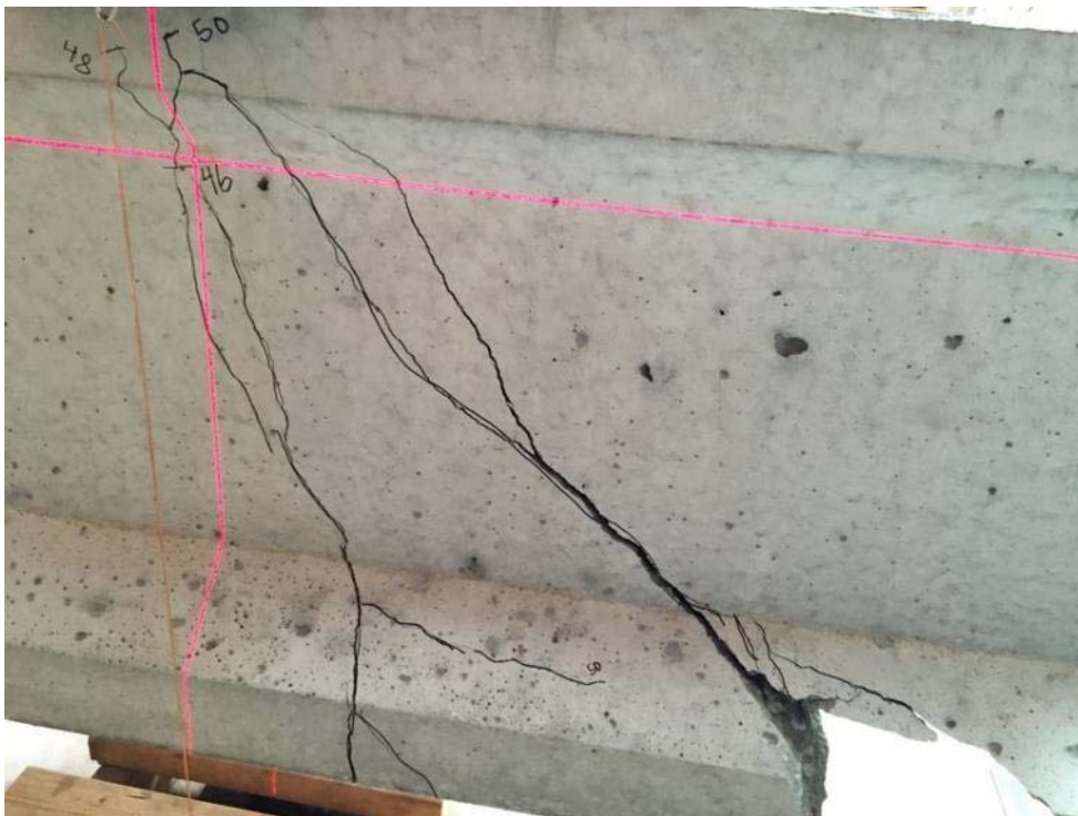
Figure 45. Visual Map of Cracking along A3N
