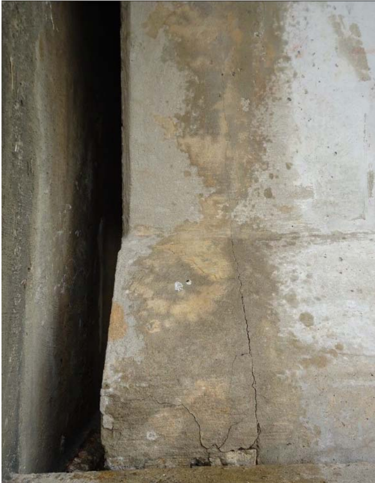
Figure 188. Vertical crack at girder/diaphragm interface (1N-W)
