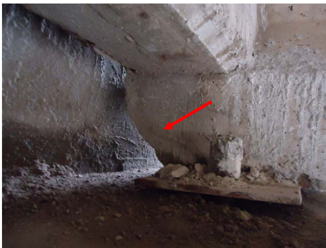
Figure 121. Spalled back corner of beam end (1W-S)
