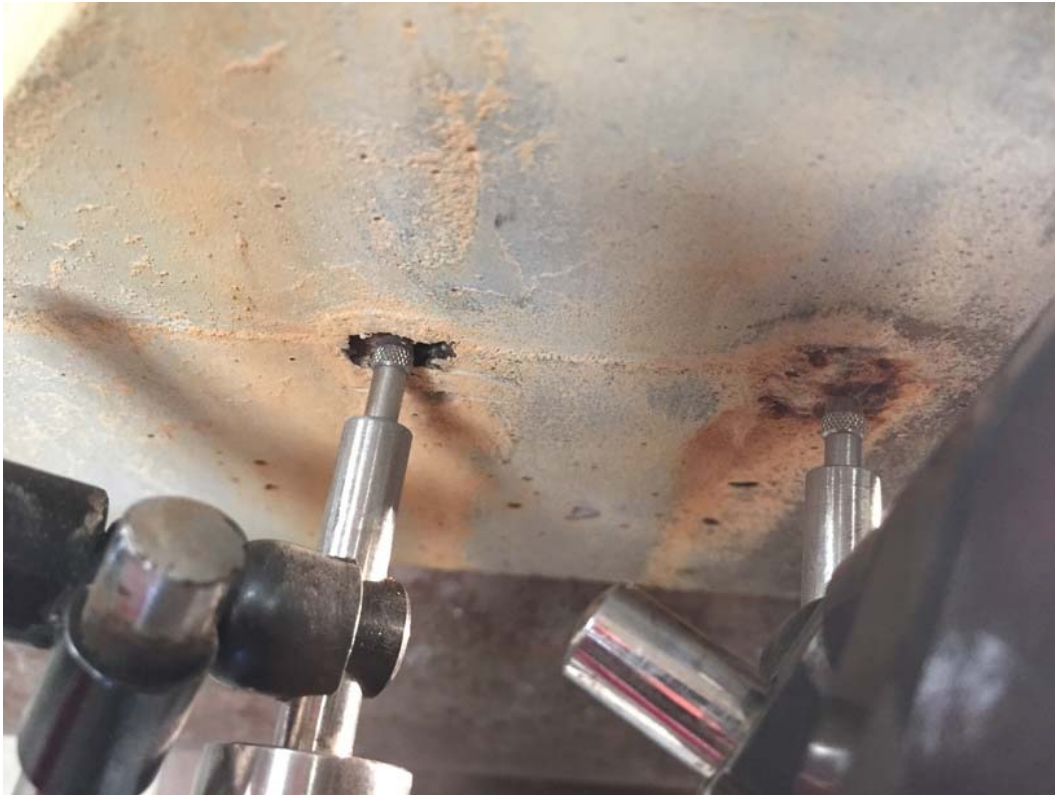
Figure 72. Visible Slip of A2SC
