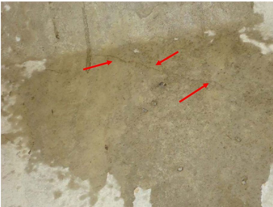
Figure 101. Example of diagonal cracking from the top flange and web interface
