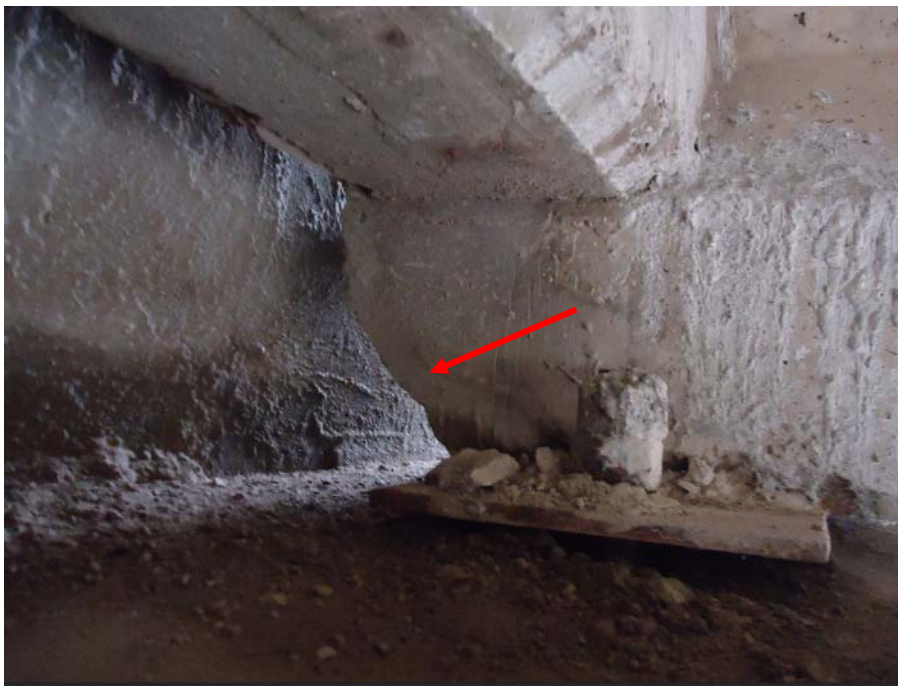
Figure 95. Example of back diagonal cracking/spalling
