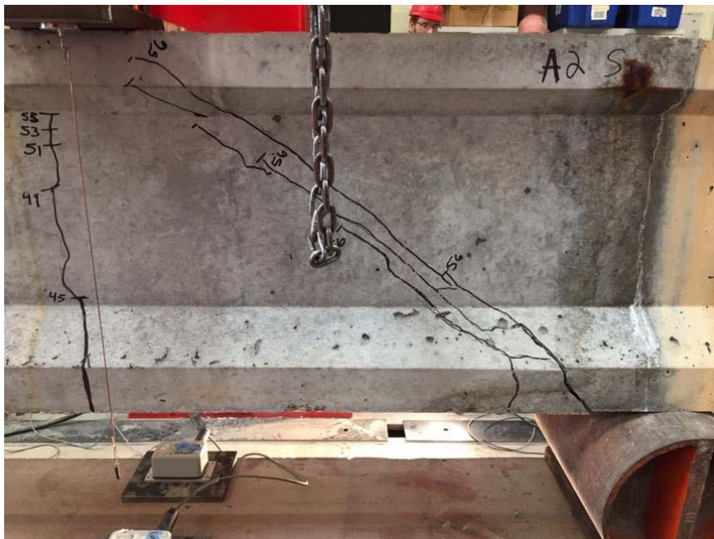
Figure 70. Visual map of cracking of A2SC
