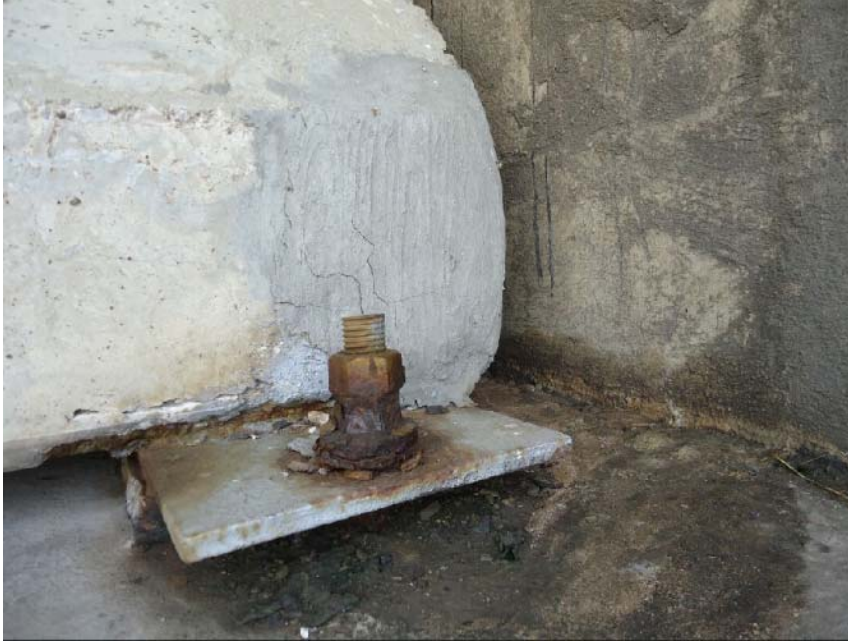
Figure 114. Repaired concrete on girder end and corroded bolt (IS-W)
