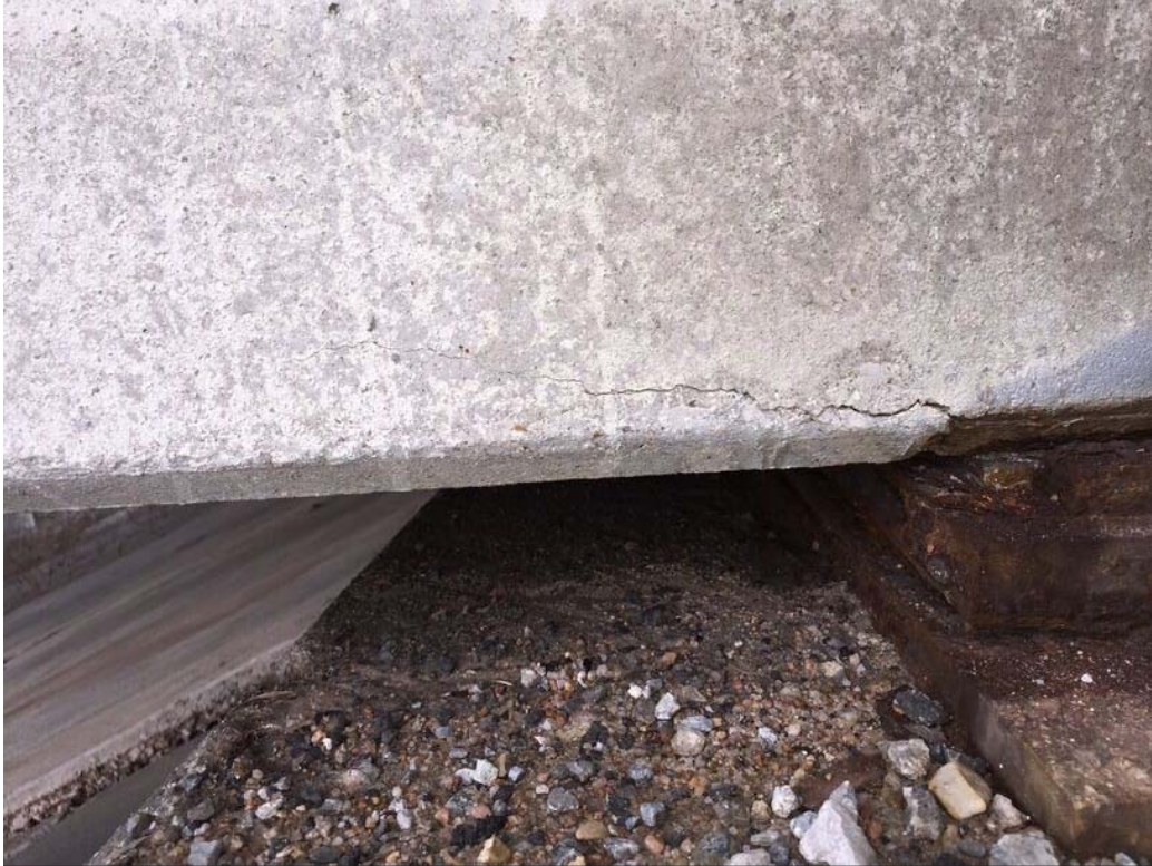
Figure 92. Example of crack from damage around the bearing plate
