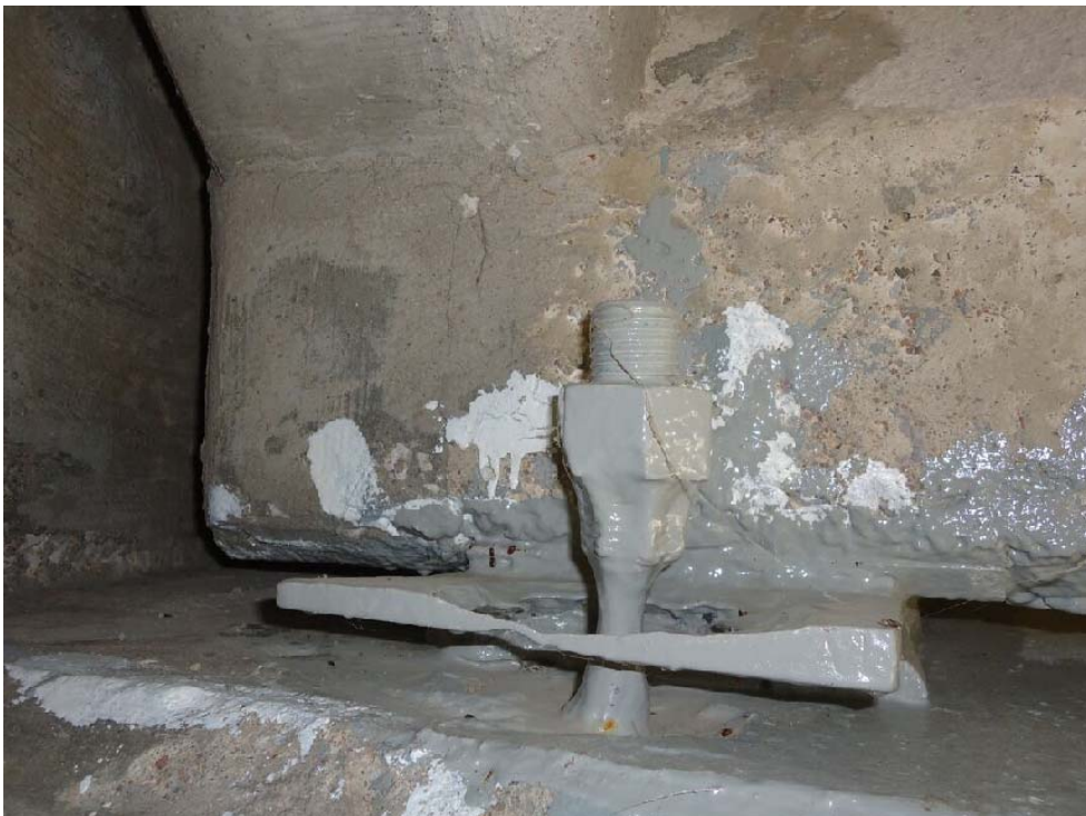
Figure 183. Necked anchor bolt and bearing plate both deteriorated and coated (2S-E)
