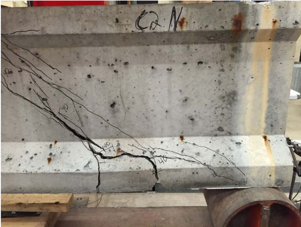
Figure 51. Visual Map of cracking of C2NC
