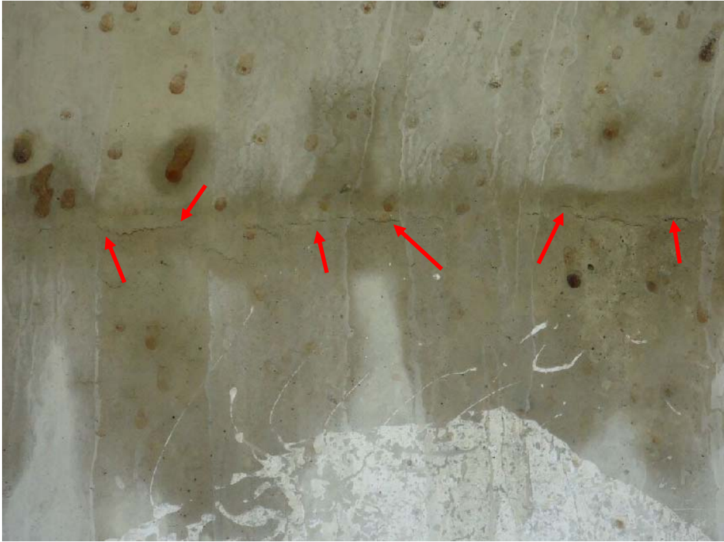
Figure 99. Example of horizontal cracking along the top flange and web interface
