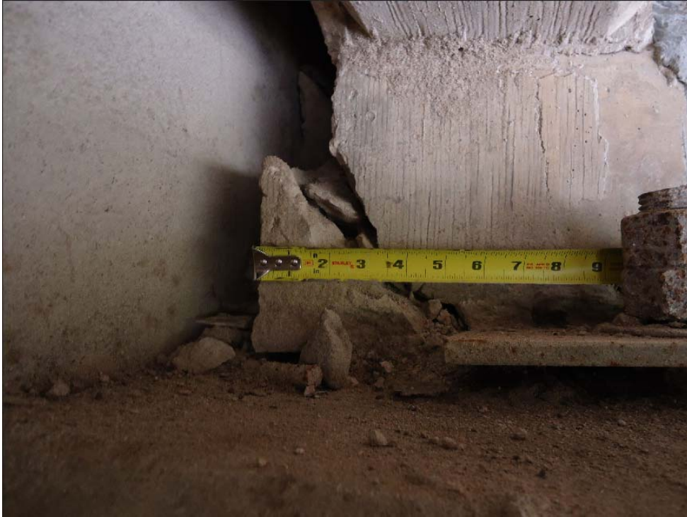
Figure 122. Spalled back corner of beam end (4E-N)
