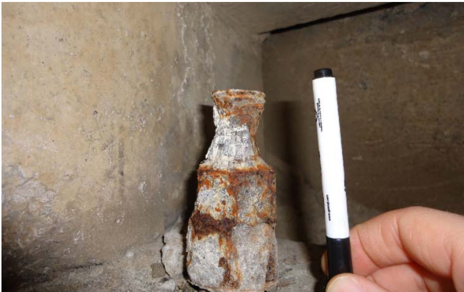
Figure 127. Close-up of deterioration of anchor bolt, with necking at the top (4E-S). The pen is shown in the picture to illustrate the amount of necking occurring to the steel member.
