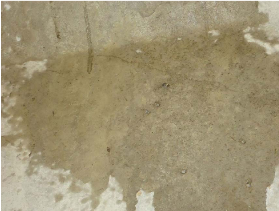
Figure 196. Diagonal crack from top flange and web intersection going further into the web (5N-W)
