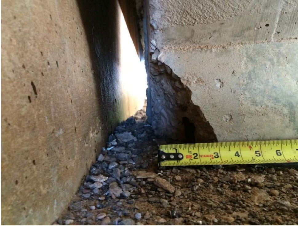
Figure 167. Back corner diagonal crack with a width at the base of approximately three inches (2E-N)
