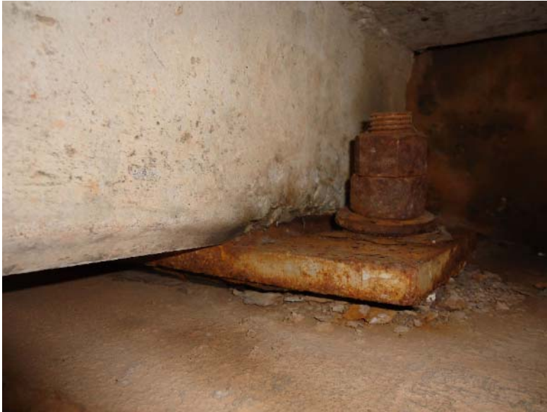
Figure 158. Corroded bearing plate and anchor bolt, with spalling above the support (5E-S)
