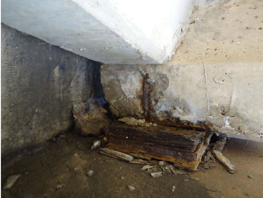
Figure 175. Exposed rebar, corroded, flaky bearing plate, and spalling of concrete (5E-N)
