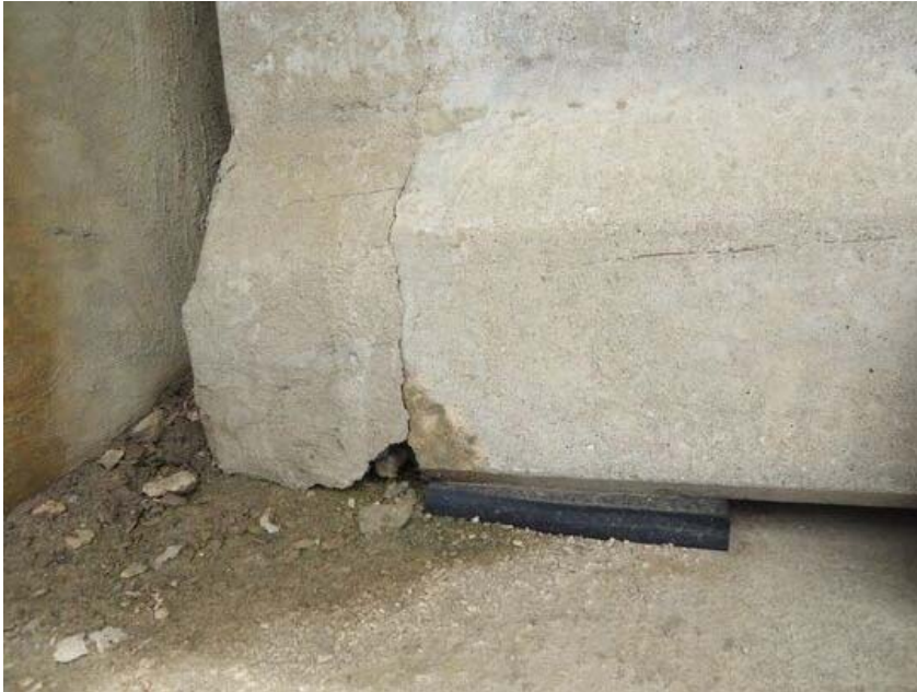
Figure 119. Separation at the diaphragm and girder end (1N-W)
