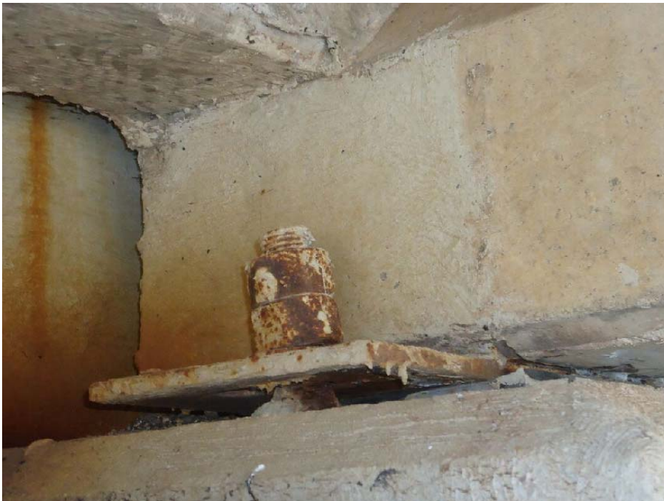
Figure 153. Corroding anchor bolt (4S-E)
