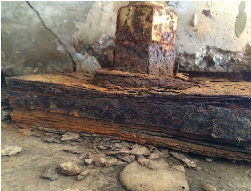
Figure 173. Corroded, flaky bearing plate
