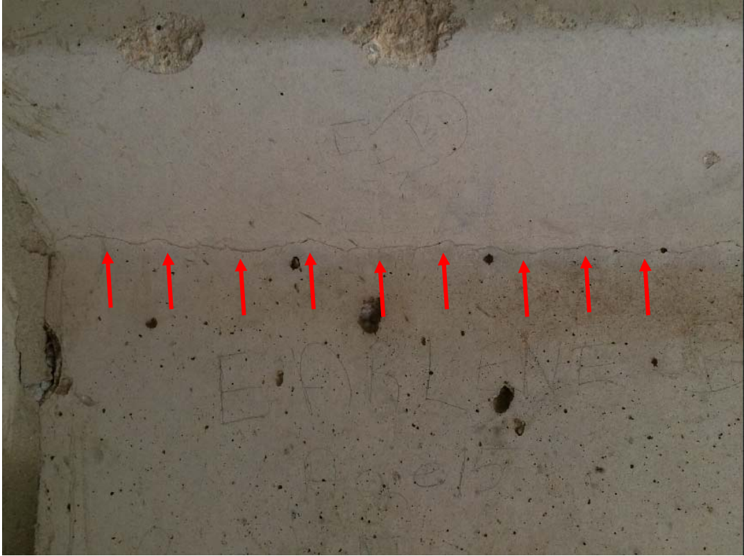
Figure 98. Example of horizontal cracking along the top flange and web interface
