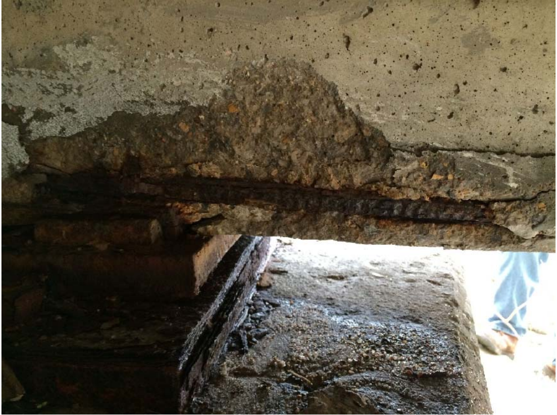
Figure 135. Exposed rebar due to spalled concrete (1N-W)
