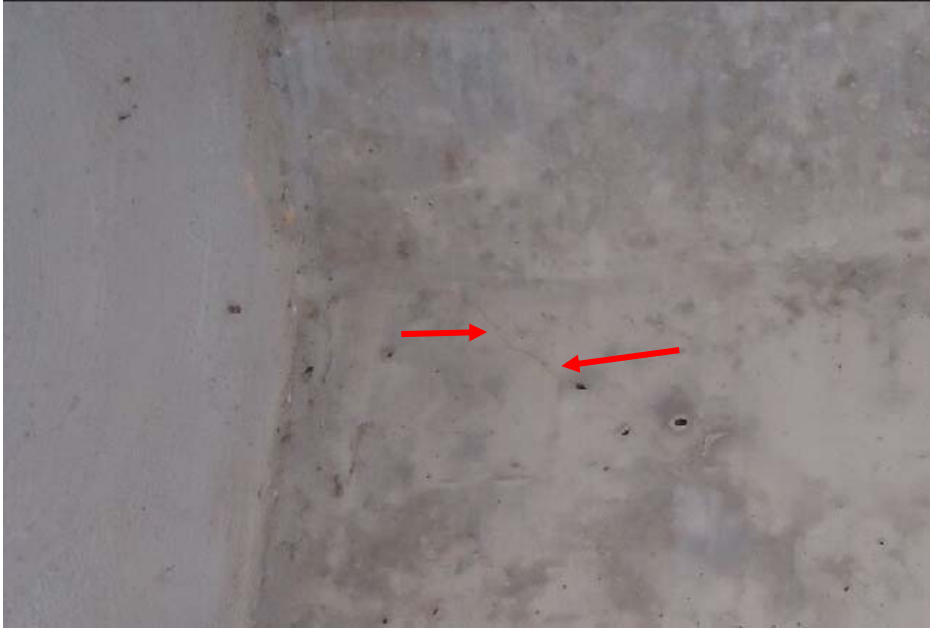
Figure 115. Diagonal cracking on the web of the beam (3N-W)
