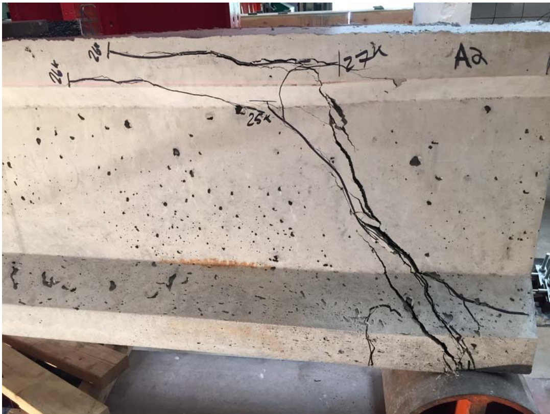
Figure 76. Cracking along the flange and web of A2N
