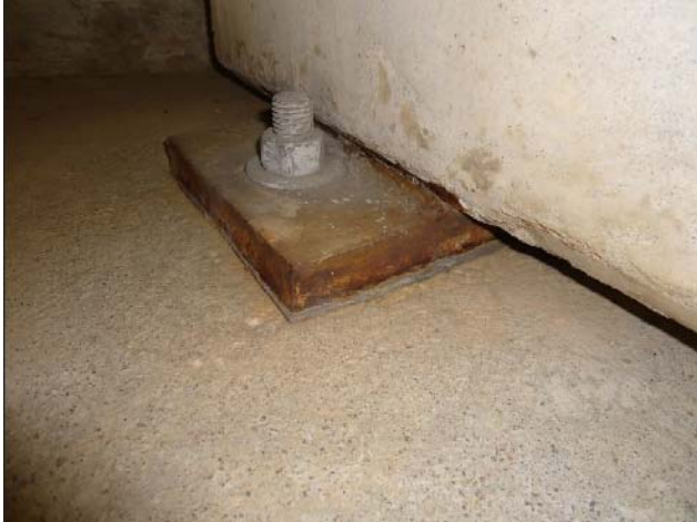
Figure 108. Example of corroding bearing plate (2W-S)
