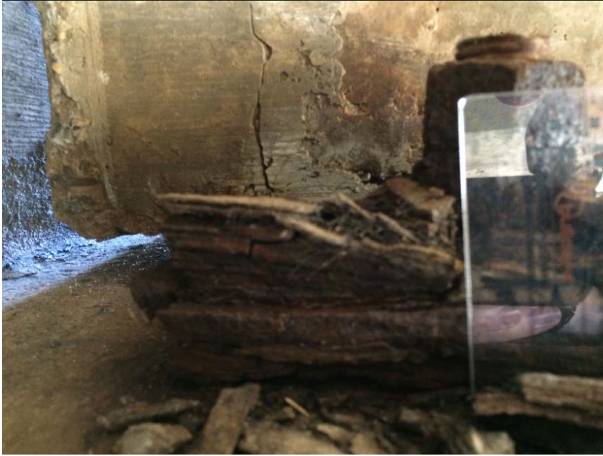
Figure 174. Vertical crack along interface of girder end and diaphragm (1W-S)
