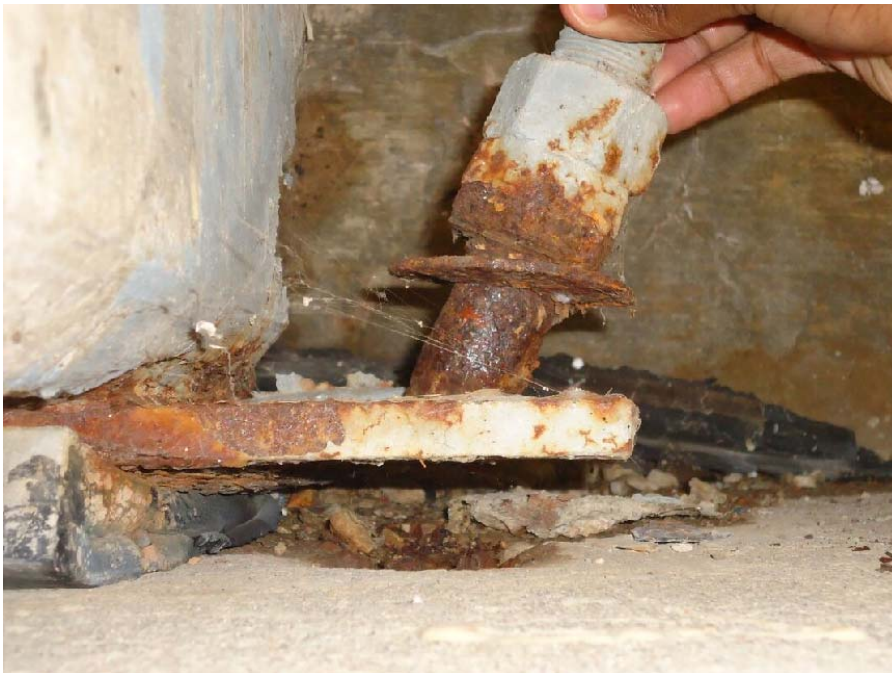
Figure 148. Corrosion at cavity of abutment and bolt interface (7E-S)
