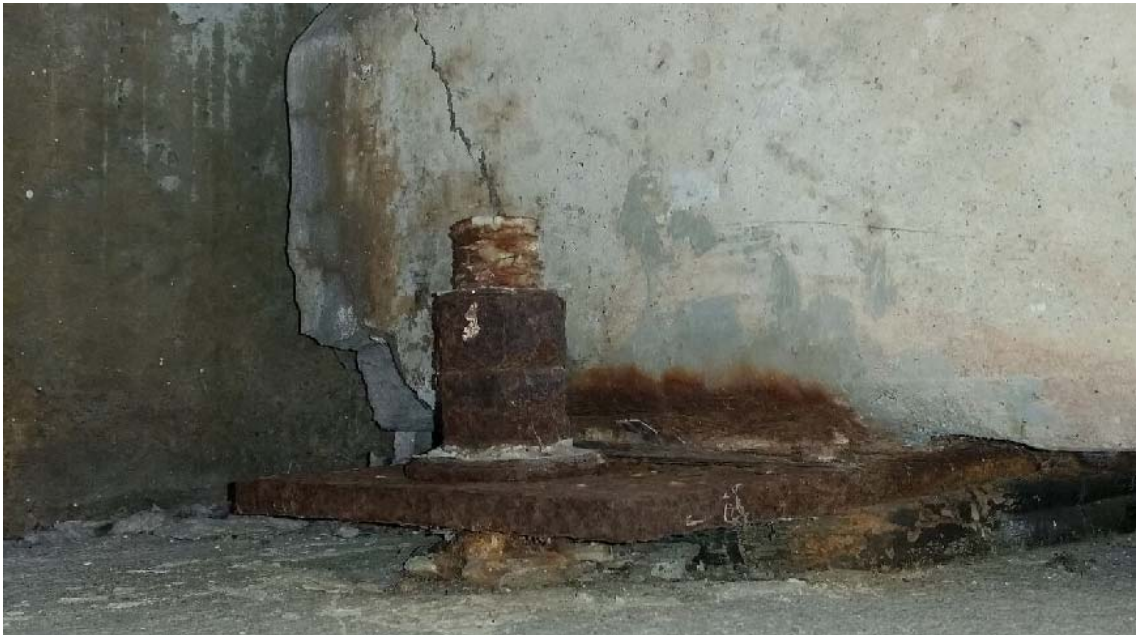
Figure 150. Back corner diagonally cracked on beam end (11W-S)
