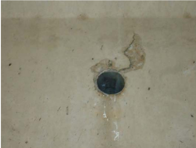
Figure 151. Spalling and cracking above pipe in web (1N-E)
