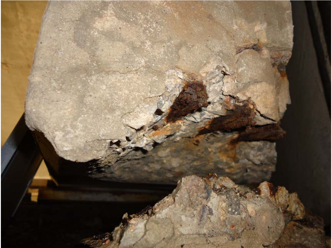
Figure 133. Spalled back corner and exposed prestressing strands
