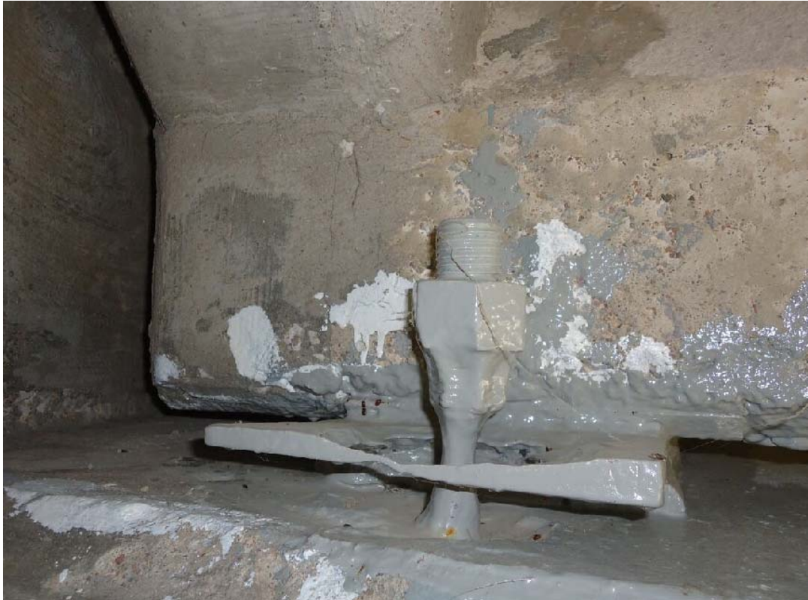
Figure 90. Example of coated, damaged anchor bolt and nut
