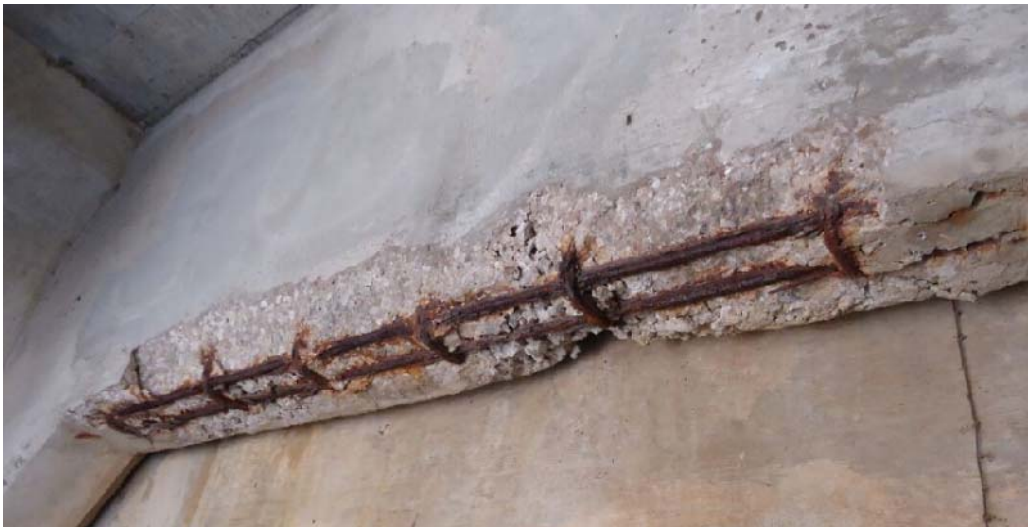
Figure 103. Example of Diaphragm deterioration
