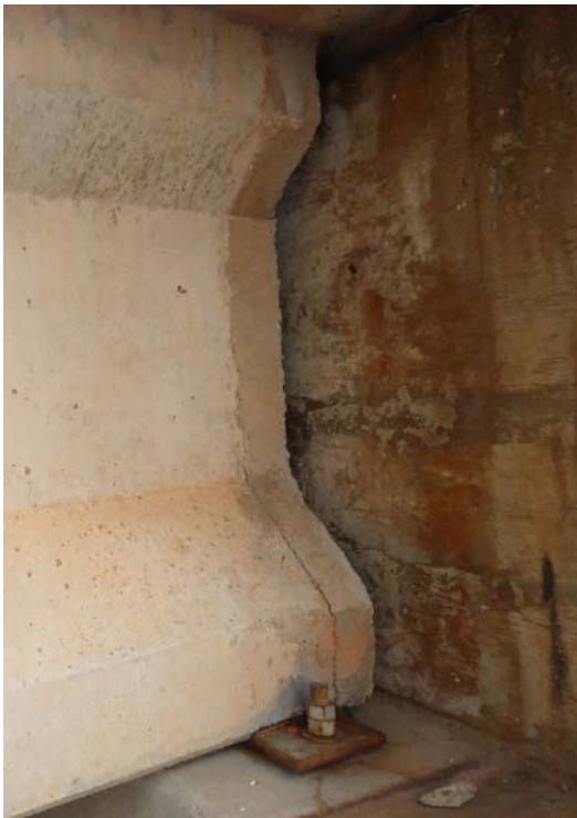
Figure 163. Vertical separation of diaphragm and girder at interface (5E-S)
