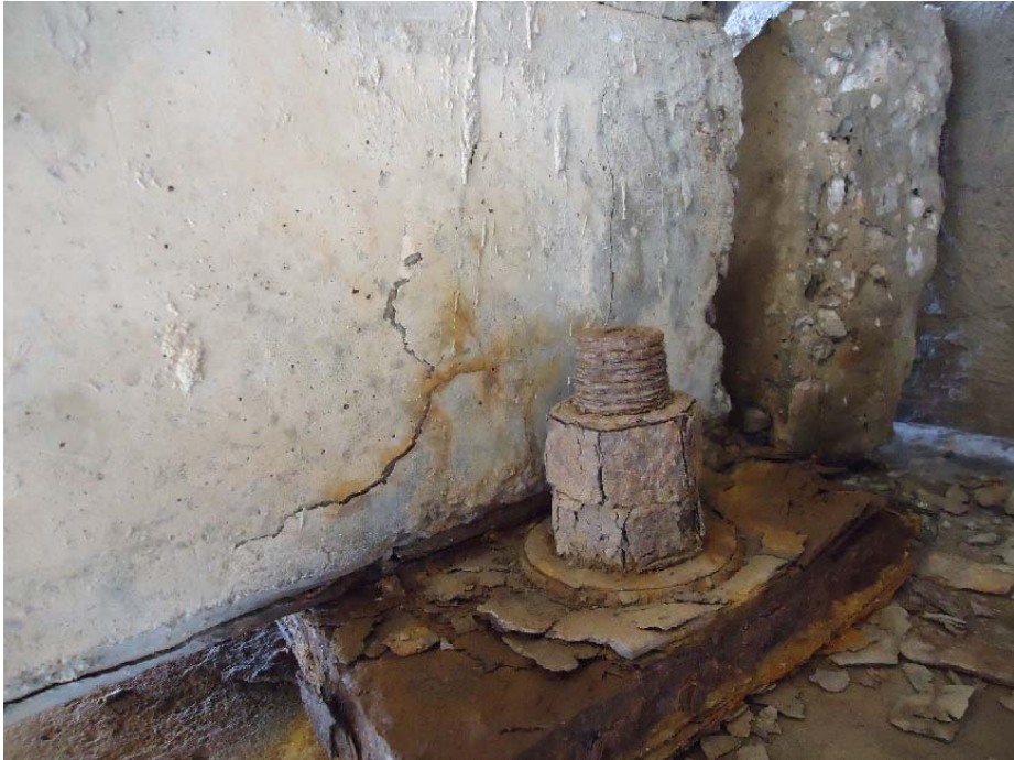
Figure 164. Corroded bearing plate and anchor bolt, with spalling and cracking above the corroded bearing plate (5W-N)
