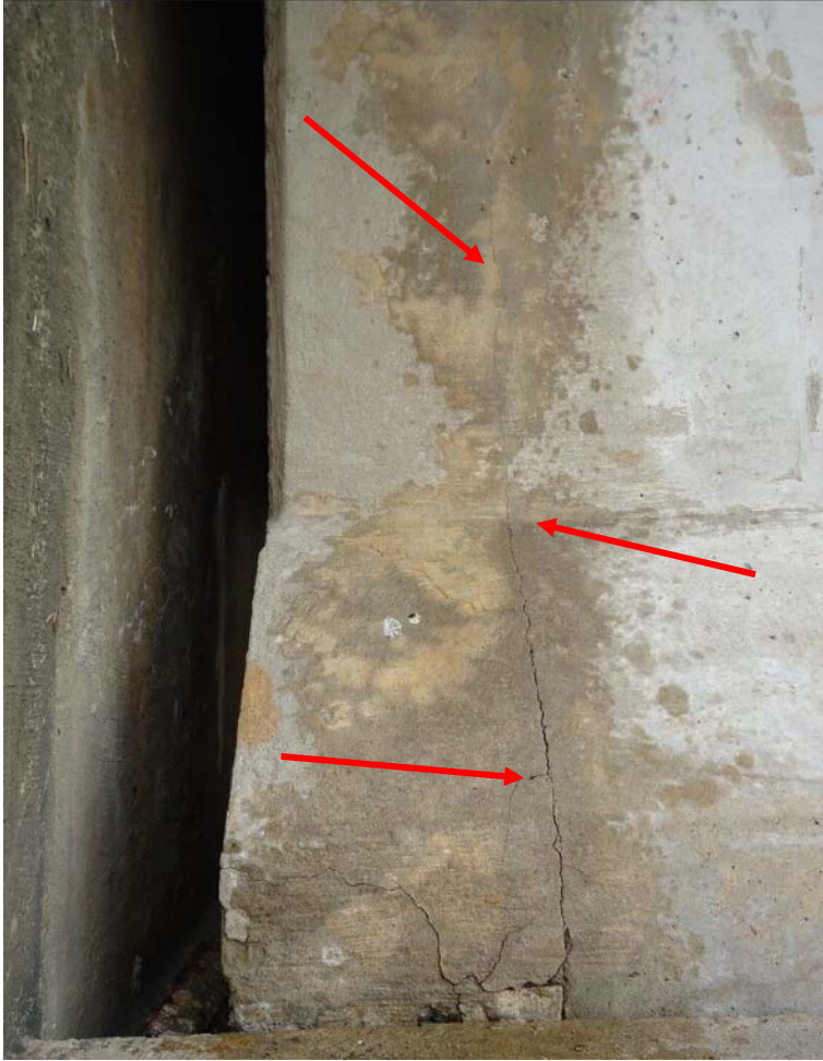
Figure 97. Example of vertical cracking along diaphragm and girder
