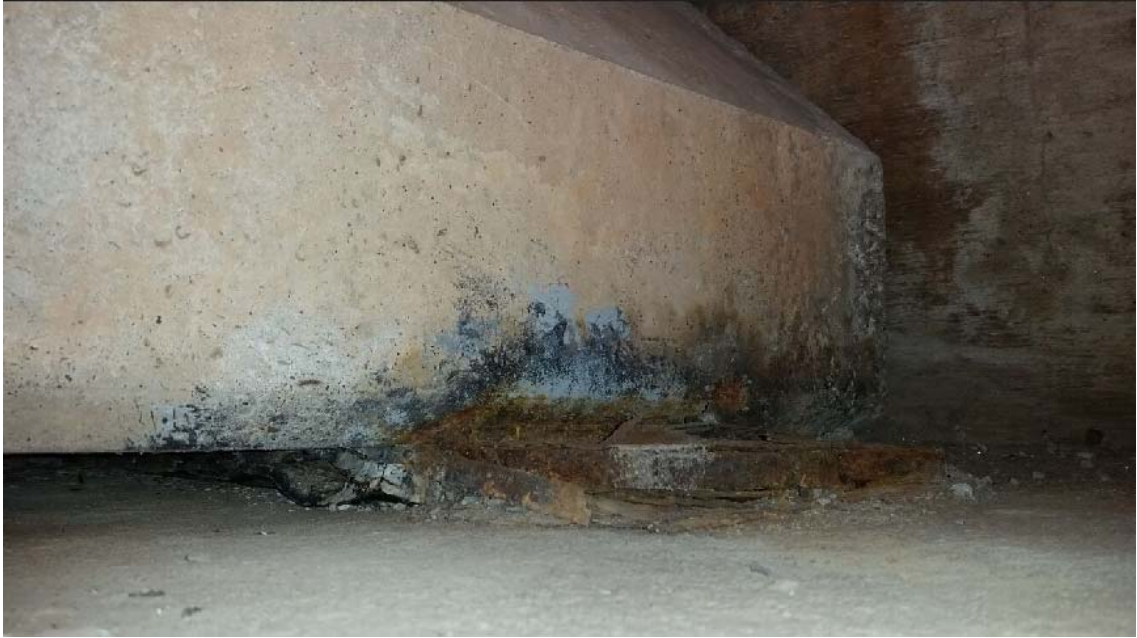
Figure 141. Corroded bearing plate, and spalling along bottom of girder and back of girder end (3S-W)
