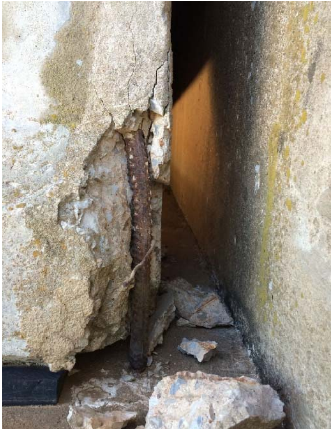
Figure 166. Exposed vertical rebar due to spalled girder end of exposed, exterior beam (1W-N)
