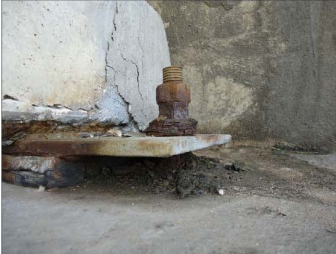
Figure 112. Corroded anchor bolt (IS-W)
