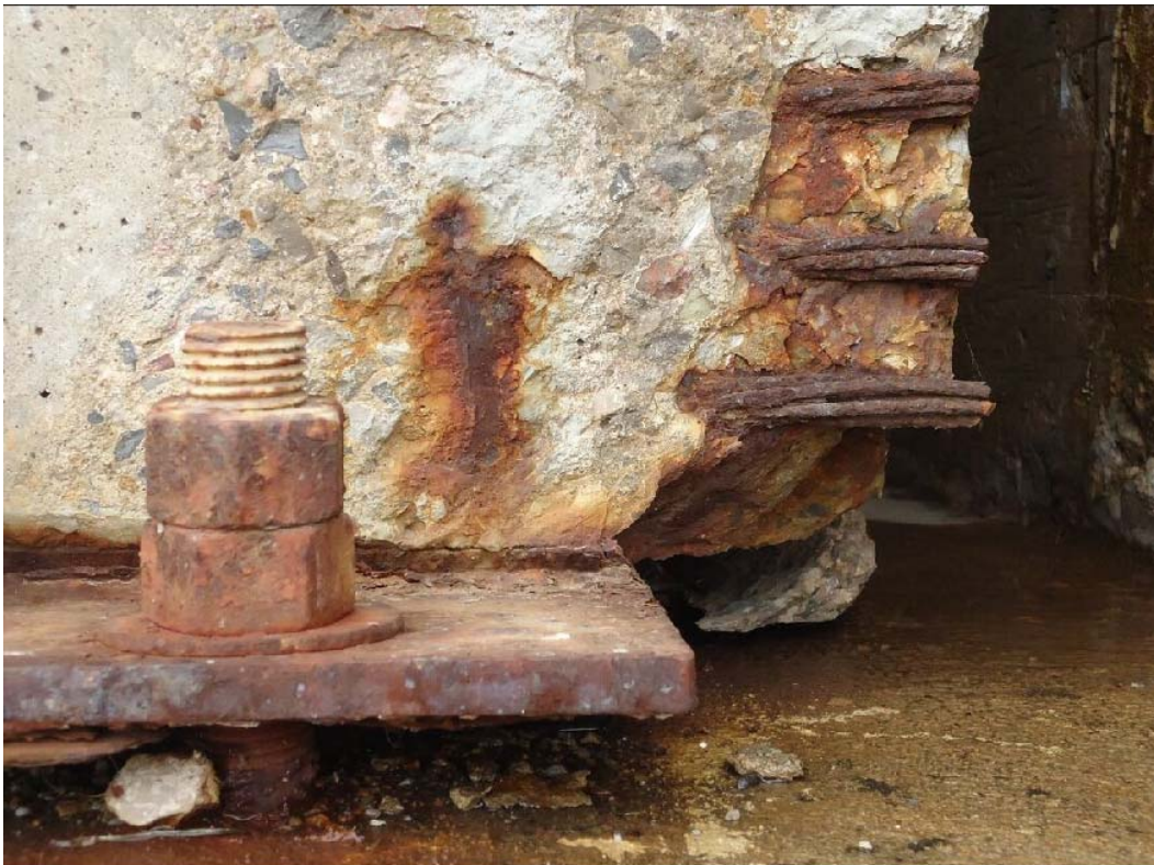
Figure 94. Example of exposed prestressing strands
