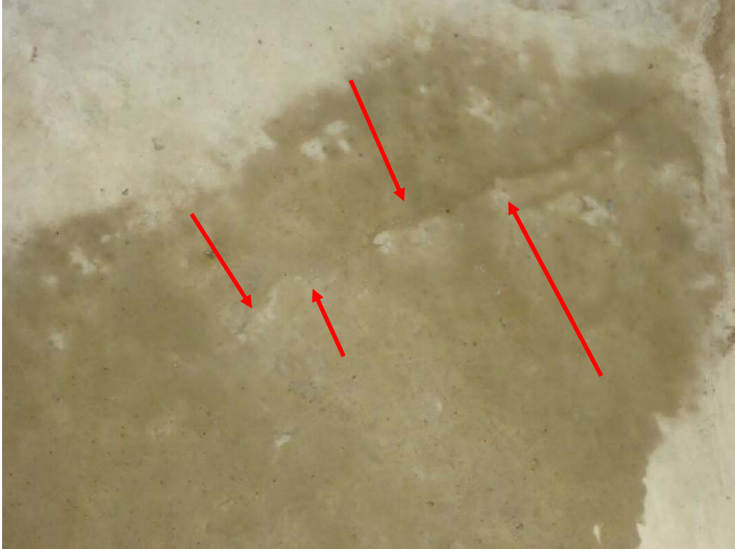
Figure 192. Diagonal crack from top flange and web interface
