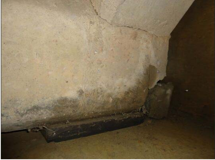
Figure 118. Back diagonal crack in the beam end (3N-E)
