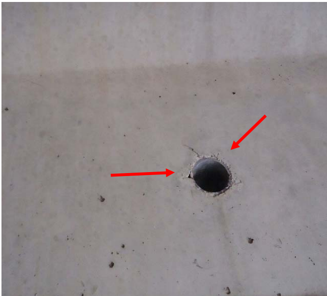
Figure 123. Crack from interior pipe that runs through web of beam (4E-N)
