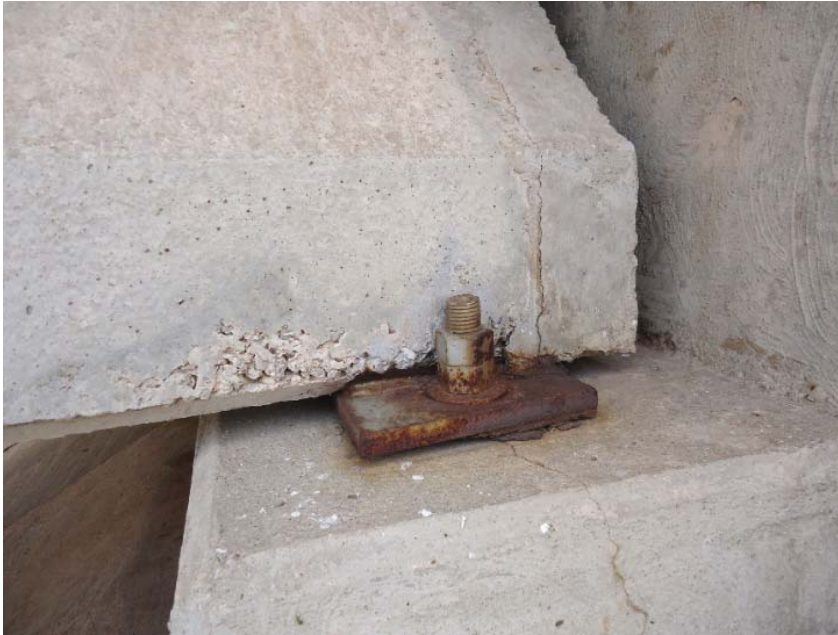
Figure 162. Spalling above the corroded bearing plate (1W-N)
