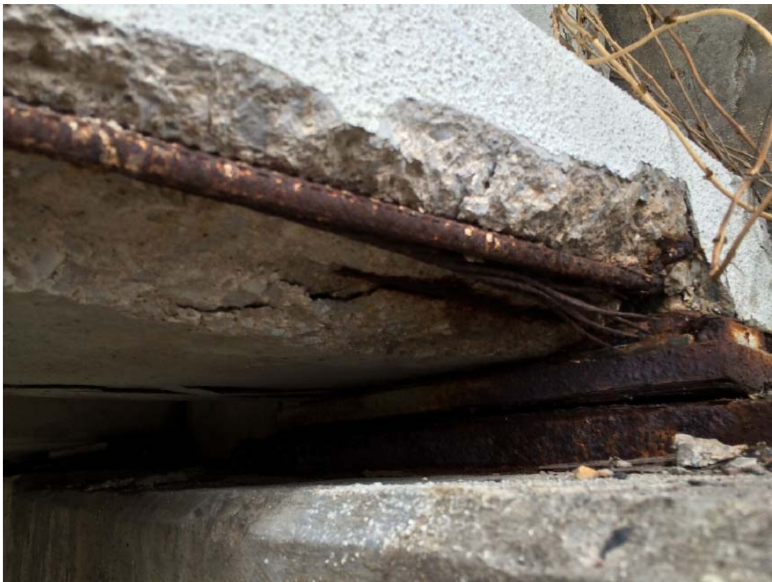
Figure 134. Exposed rebar due to spalled concrete on the bottom of an exposed, exterior girder (1N-E)
