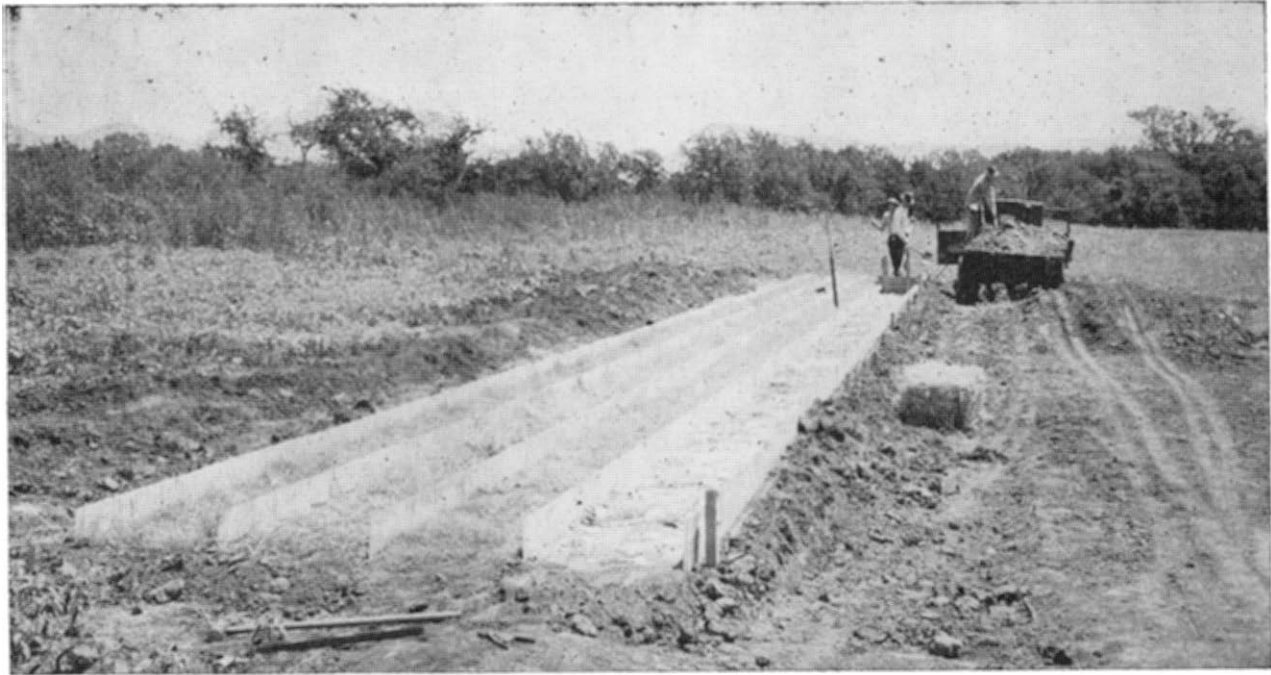
Figure 2.—Installing a channel on one percent slope, using 2" x 12" boards to hold the sheet iron separators to true alignment.
