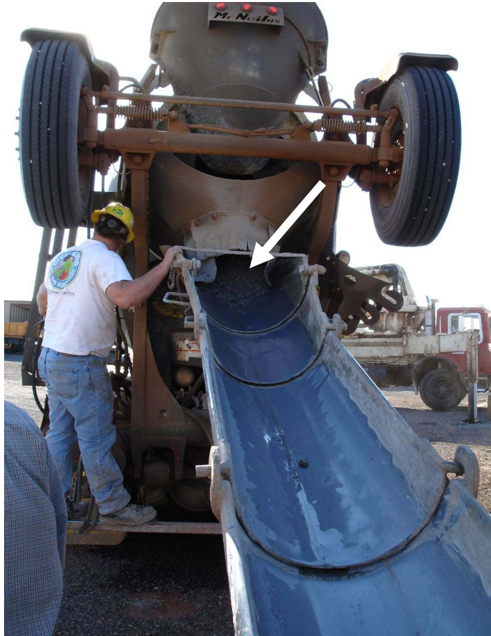
Figure 6.9 – Fiber Mixture Clogged In the Mixing Truck after the Pump Truck Attempt and Before the Additional Water
