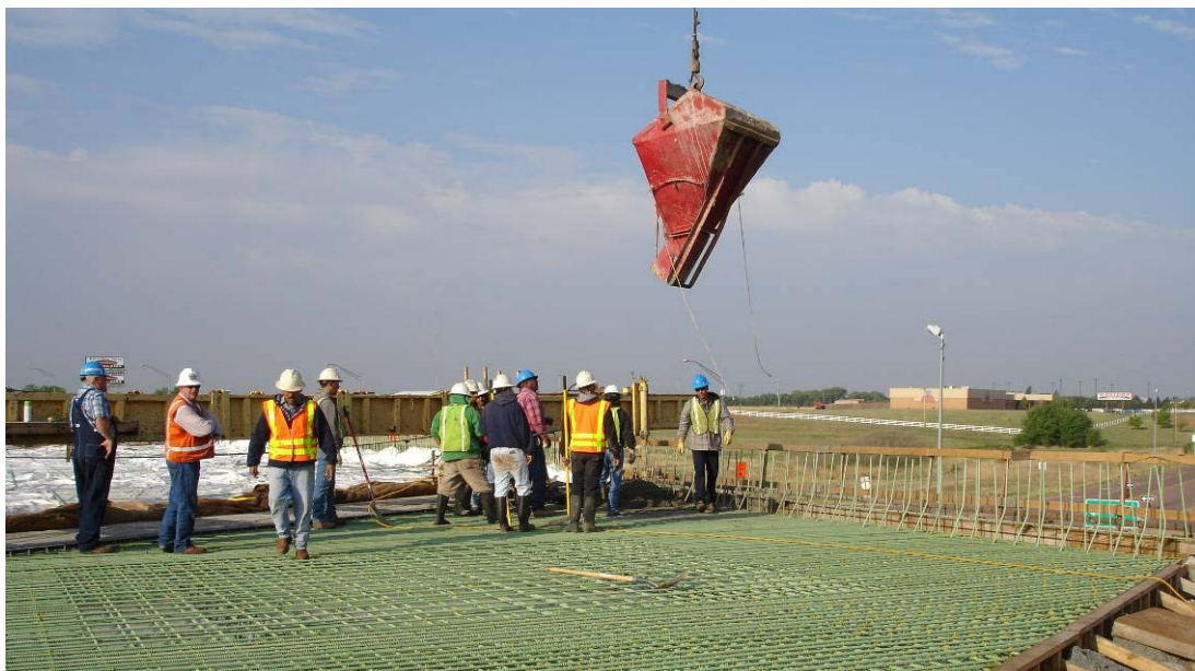
Figure 6. 18 – The Drop Bucket Being Used for the Application of the Fiber Mixture on Span 3
