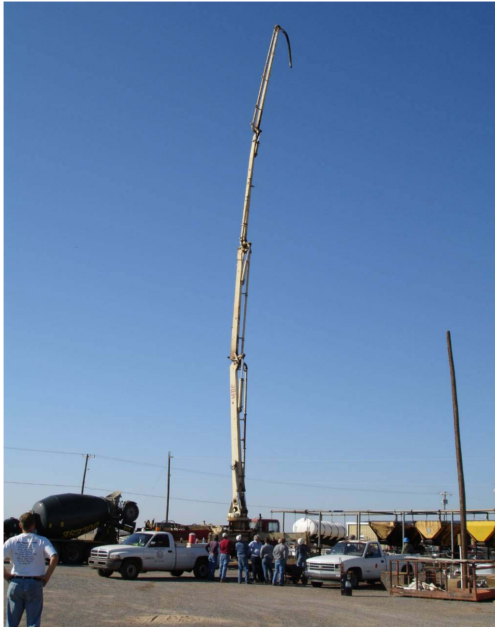
Figure 6. 8 –Back Pumping of the Pump Truck Boom Due to Being Clogged After Attempting to Pump the Fiber Mixture for Test Slab 2
