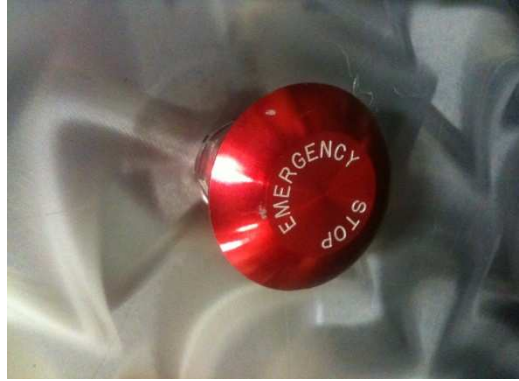
Figure 52. Emergency Shutdown Button
