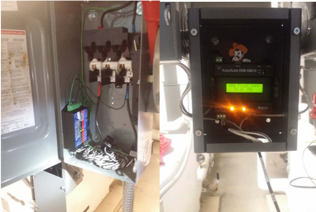
Figure 5.1 Electricity meter (left picture) and data acquisition system (right picture)
