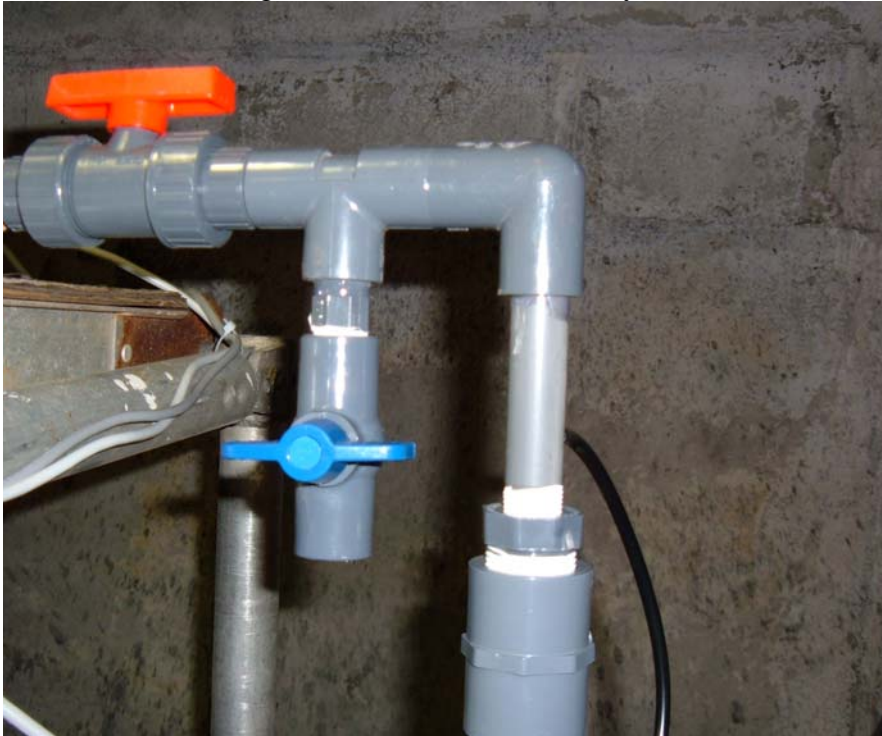
Figure 12: Connection of isolation valve to sample valve and static mixer
