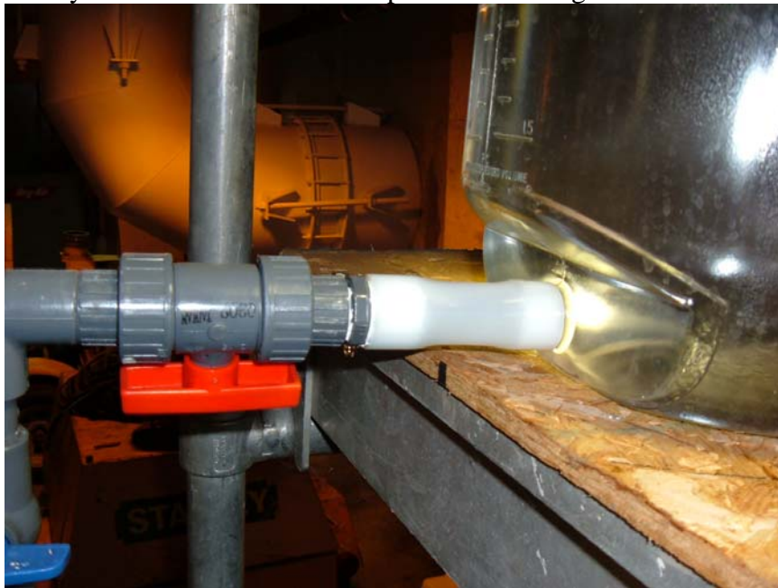
Figure 4: Carboy connection to isolation valve
