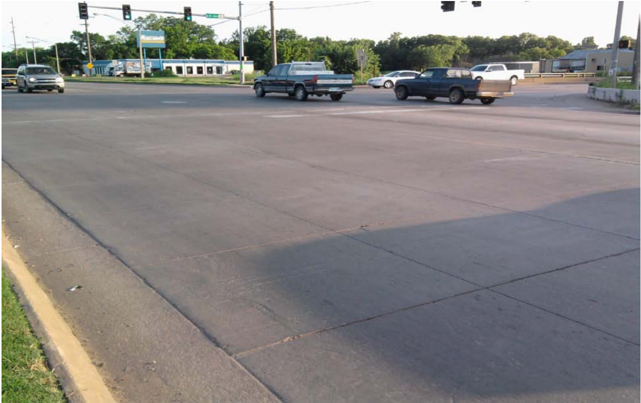
Figure 2.34 - Photo of intersection seen on US 177 towards south-west showing excellent condition of overlay.
