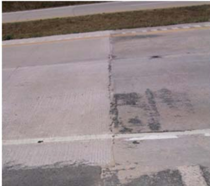
Figure 2.20 – The interface of the overlay and the adjacent pavement is in good condition.
