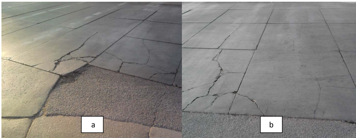
Figure 2.44 - Large block cracking at the east end of the intersection where the overlay is adjacent to the gas stations. The shadows shown in photo a show the difference in height between to the overlay and the adjacent asphalt. Additional block cracking can be seen in photo b.
