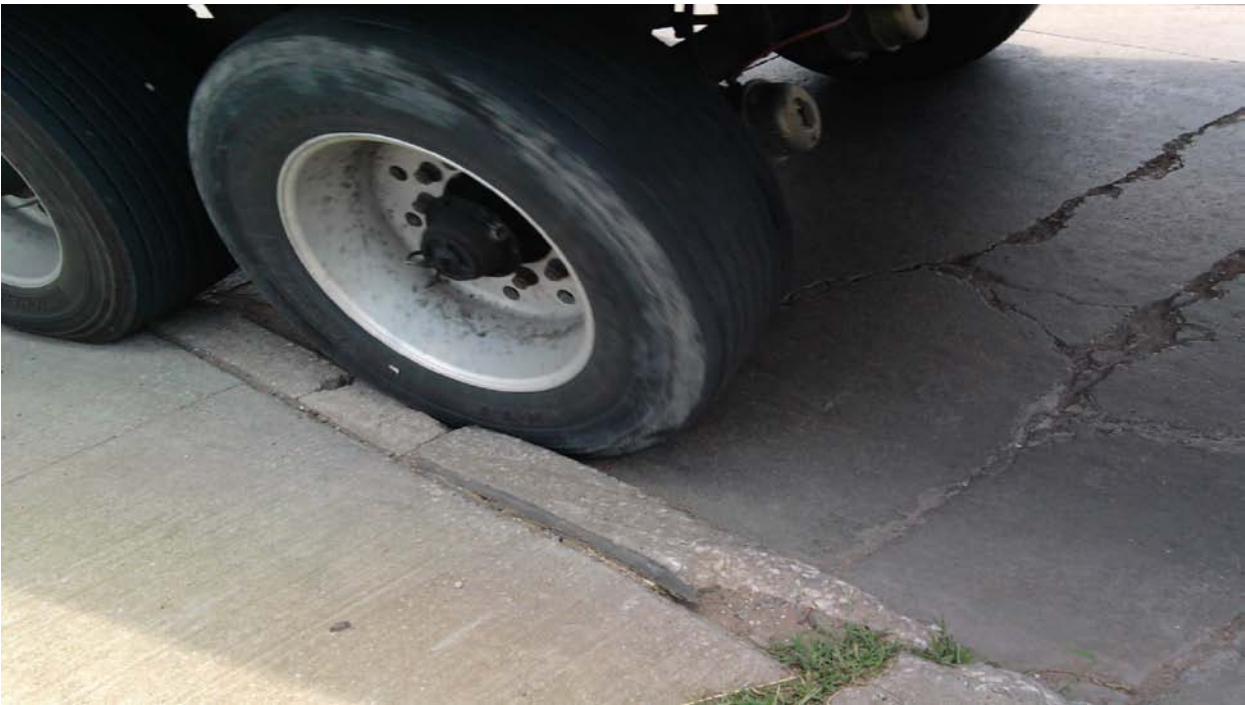
Figure 2.40 - Photo showing the impact loading due to lack of radius of curvature for large trucks.
