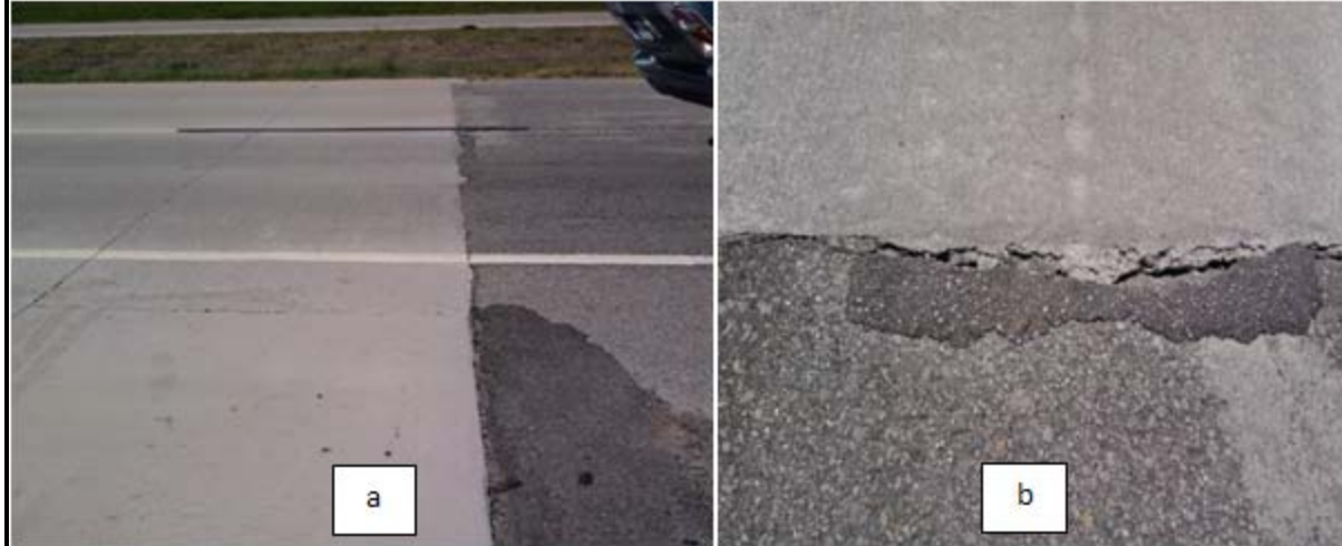
Figure 2.18 - Photo a shows the end of the overlay. The asphalt pavement looks good where it starts. But there is bit of distress initiation as shown in photo b.
