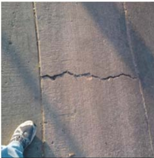
Figure 2.36 – Distress cracking in the shoulder.
