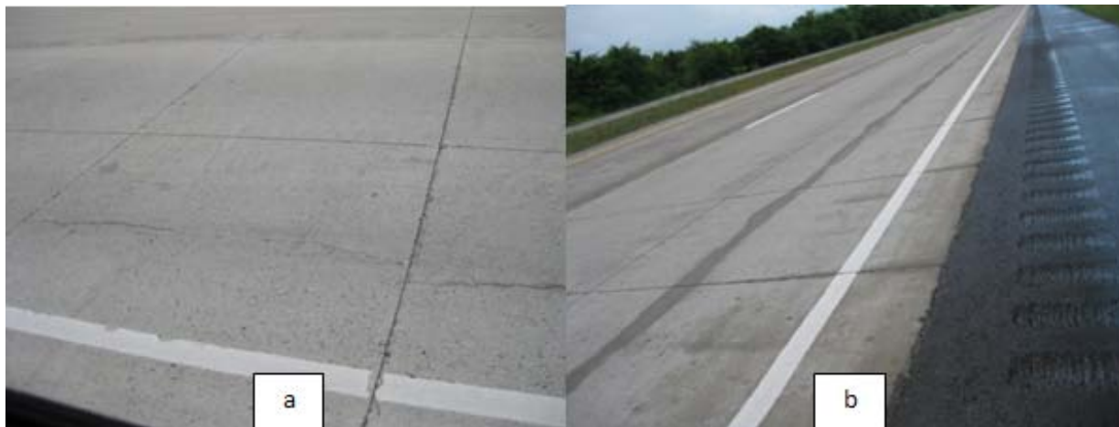
Figure 2.24 - Photo a showing the type of longitudinal cracking pattern. Photo b shows the cracks after heavy rains overnight. The seepage of water through the cracks is clearly visible.
