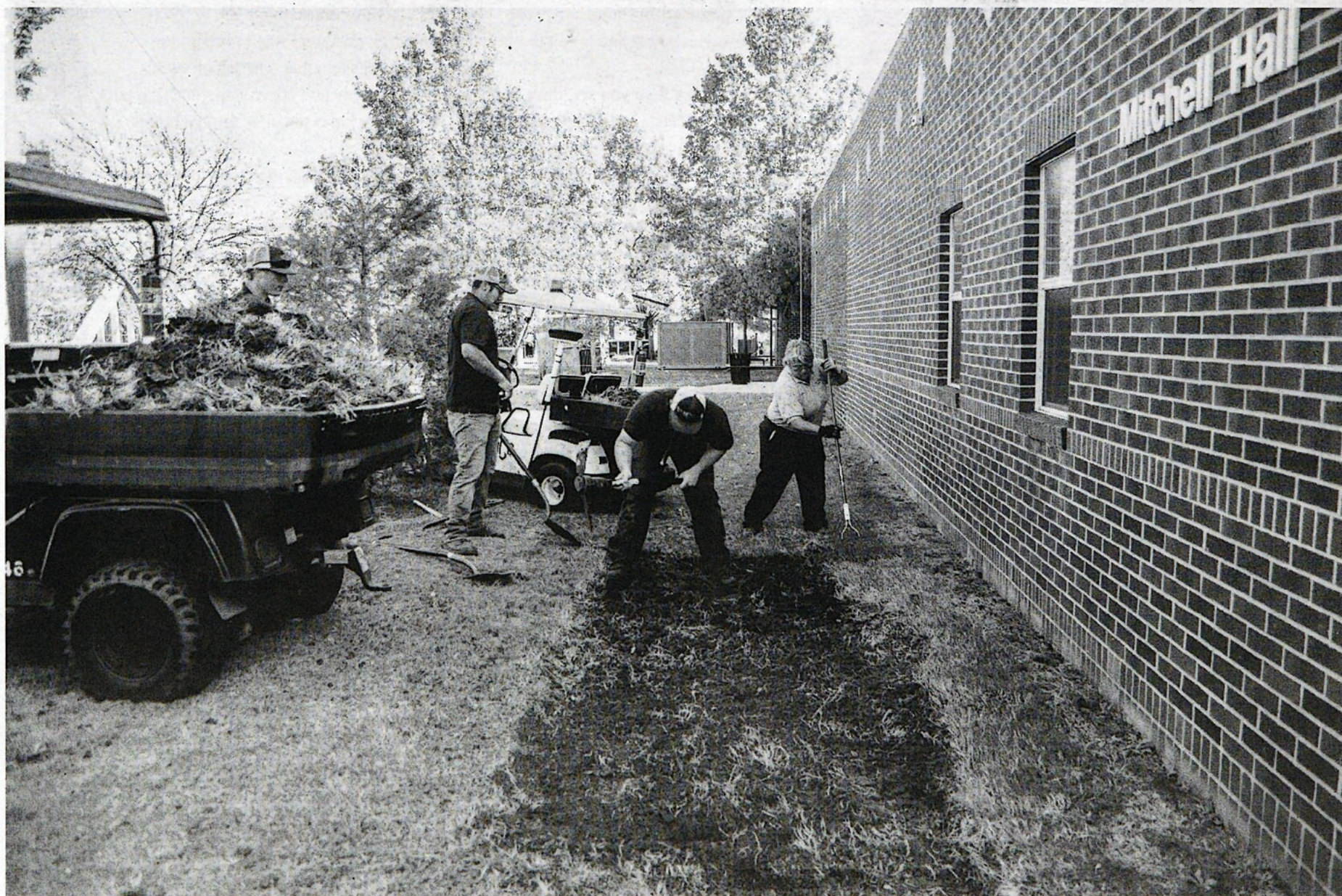
A landscaping crew prepares the ground for the ground breaking ceremony outside of Mitchell Hall. The ceremony was held on November 11 and several UCO administration members were there to kick off the construction process. Photo by Lauren Capraro, The Vista.
