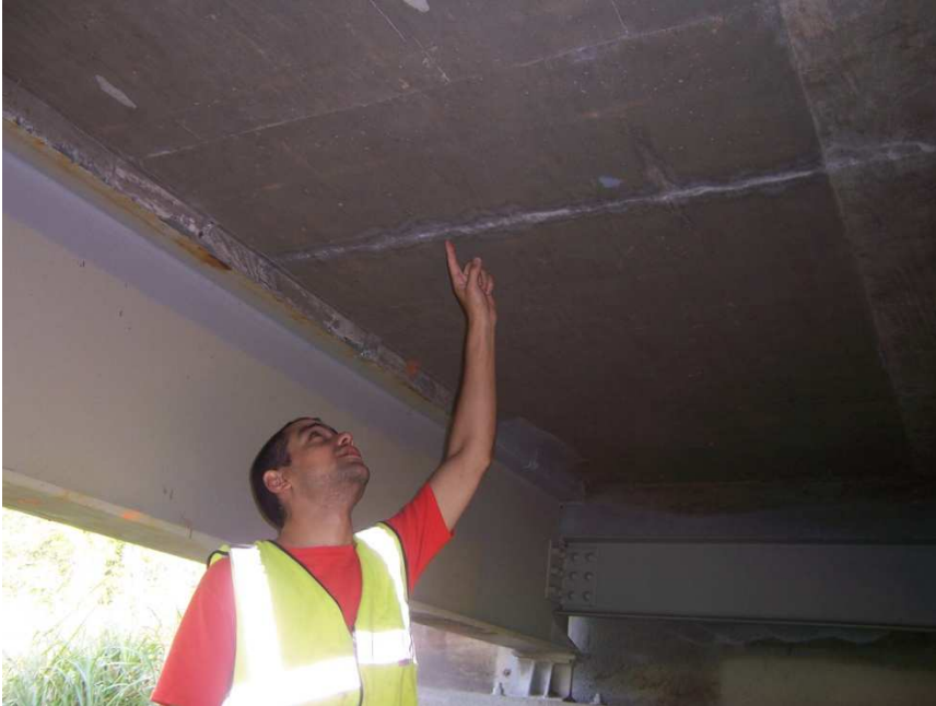
Figure 56 from field investigations, cracking occurs at regular patterns
