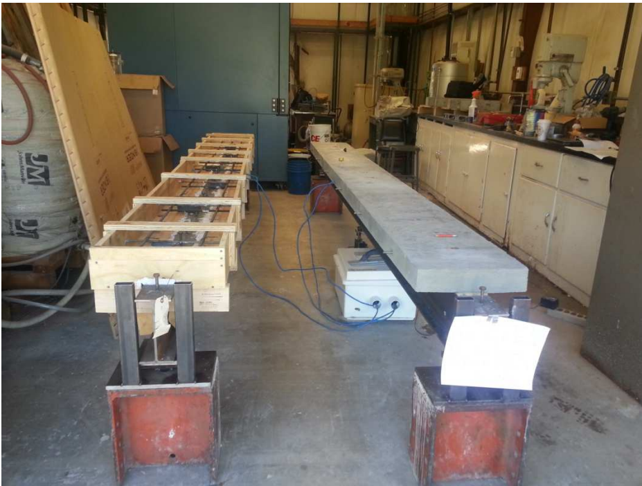
Figure 18 Prototype beam # 1 is cast and beam # 2 is ready to get concrete placed.
