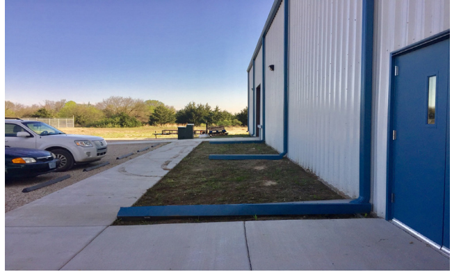
Figure 5. Picture of downspout reconnected to sidewalk (discouraged).
