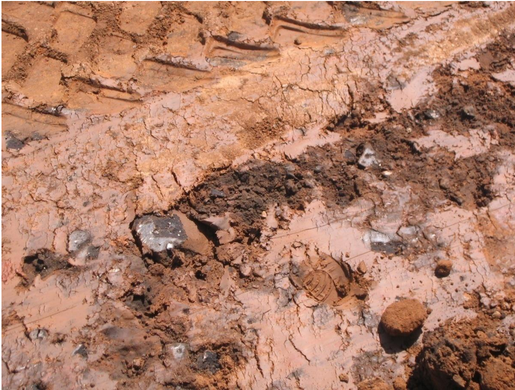
Figure 3-46 Weak Subgrade Soil Encountered during Milling Process
