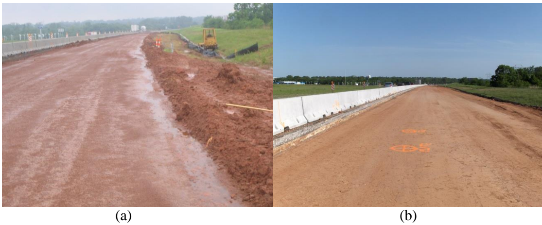
Figure 3-60 Stabilized Subgrade Layer, Facing South (a), After Heavy Raining (b), After Drying
