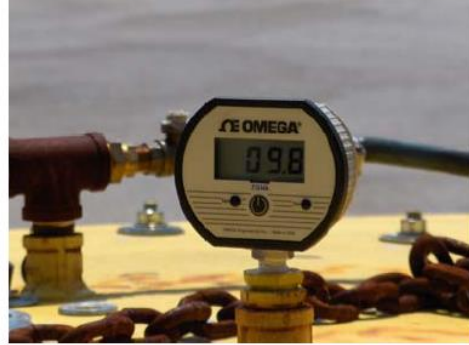
d) External Pressure Gauge on Chamber
