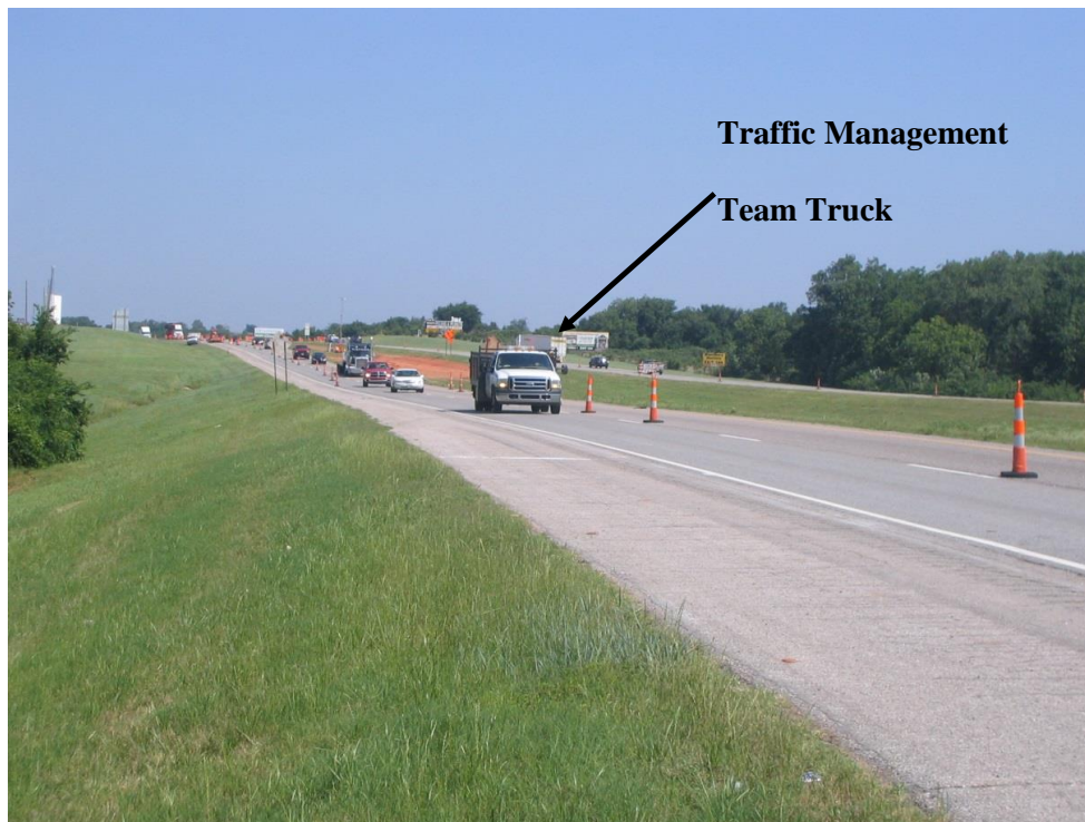
Figure 3-82 Opening of Lane for Traffic
