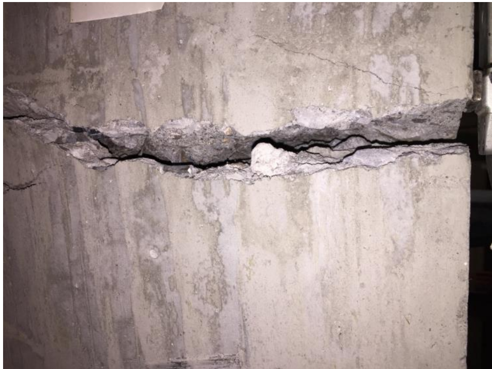
Figure 85. Crack in base concrete on south side from underneath
