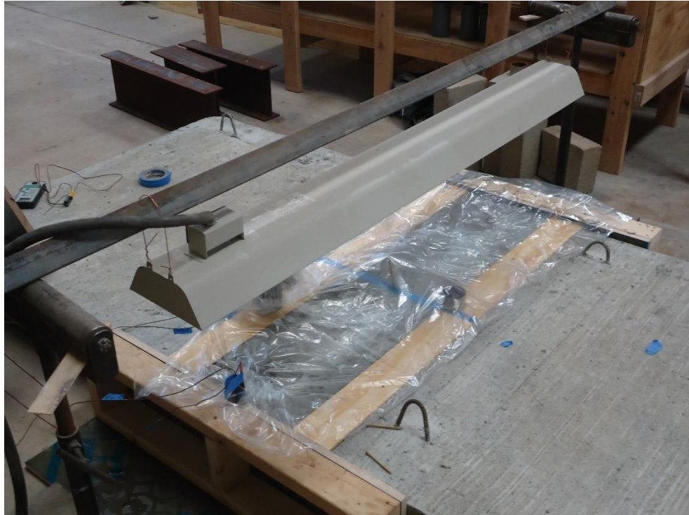
Figure 97. Heat lamp and medium-scale slab with UHPC joint during heat curing process
