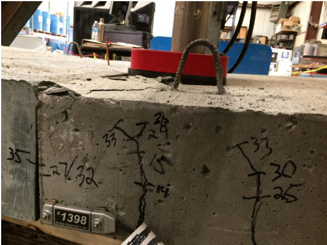
Figure 43. Cracks formed underneath load on south side of slab 1 and concrete crushing at the top compression fiber
