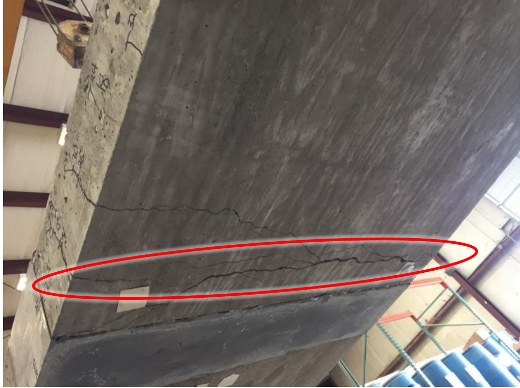
Figure 41. Major cracking underneath load point for slab 1
