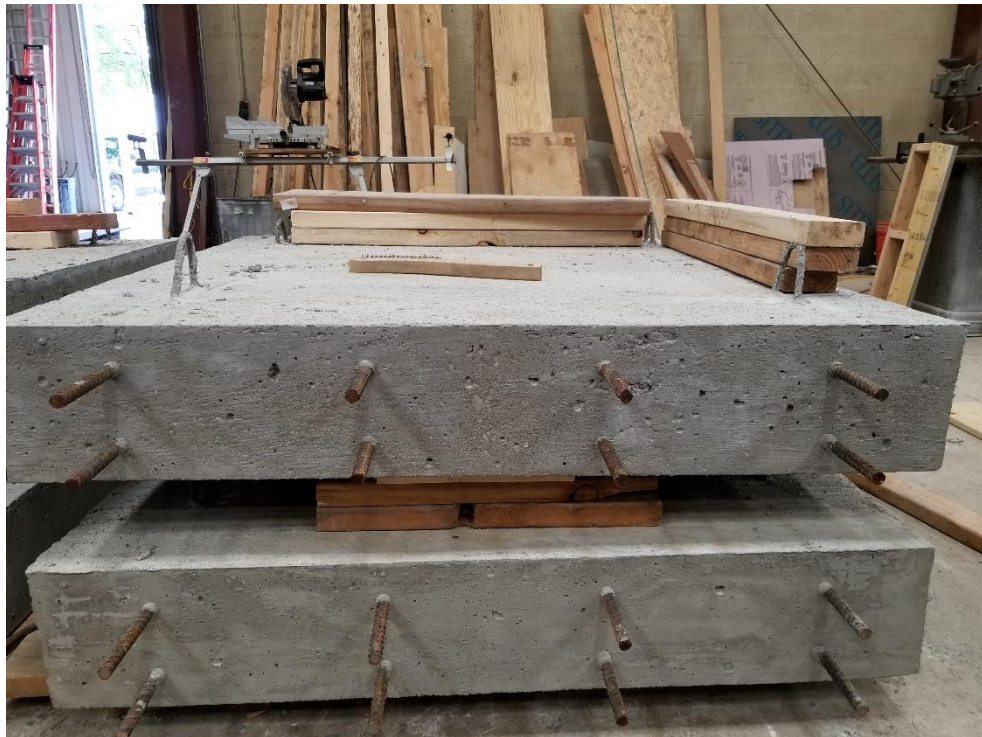
Figure 96. Slab panels with exposed rebar prior to casting of the UHPC joint
