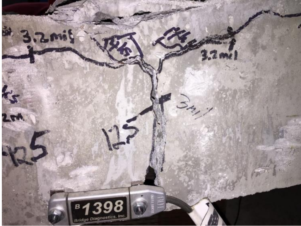
Figure 84. Crack in base concrete on south side and crushing of the top compression fiber after final static loading
