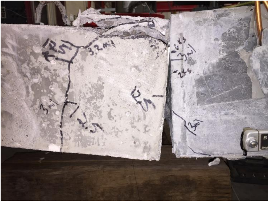
Figure 82. Crack at interface on north side of slab after final static loading and crushing of the top compression fiber in the base concrete
