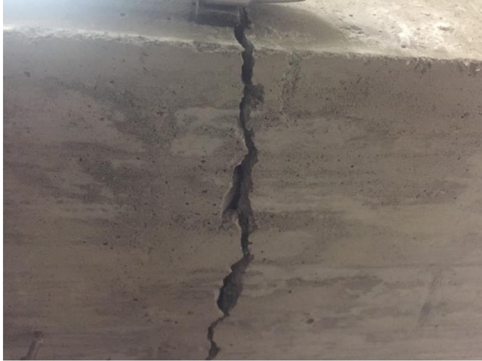
Figure 77. Crack in base concrete on south side after fatigue loading
