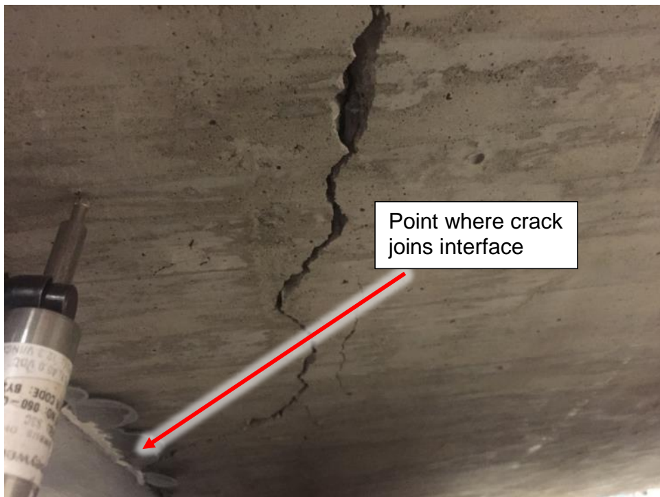
Figure 78. Path of crack underneath slab from base concrete to interface
