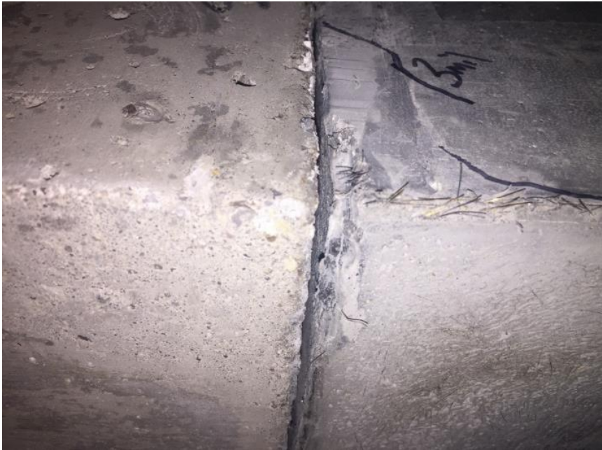
Figure 76. Crack at interface on north side of slab after fatigue loading
