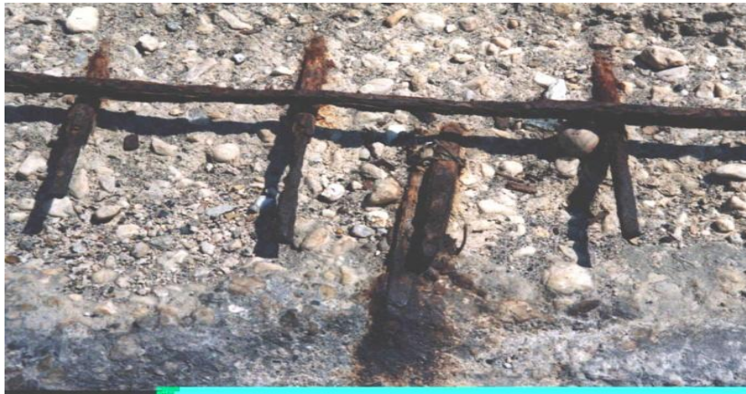
Figure 2.4 Corrosion of reinforced concrete in bridge
