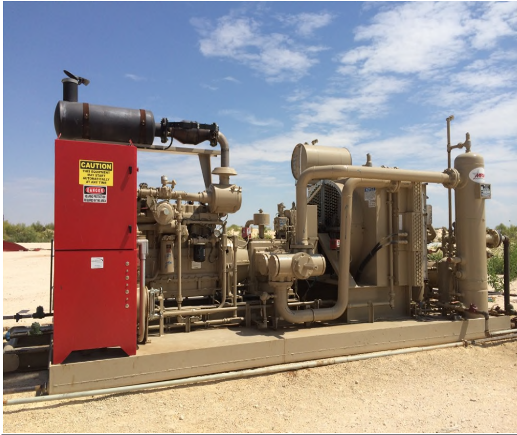
Figure 6.5: High-speed 3-stage compressor, Courtesy of NGSG
