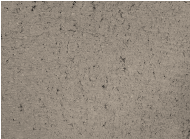
Figure 4-16: Mixture 47 shows poor finishability with high amounts of #16.
