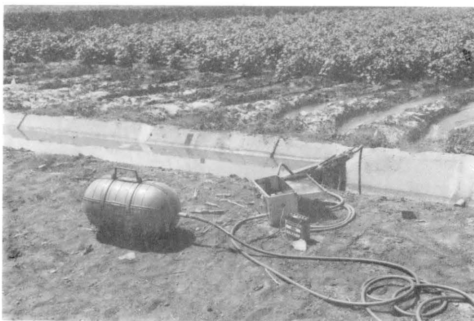
Figure 5. Rotating Gate Control Unit With Air Tank and Battery
