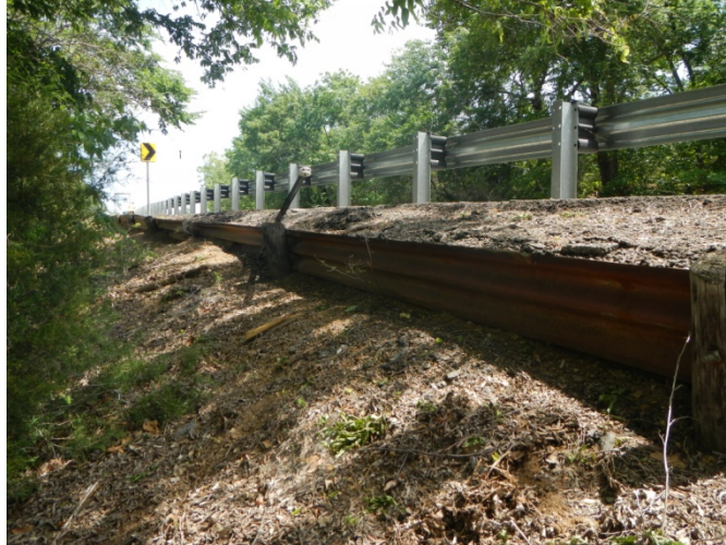
Figure_APX_B 9. Old Guardrail is seen here actually acting as a retaining measure for additional asphalt overlays.
