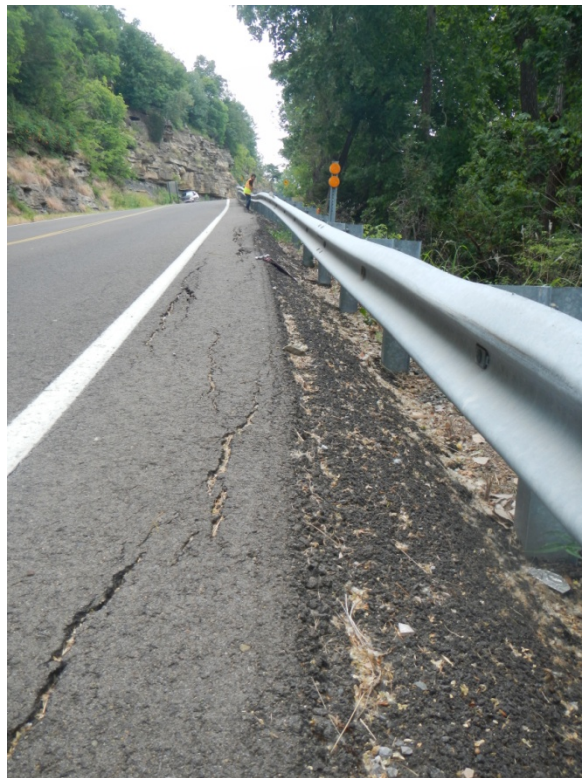
Figure_APX_B 39. Looking south on Route 80 N (away from dam), shoulder cracking is seen, as well as overlay
