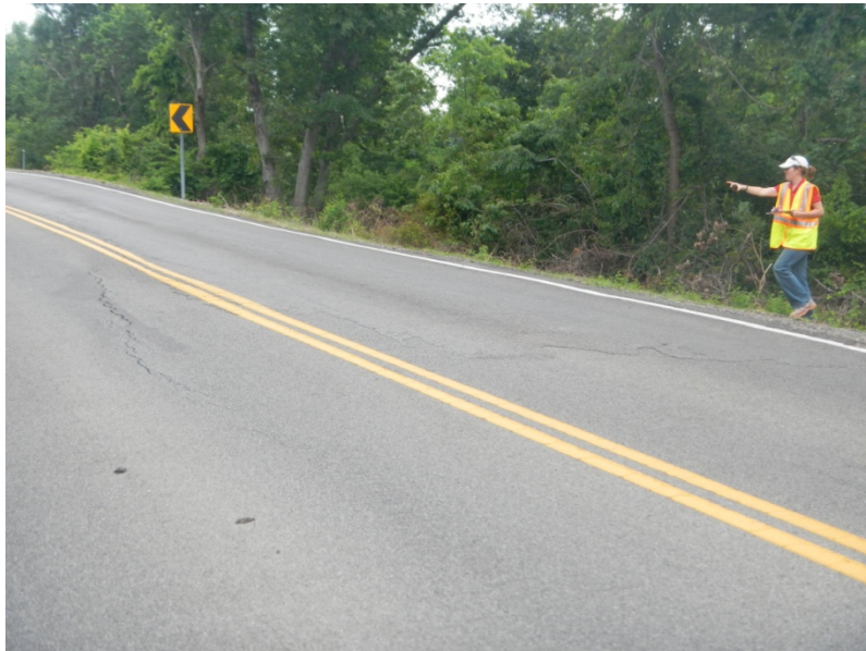
Figure_APX_B 36. West side of Route 10, south side of reflective guardrail, circular cracking is evident. No riprap at toe in this location.
