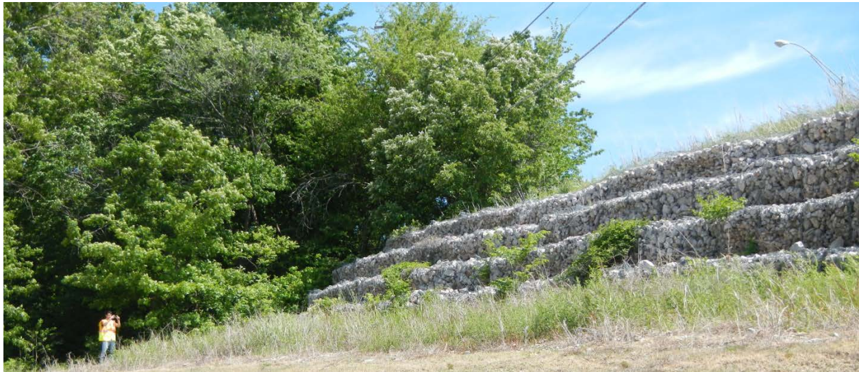
Figure_APX_B 5. Gabion Wall as Retaining Structure.
