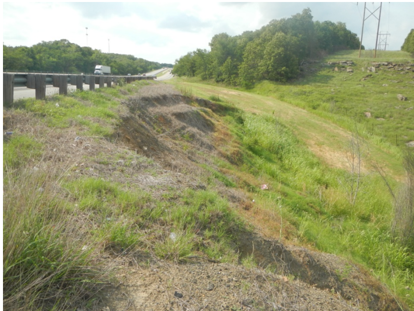
Figure APX_B 40. Route 75, 0.6 miles north of Preston Road, slide area is well defined, toward north end of guardrail, where the natural tree toe support ends.
