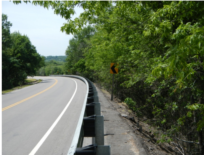
Figure_APX_B 7. Looking west on Route 9. Landslide on the north side of road.
