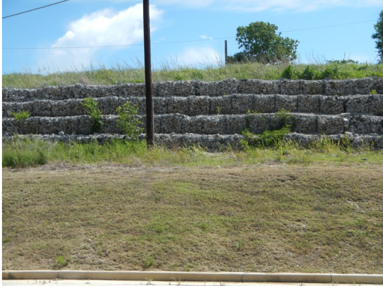
Figure_APX_B 4. Gabion Wall as Retaining Structure.
