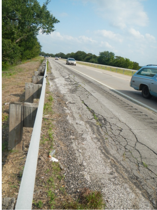
Figure_APX_B 41. Route 75, 0.6 miles north of Preston Road, looking southbound, shoulder cracking is evident.
