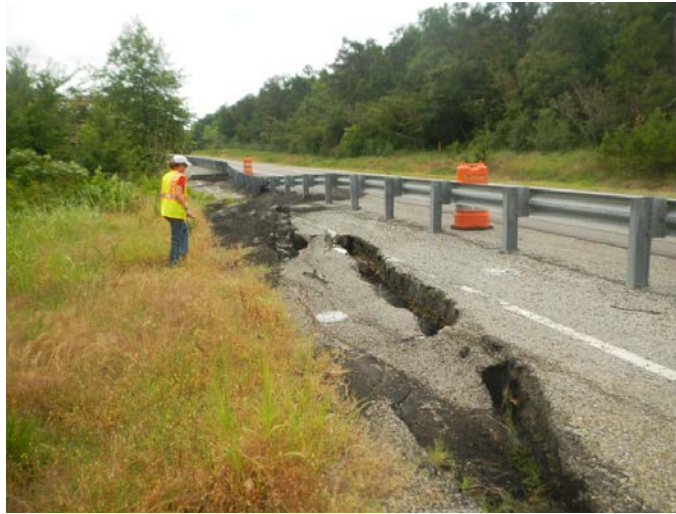
Figure_APX_B 32. Route 2, 4 miles south of junction with Route 31, headscarp in active slide.
