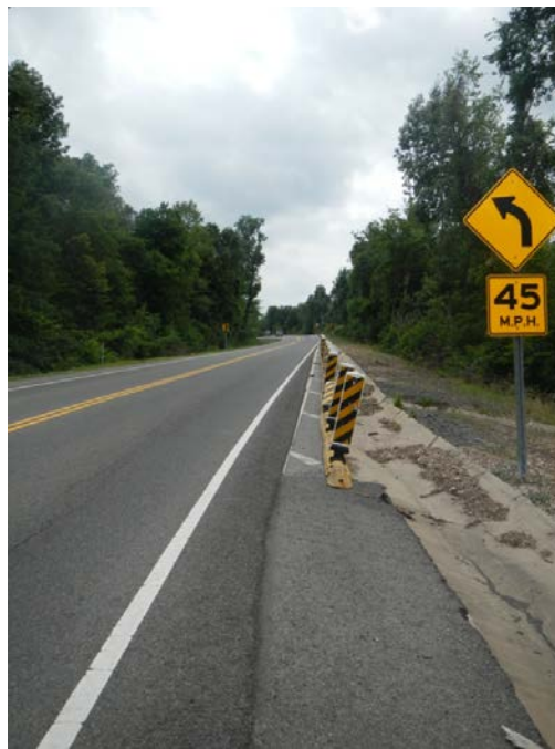
Figure APX_B 34. West side of Route 10, looking south, realignment is evident. Outline of slide is difficult to see.
