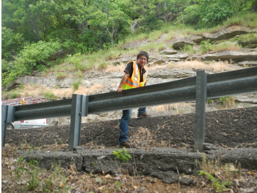
Figure_APX_B 38. Route 80 just south of Fort Gibson Dam, 3' of overlay in middle of slide area.
