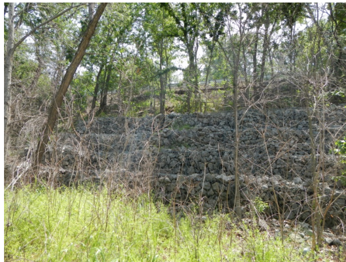
Figure_APX_B 10. 240' long row of Gabion Baskets, stacked 4 high in stair step fashion.
