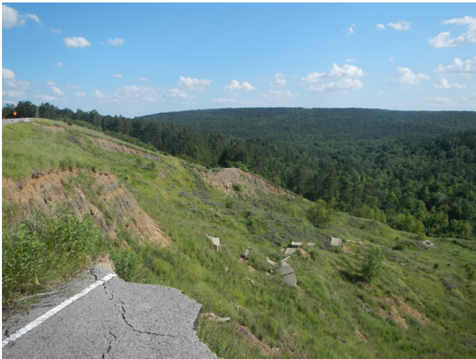
Figure APX_B 25. Photo taken May 9, 2012 standing at the end of destroyed county road.
