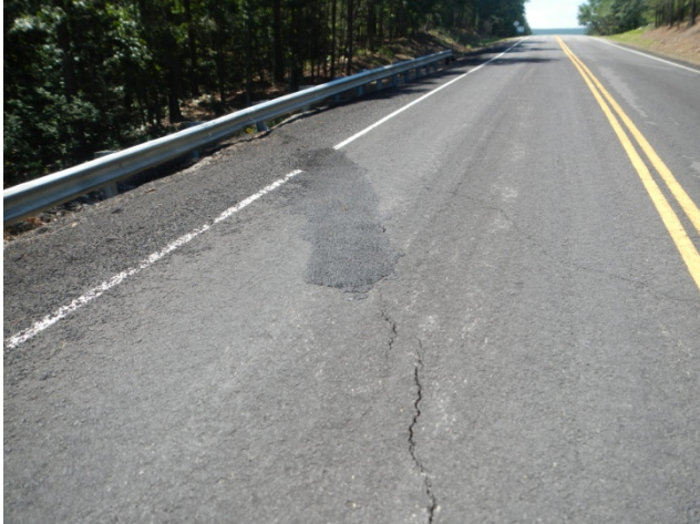
B18. A. Cracking in the road bed.
