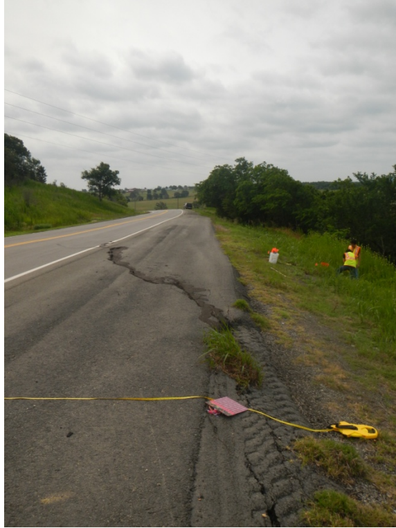
Figure_APX_B 29. Route 9, 1 mile east of Turnpike, road realignment and landslide cracking in new shoulder (old east bound lane) visible.
