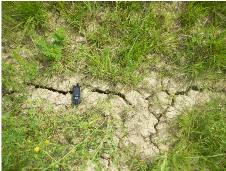
Figure_APX_B 13. Desiccation Cracks all over slope, although water was found only 4 feet below the surface.
