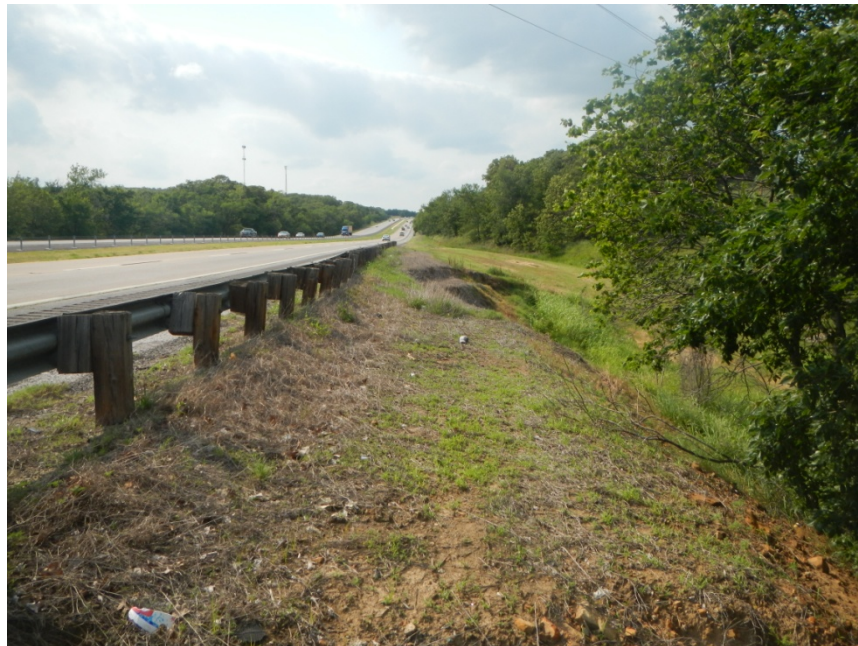
Figure_APX_B 42. Route 75, 0.6 miles north of Preston Road, proximity of headscarp to guardrail. Note end of trees/toe support is where slide occurred.
