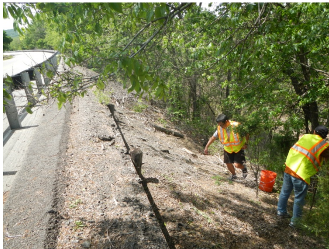
Figure_APX_B 8. Can see old guardrail almost buried down the slope. The road was slightly realigned away from the slope a few years ago, although it is still moving.
