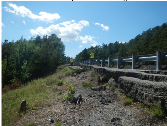
Figure_APX_B 22. Route 271, after Talimena state park Looking north. 3 feet of asphalt overlay visible.
