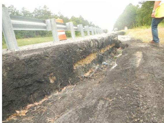
Figure APX B 31. Route 2, 4 miles south of junction with Route 31, pavement overlay depth in active slide.
