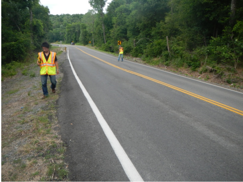
Figure_APX_B 35. West side of Route 10, standing on south side of slide area looking north, new overlay is evident.
