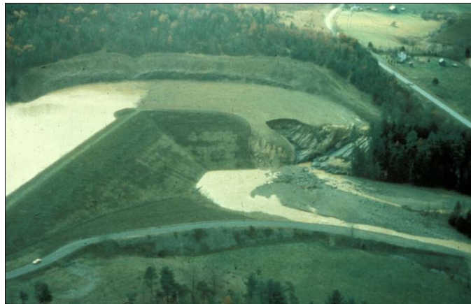
Figure 2.1 Vegetated spillway being eroded. Photo courtesy USDA-ARS HERU
