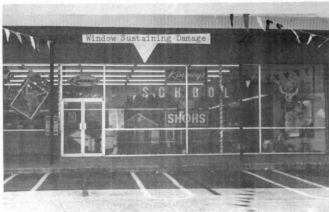
Figure 31. Location of Window Sustaining Damage
