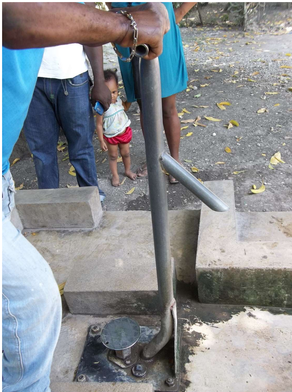
Figure 11: Second broken foot pump
