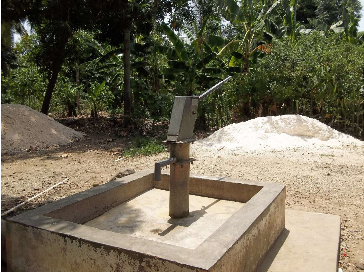
Figure 4: Typical water hand pump
