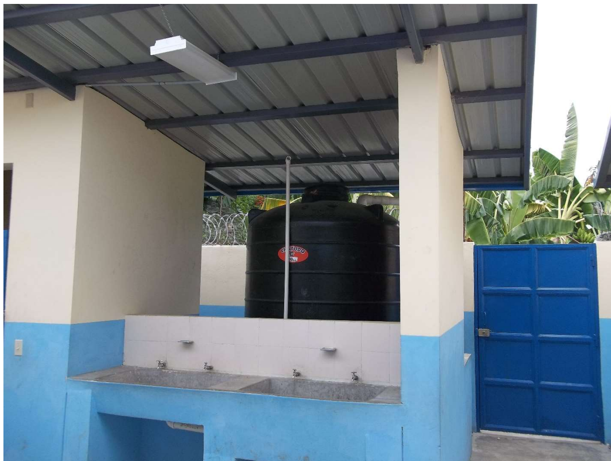
Figure 12: Large storage tanks for water
