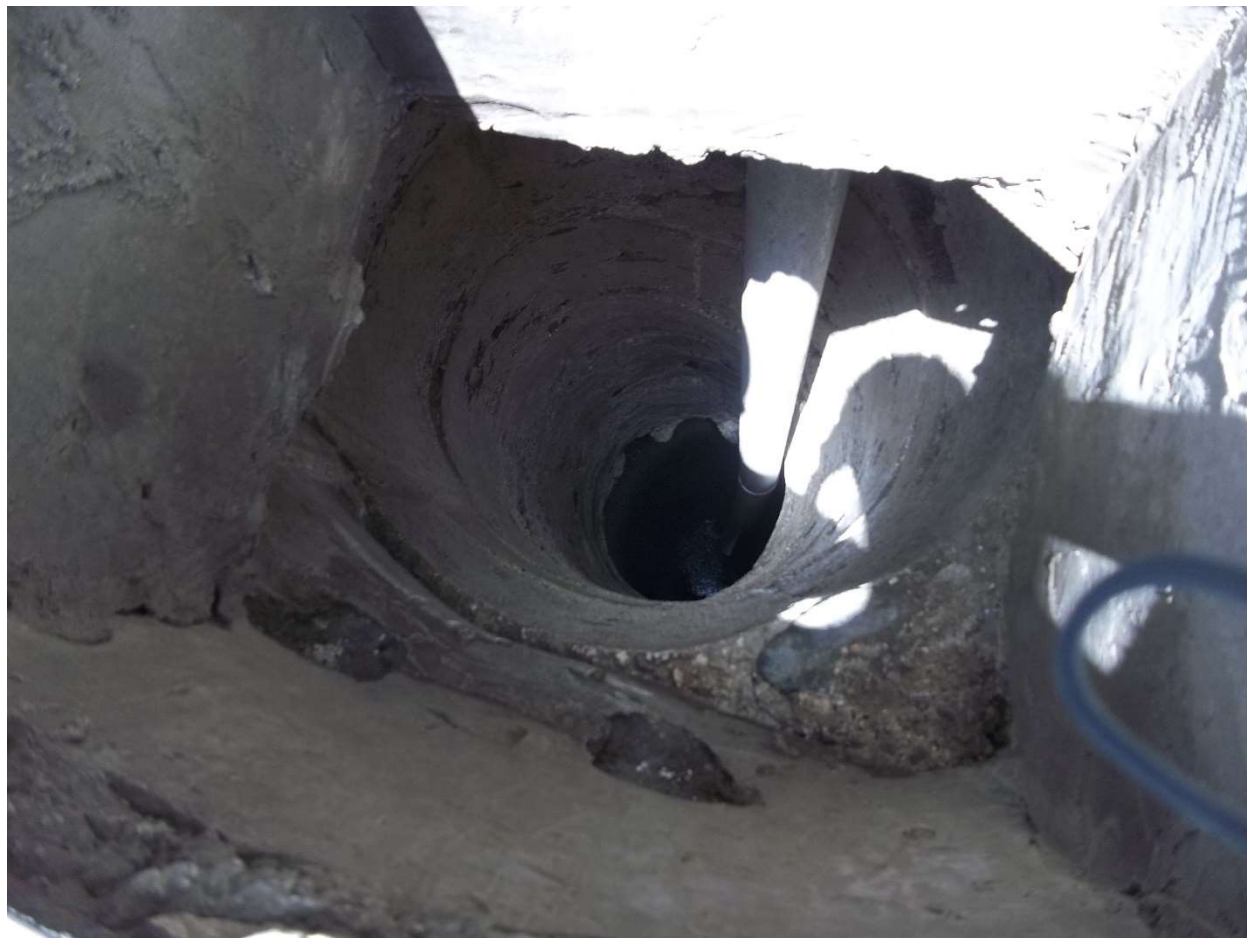
Figure 8: Evidence of insufficient length of pipe
