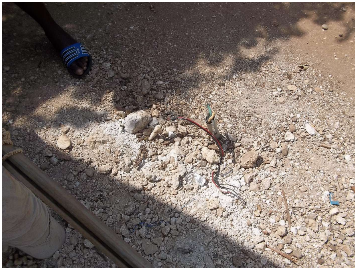
Figure 18: Cut wiring for electric pump
