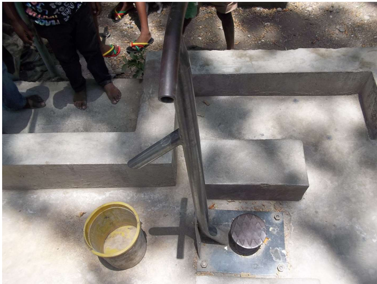
Figure 10: Broken foot pump
