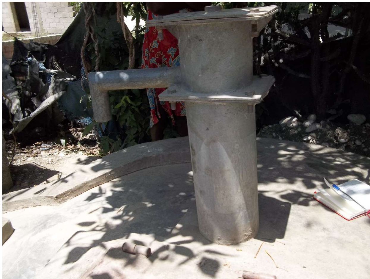
Figure 9: Dry pump due to incorrect installation
