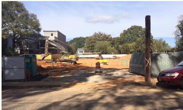
Figure 43 Mauldin Street view of former Stewart Center property, post demolition, 2016. Author photograph.
