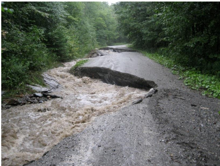
Figure 5.3. Washout on North Road, Middletown Springs, VT during Tropical Storm Irene (28 August 2011). Photo credit: Hilary Solomon, Poultney-
