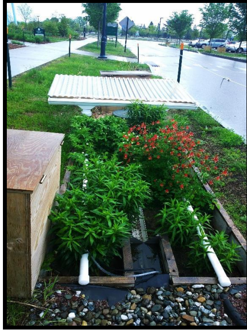
Fig. 1. Bioretention cell with rainpan and PVC precipitation-distribution pipes. The rainpan is installed outside of the cell. Rainwater from the corrugated pan drains into gutters, vertical downspouts, and to pipes that run horizontally along the length of the cell and contains perforations at the bottom to deliver water evenly across the cell.
