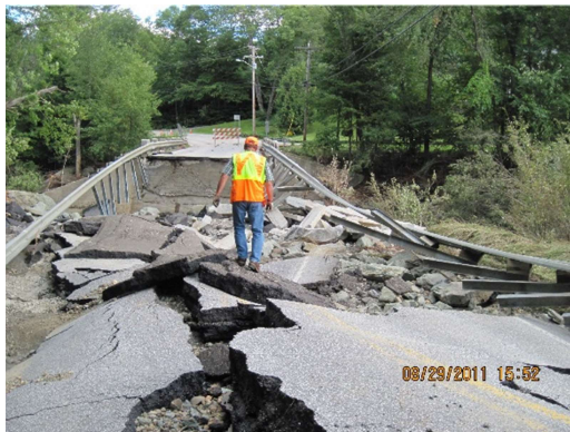
(c) Extensive Channel Flanking Damage
