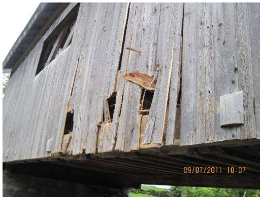
(a) Slight Superstructure Damage
