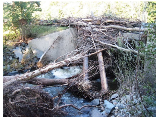
(b) Moderate Debris Damage
