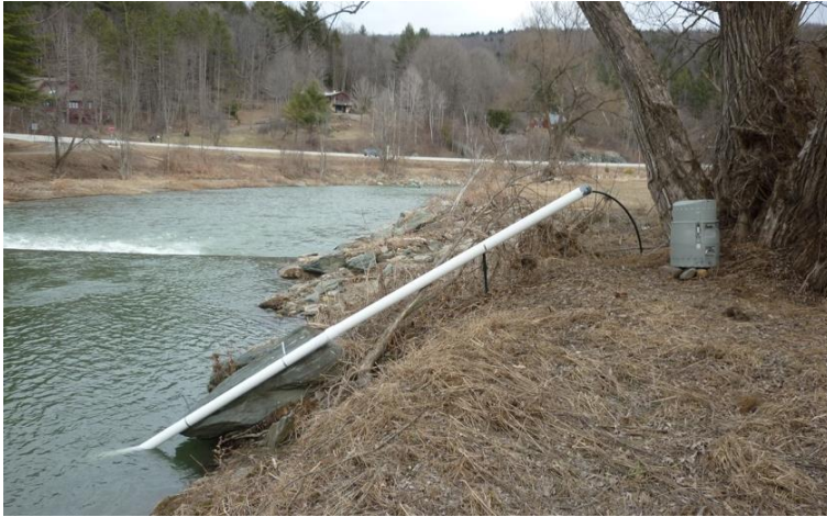
Mad River turbidity sensor installation looking downstream. USGS gauge on opposite bank
