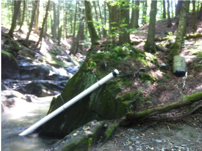
High Bridge Brook turbidity sensor and stage sensor installation looking upstream
