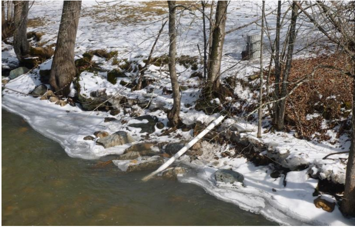
Shepard Brook turbidity sensor and stage sensor installation
